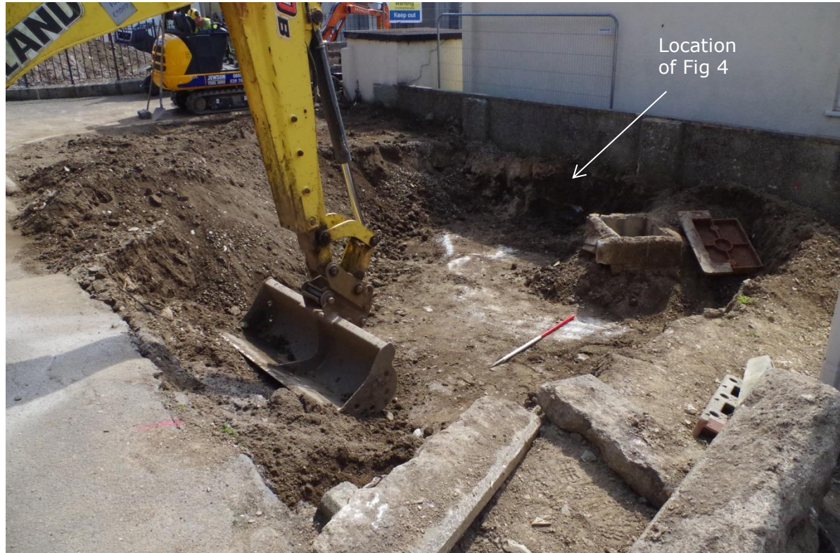
Fig 3 New toilet block – initial excavation. Note the concrete plinth and inspection hatch near ranging rod.
