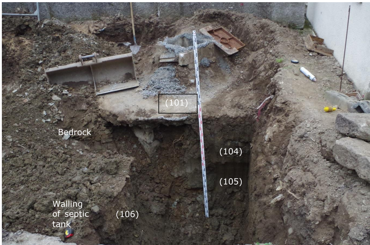
Fig 5 New toilet block – looking to the SW corner of the deeper excavated area. .
