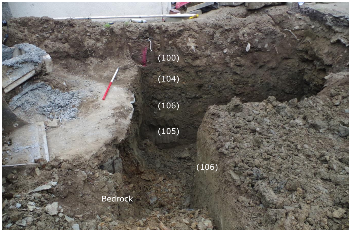
Fig 7 New toilet block - looking to the E facing section in the SW corner of the deeper excavated area.
