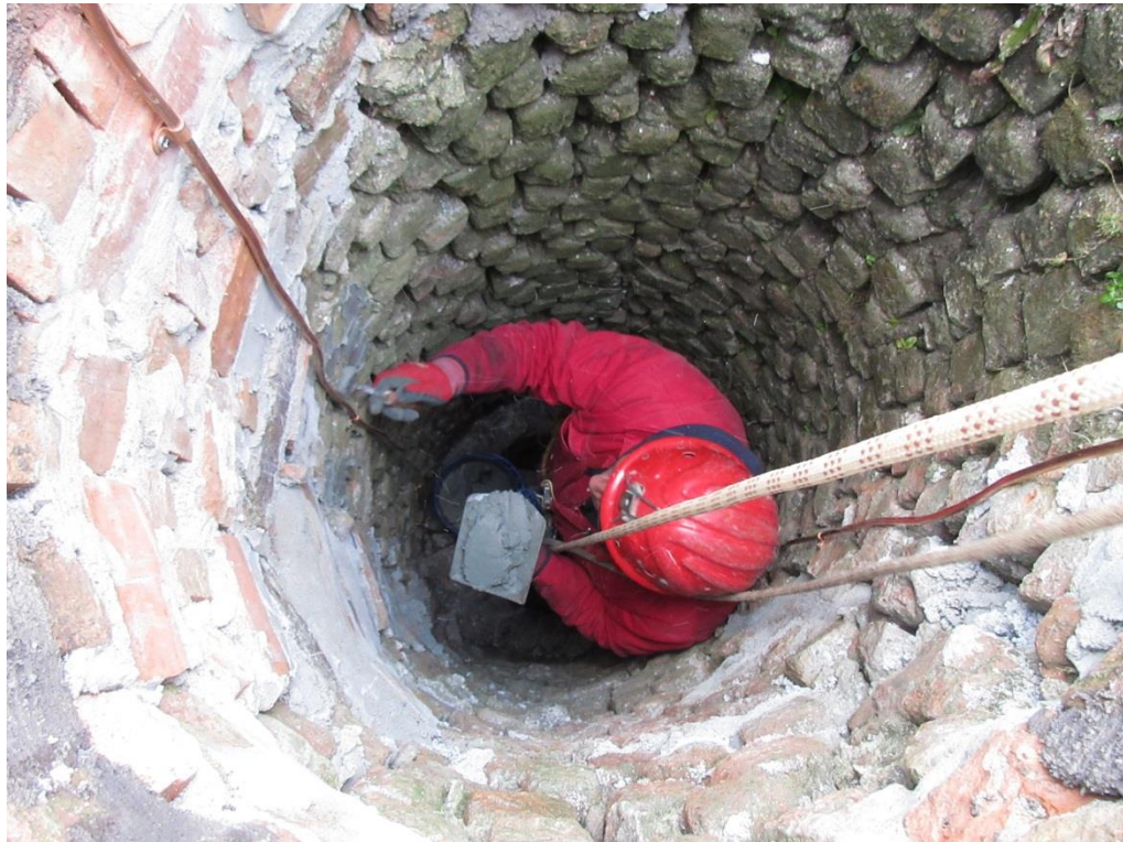
Fig 17. Filling the inner faces of the brickwork joints, which had lost most of their original pointing mortar.
