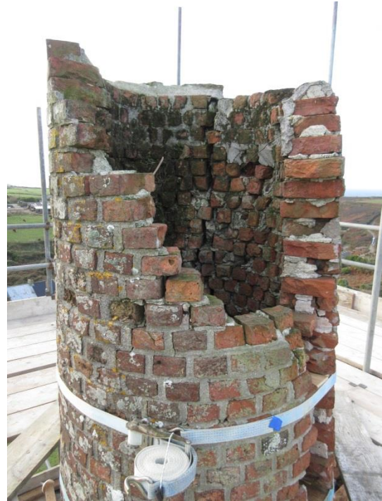
Fig 4. The top of the chimney, ratchet strapped to secure it at an early stage in the works.
