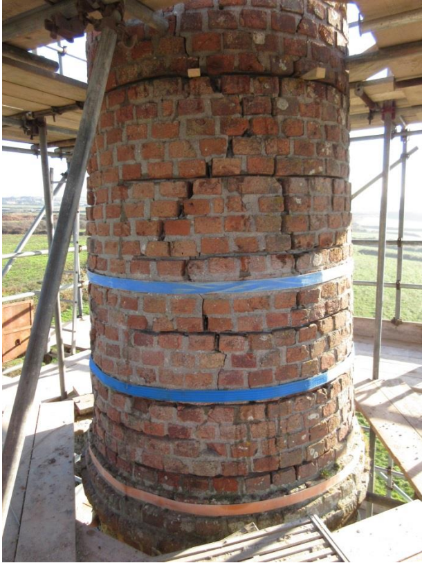
Fig 13. Brick joints cut out across the southern cracks in preparation for the installation of the helicoil bedjoint reinforcement.
