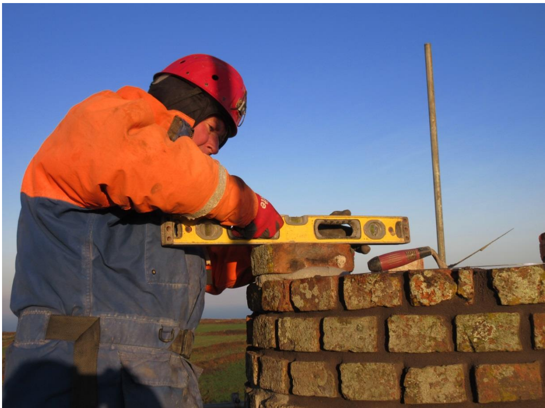
Fig 10. The original brickwork courses were far from level. Not so their replacements.
