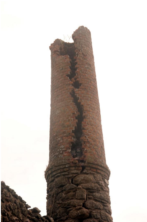
Fig 3. The chimney shortly after the lightning strike.
