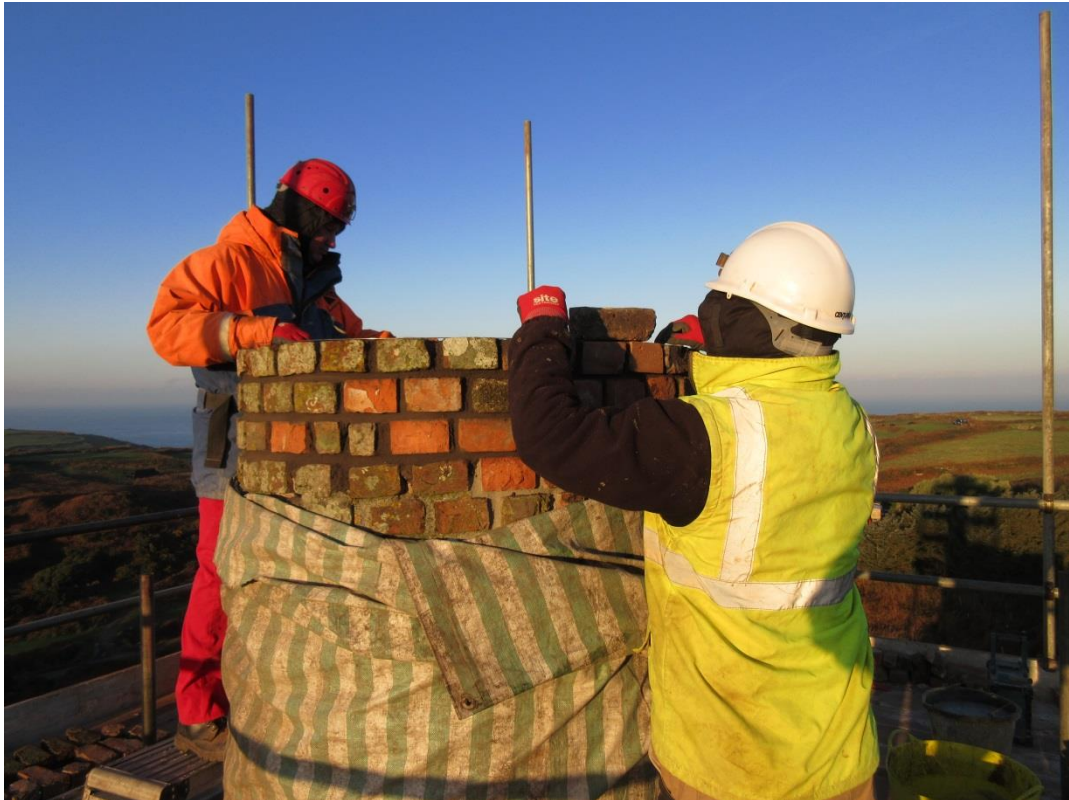
Fig 9. Rebuilding the chimney brickwork. The tarpaulin was used to protect the mortar from the effects of the winter weather.
