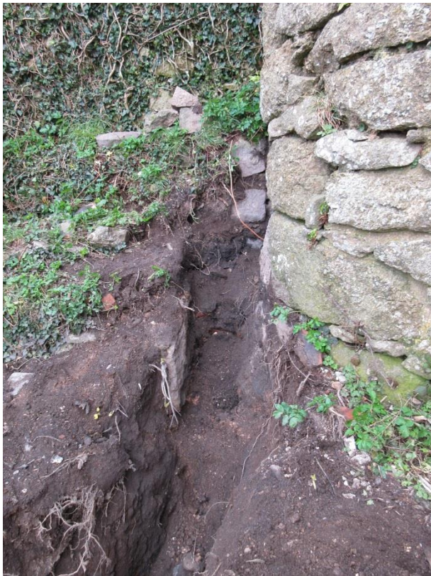
Fig 20. The trench excavated for the earth protection system showing the doorway into the flue and flue opening in the chimney.
