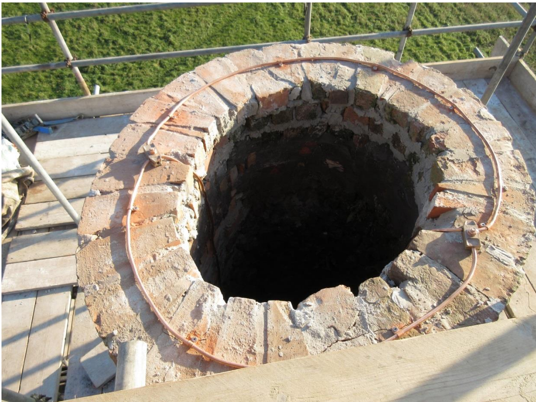
Fig 12. The lightning protection crown ring and twin down tapes.
