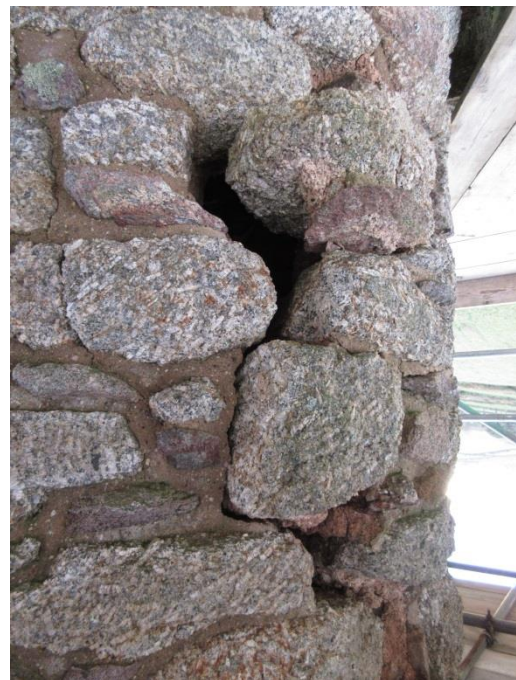
Fig 6. The displaced upper section of the stonework below the drip ring.
