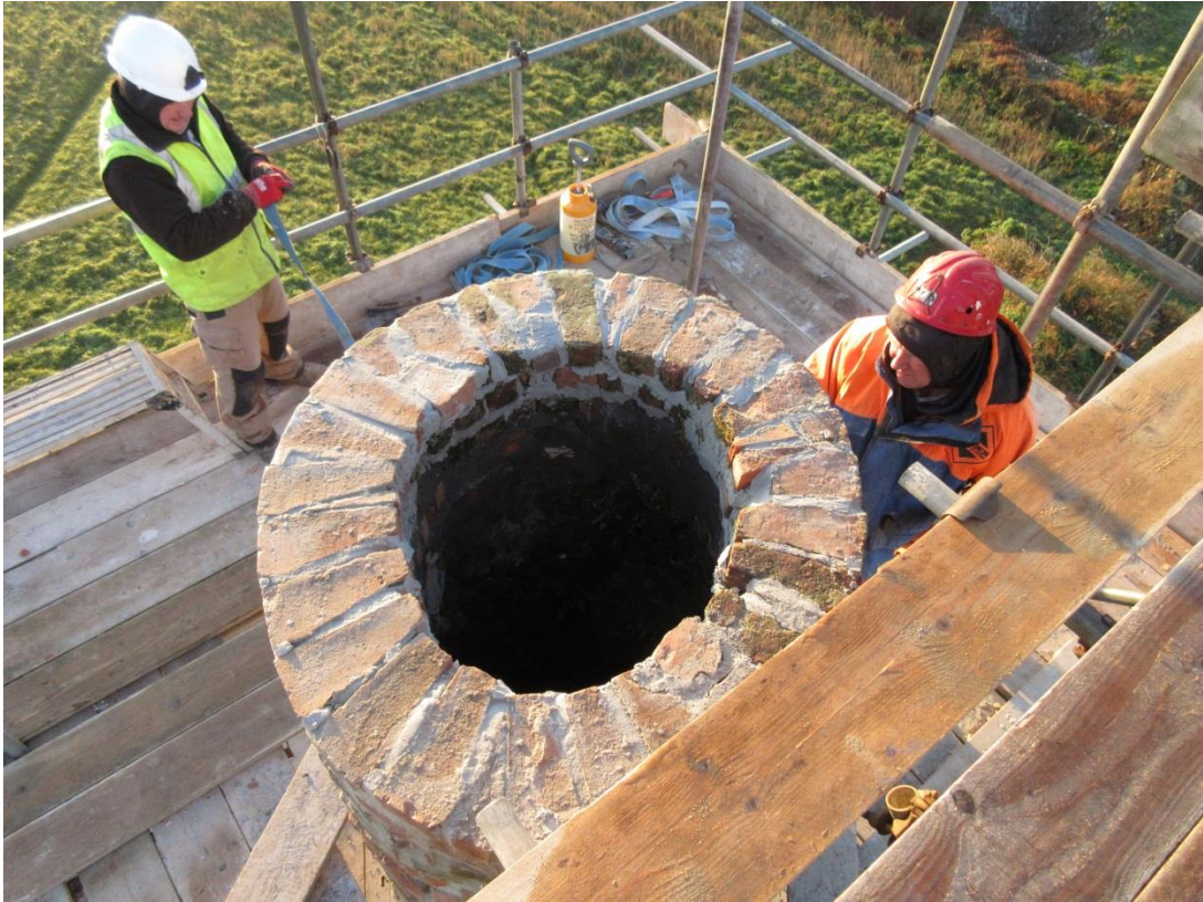
Fig 11. As can be seen the chimney was far from circular in plan, partly as a result of the lightning damage.
