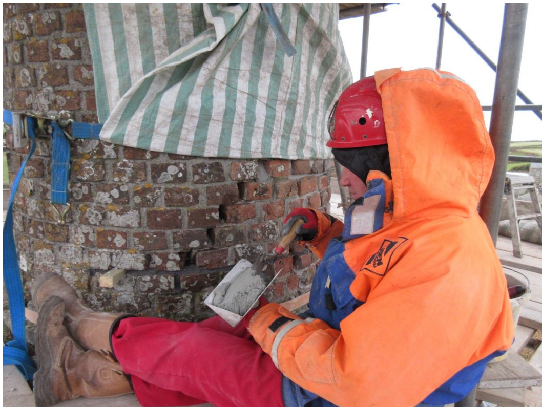
Fig 15. Repointing a stepped crack near the base of the chimney brickwork. The open vertical joints were infilled with brick gallets.
