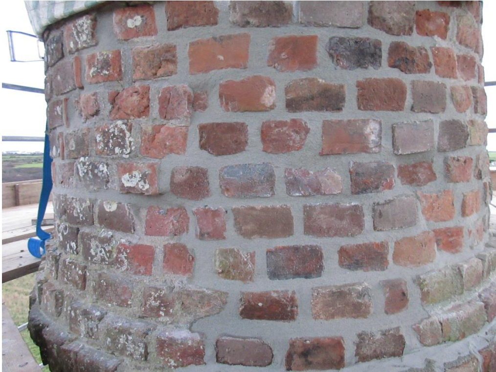
Fig 16. The lower section of the repaired brickwork at the location of the original major cracks. The mortar had yet to be tamped to bring up its texture.
