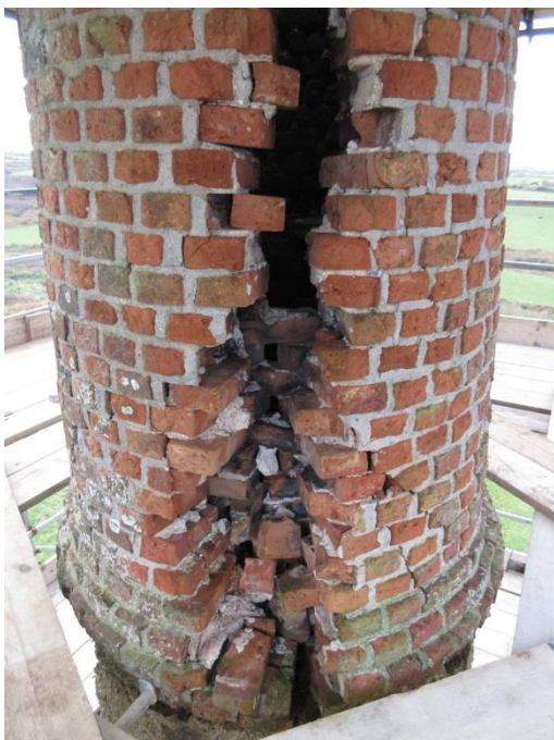
Fig 5. The unzipped lower section of brickwork and drip ring.
