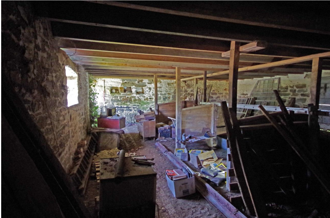
Figure 65 North-west Range - stalls within later cow-house in ground floor of central block [21].
