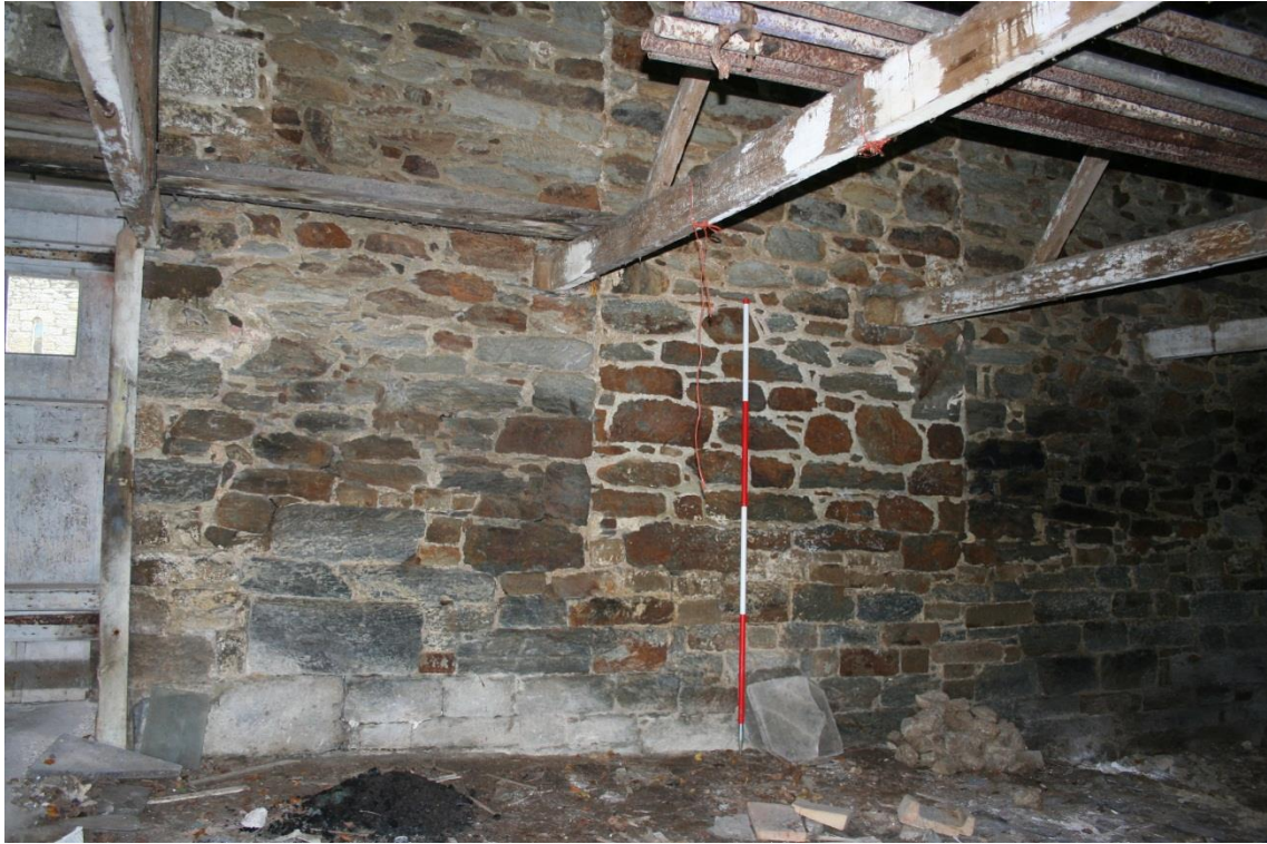
Figure 29 Rear wall of the Stables Range – viewed from inside room [10] of the Farmyard Range; old doorway blocked before lean-to roof of Farmyard Range was added, and masonry underpinning inserted at base of the wall to deal with change of level.
