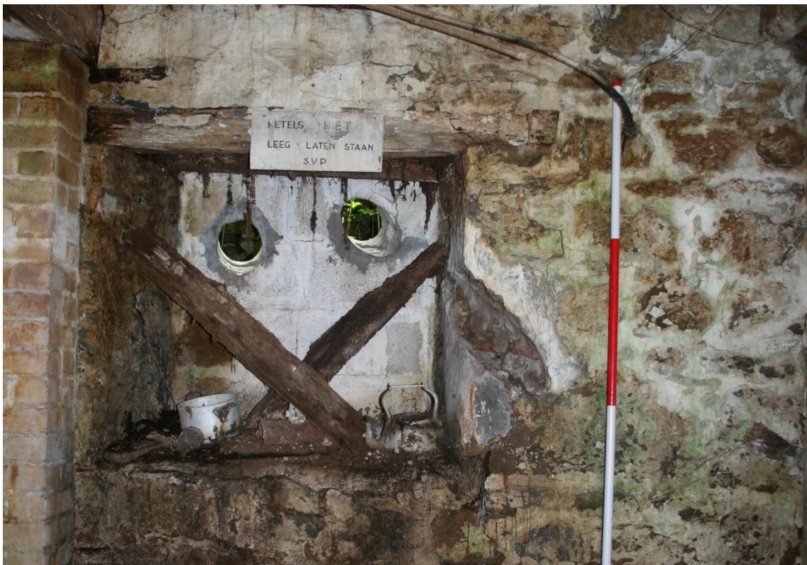
Figure 40 South-west Range – the north-west ground floor room space of the barn [24], with Dutch painted sign and traces of removed stove pipes.
