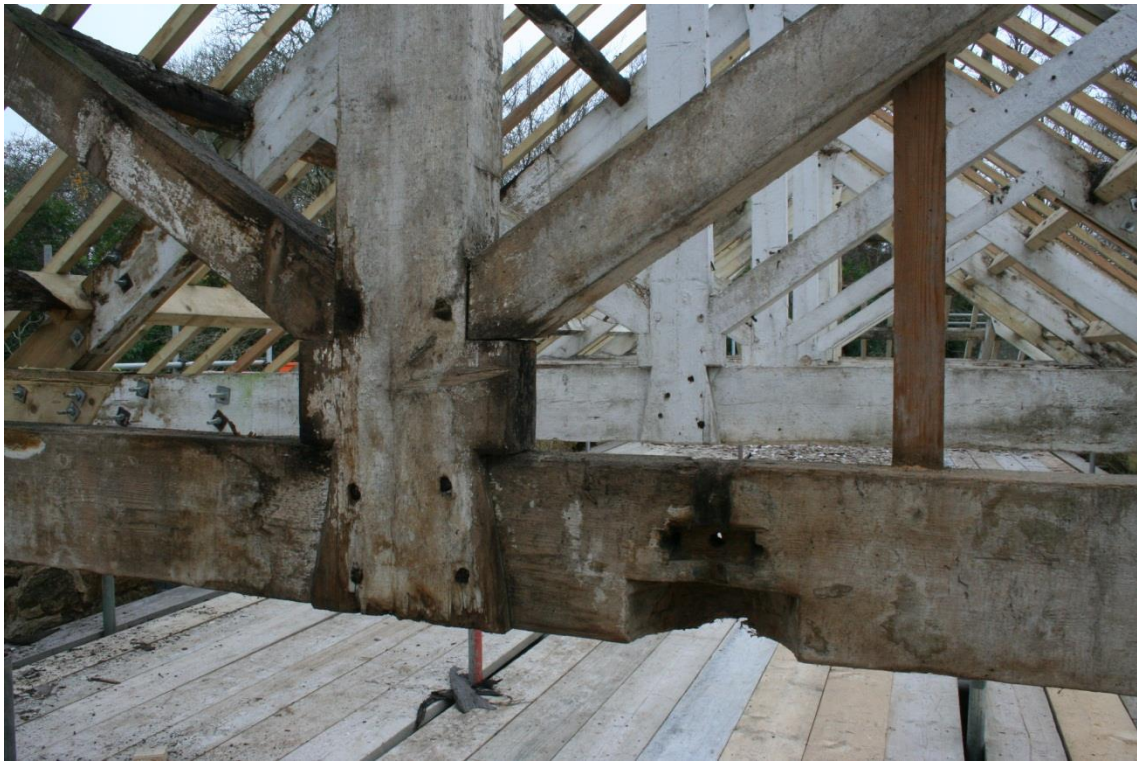
Figure 47 South-west Range - detail of a king post roof truss. Note also the cut-out for a machinery bearing to the right.
