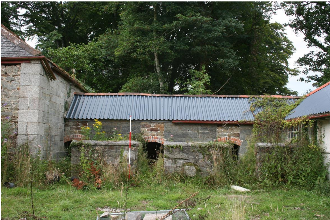
Figure 14 North-west Range – farmyard elevation of the three pigsties at the north-east end [19].
