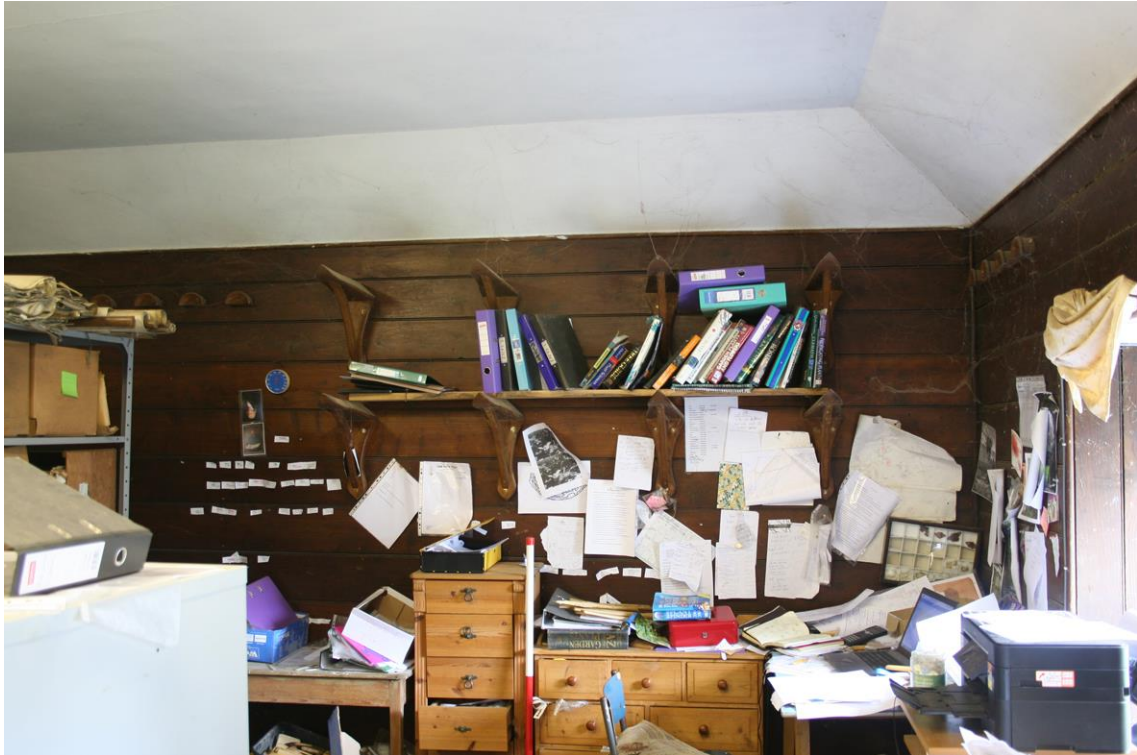
Figure 27 Stables Range – interior of former first floor tack room [8] with saddle rests visible on panelled wall.
