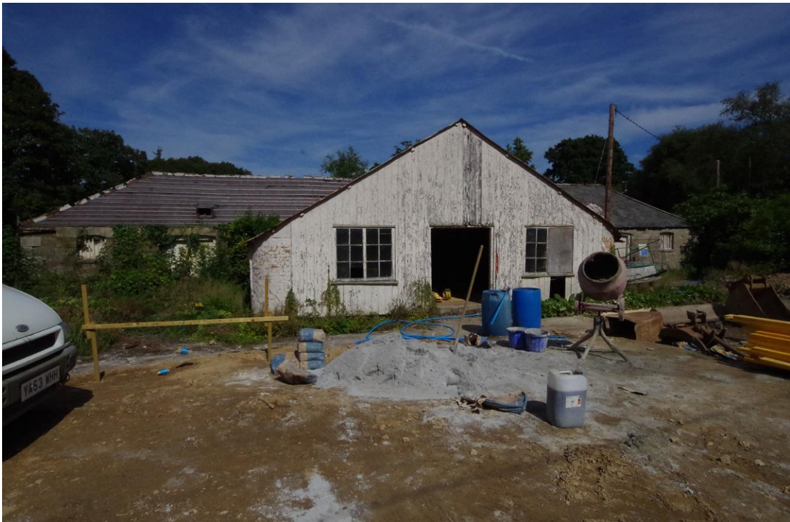
Figure 36 South-west Range – the rickyard elevation with the loft over the horse-engine house (centre).
