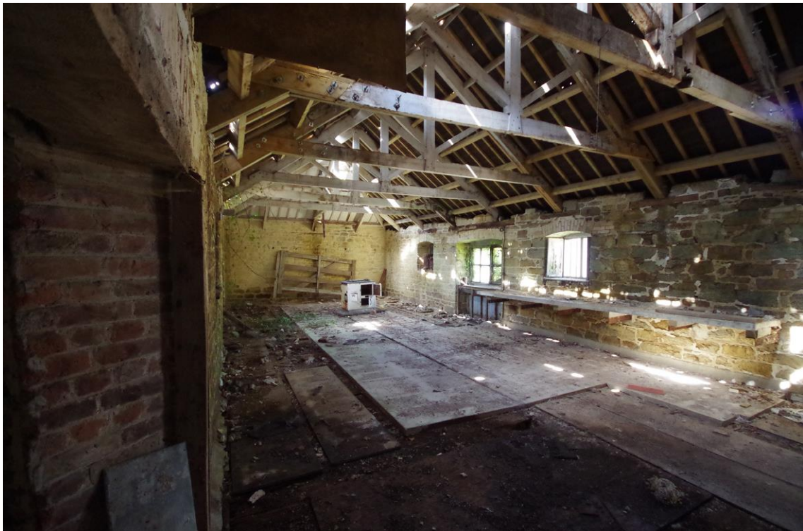
Figure 44 South-west Range – first floor, north-west room space [31] with roof trusses showing recent repair and damage to roof covering visible.
