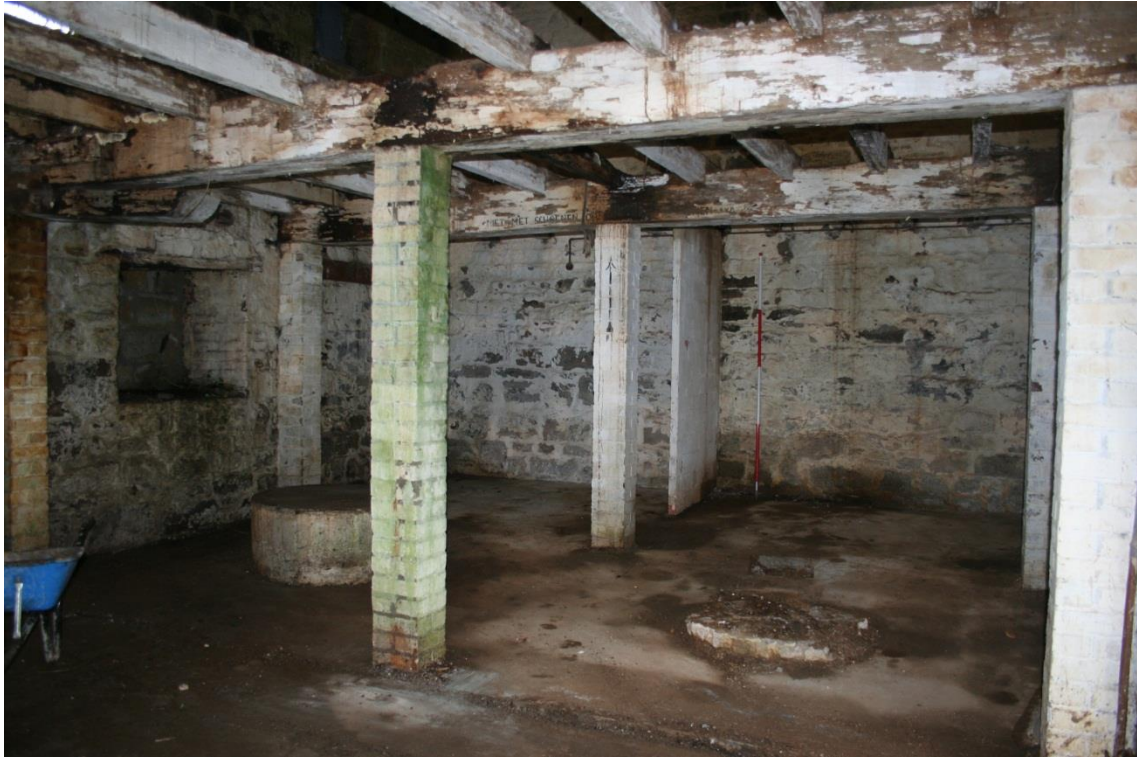
Figure 39 South-west Range – the north-west ground floor room space of the barn [24], with later adaptation in the Second World War.
