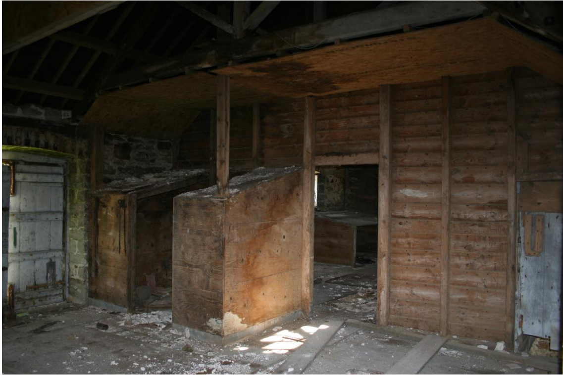
Figure 45 South-west Range – first floor, north-west room space [31], grain bin, partition wall with doorway to south-eastern part [29]/[30] and chute leading to ground floor (right).
