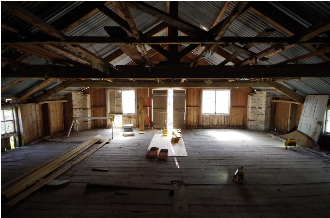
Figure 54 South-west Range – looking south-west to the rear wall of the upper floor extension to the horse-engine house [33].
