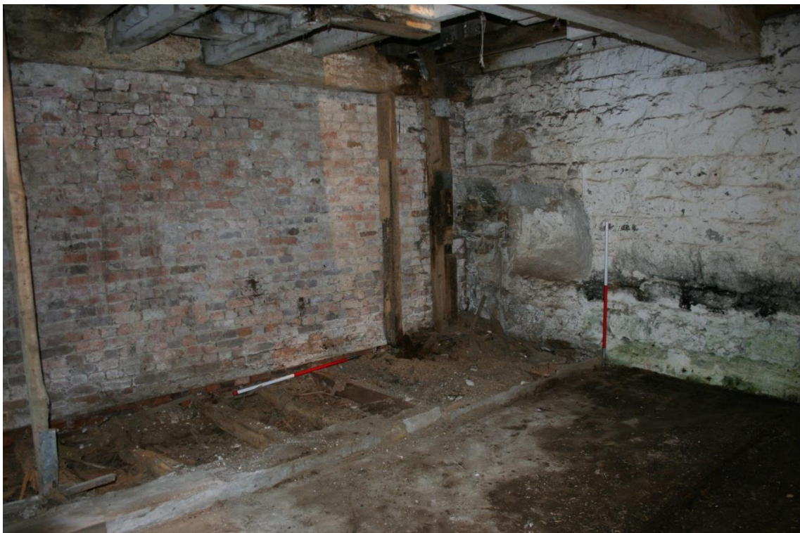
Figure 42 South-west Range – ground floor, central room space of barn [25] showing gear recesses (right of centre), inserted brick wall and raised floor level.
