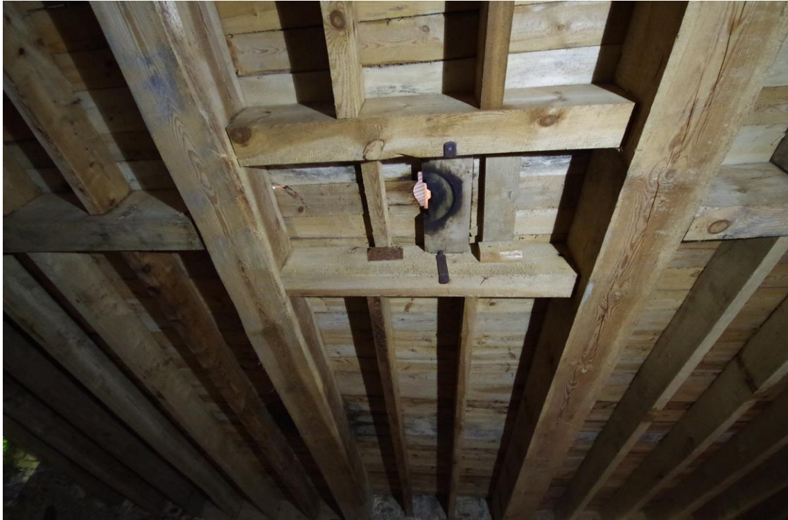
Figure 53 South-west Range - horse engine [32] upper bearing location, timberwork and added upper floor.
