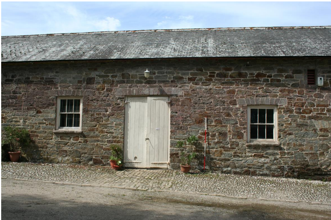
Figure 22 Stables Range - middle part of the range showing later principal doorway and windows. Note the blocked slit ventilator between the scale pole and the RH window.
