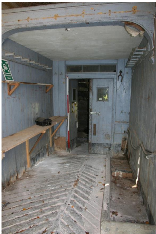
Figure 26 Stables Range – entrance corridor [4], showing details of woodwork. Although they were originally built as separate entities this corridor now links the stables to the Farmyard Range.
