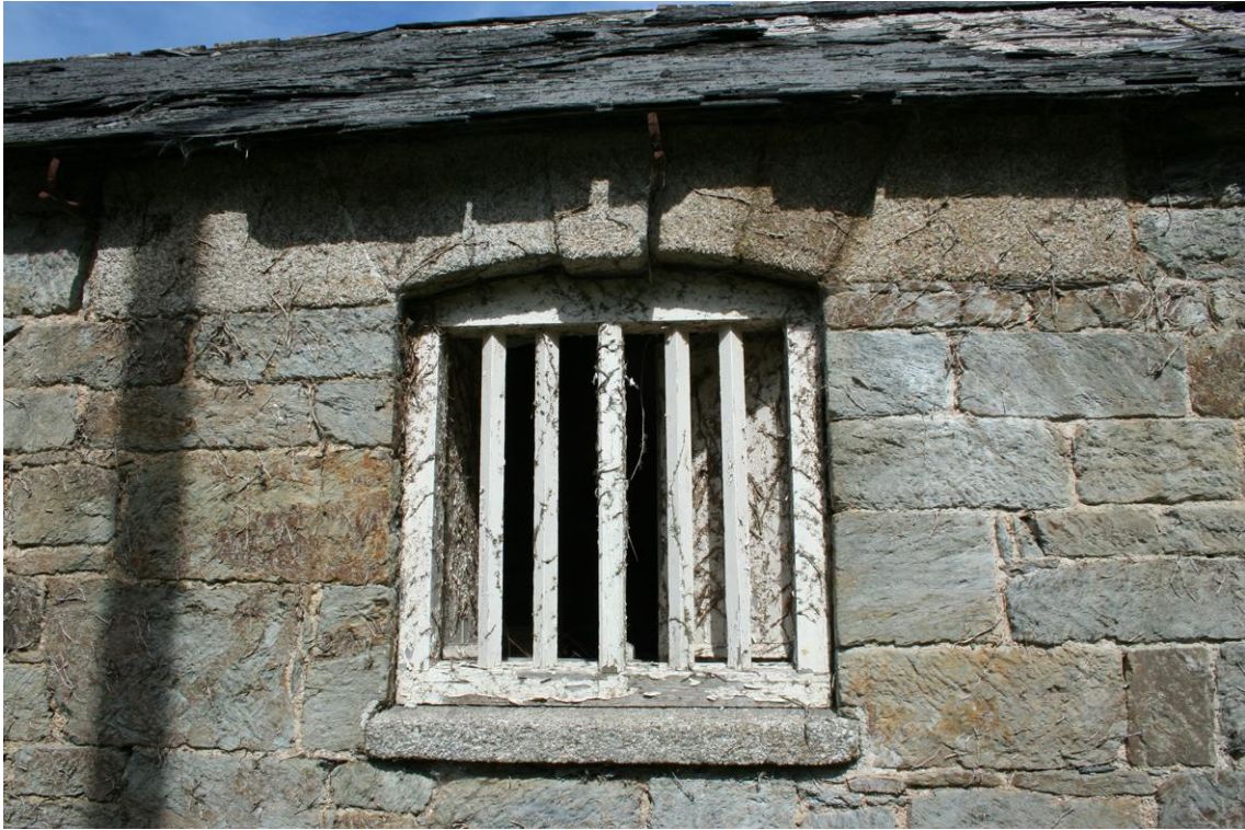
Figure 37 South-west Range – rickyard elevation, first floor; masonry detail of wall and window opening with the wood ventilators and internal shutters.
