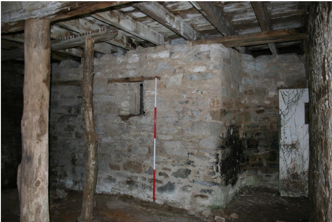
Figure 38 South-west Range - subdividing wall in the ground floor at the south-east end of the range [28].
