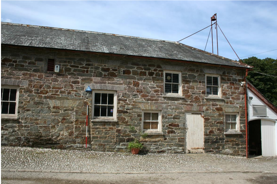
Figure 21 Stables Range - south-east elevation of the lower end of the stables with garage/game larder to right. Blocked ground floor and first floor windows indicate the upper floor once extended further left. Note also the bell on the roof of the range.
