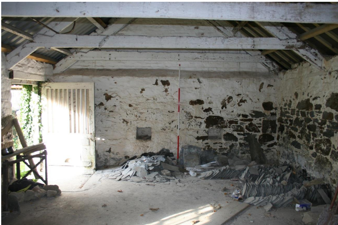
Figure 60 North-east Range - interior of room [15] showing recesses 'keeping places' in dividing wall and original feed passage door to left.
