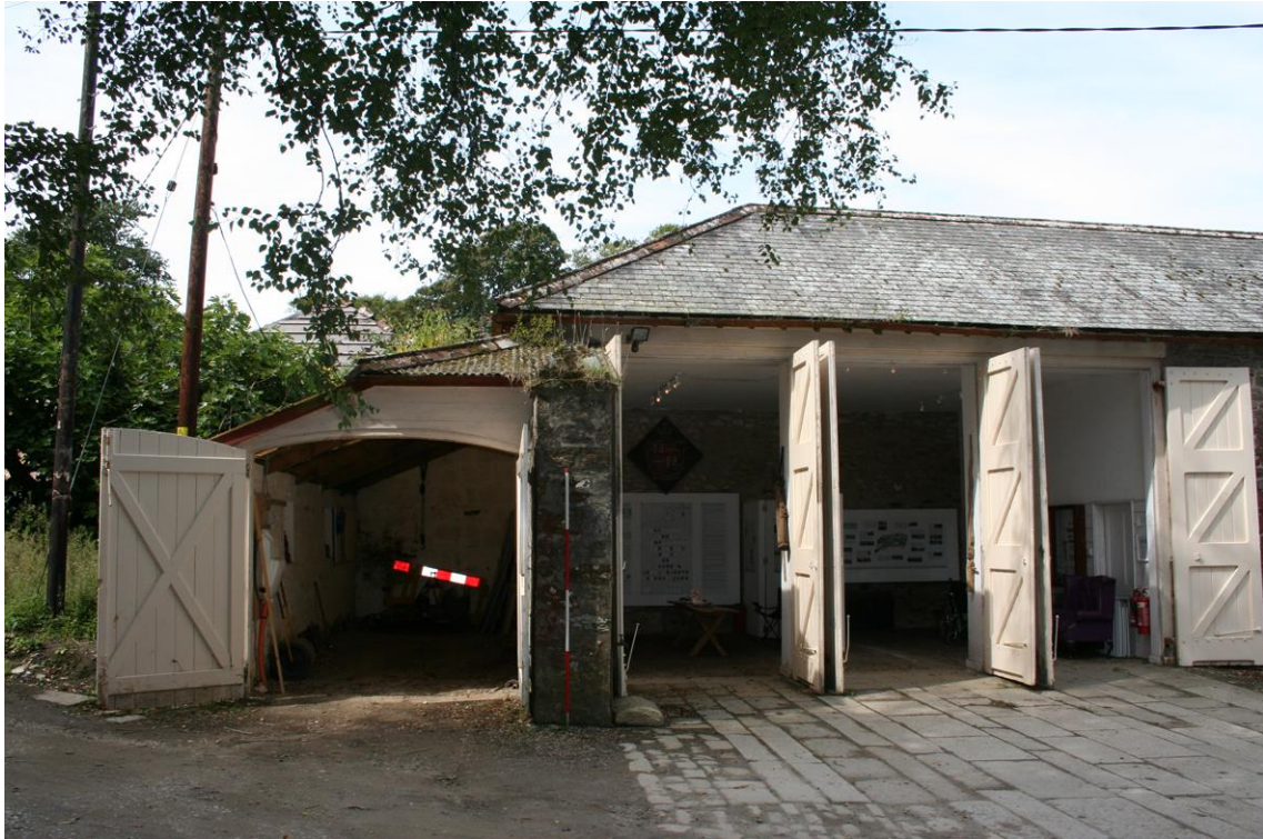
Figure 23 Stables Range – upper end of the south-east elevation of the stables, showing a later lean-to addition [1] to left of the coach house [2].
