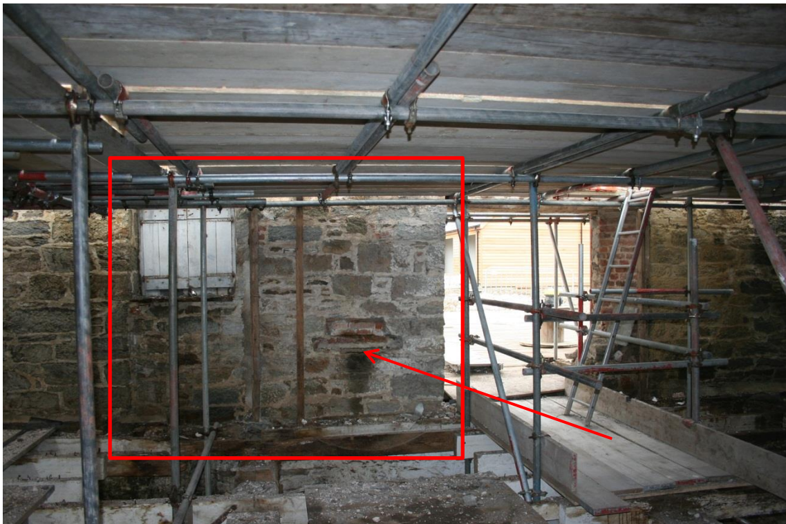
Figure 46 South-west Range - original threshing doorway (within red rectangle) blocked when horse-engine was added outside, new doorway to right, and machinery bearing support included in masonry (arrowed).
