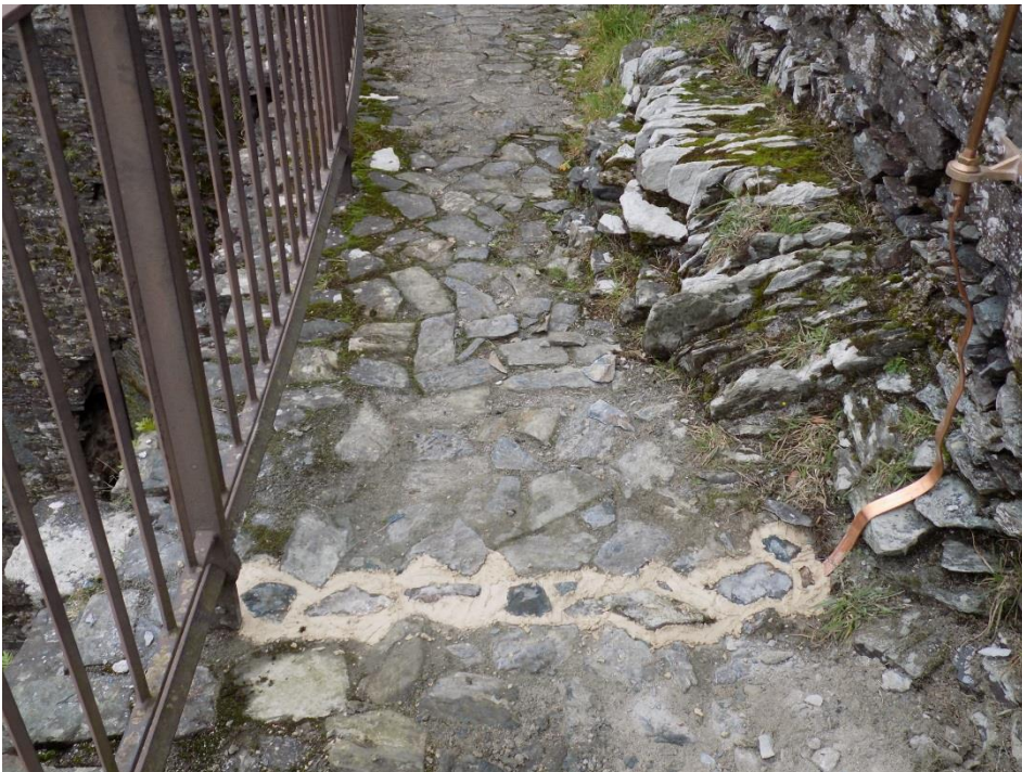
Figure 13. Slot 1 after re-instatement of wall walk surface, the stones bedded within a lime mortar.
