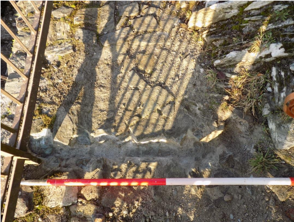
Figure 12. Slot 1 after excavation showing concrete bedding for the stone surface of wall walk.
