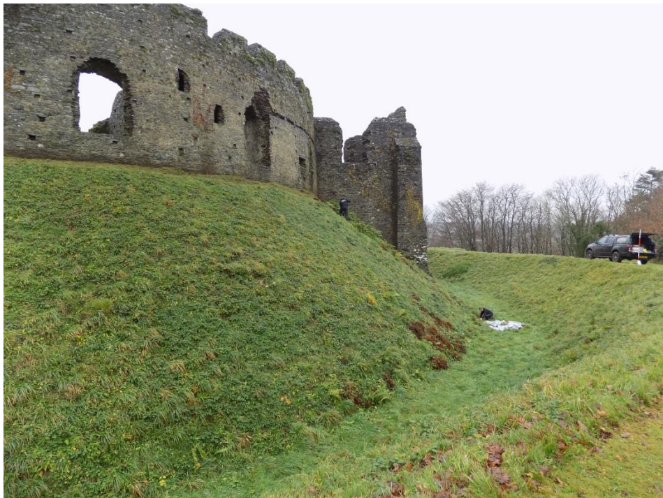
Figure 5. View of site looking north-west showing location of conductor tape trench and pit for the earthing plate.
