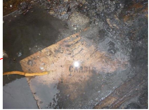
Figure 11: Floor tile CARBIS (111) in situ.
