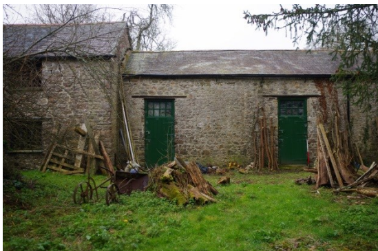
Fig 261 south end of east elevation of stables and north end of Pound House.
