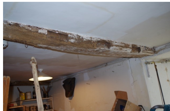
Fig 161 Room 11 second joist from east showing recesses for removed stud partition wall.
