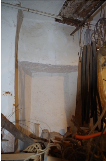
Fig 156 Room 11 blocked window and evidence for possible west extent of phase 1 building.
