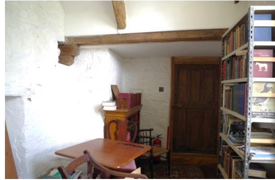
Fig 206 Room 25 looking north showing chimney breast and stone wall with inserted door opening.
