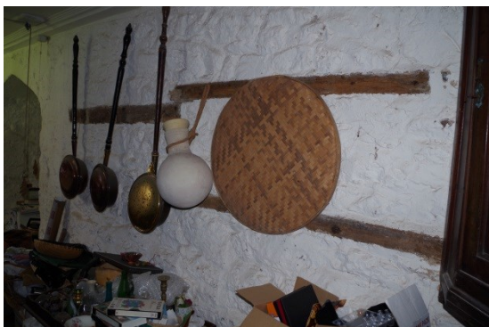
Fig 152 Room 9 timber inserts in west end of south wall (former external wall).
