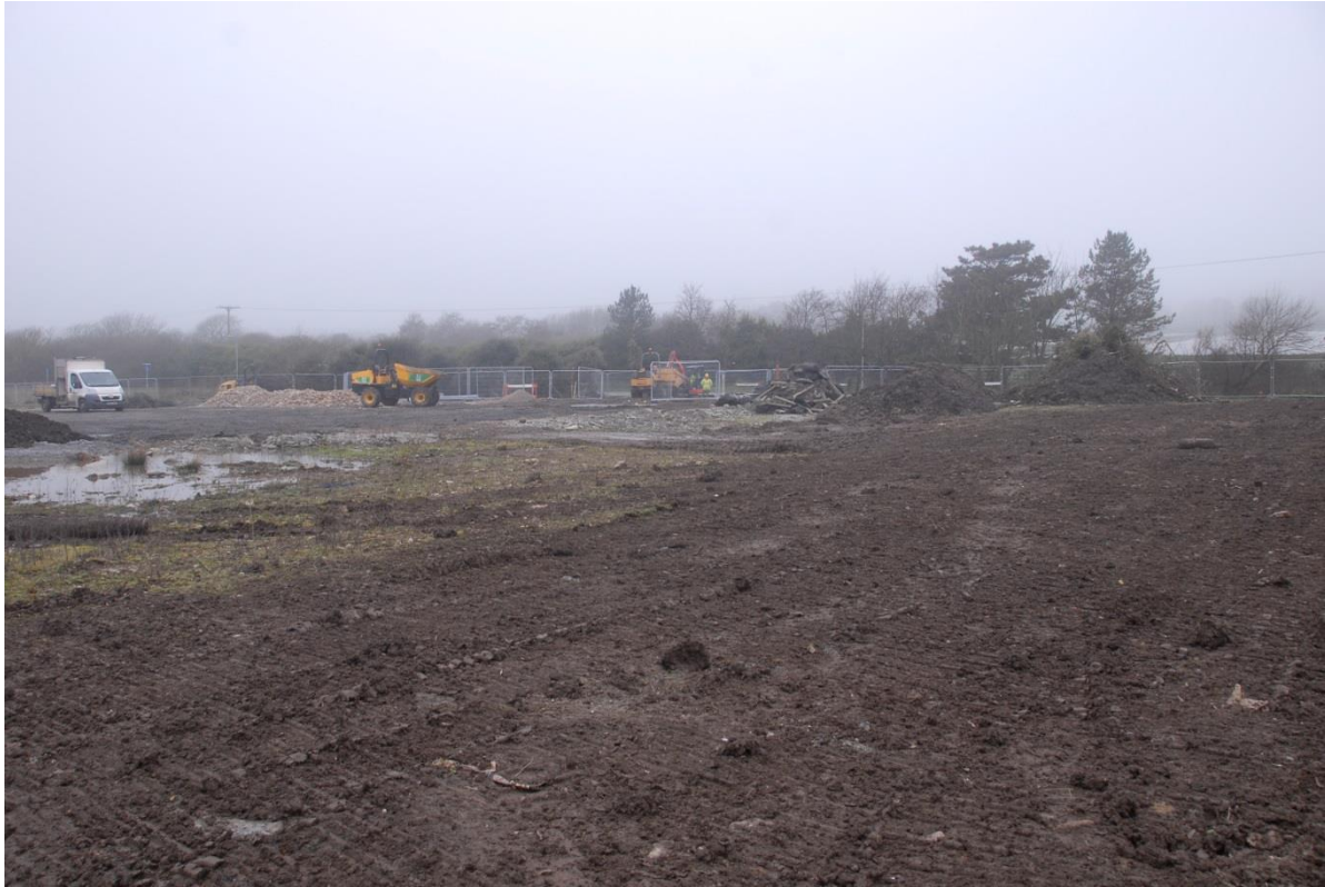
Fig 5. A general view looking north across the site during the early stages of the works. The area to the right had been skimmed of topsoil, whilst the new site entrance is in the background at the centre of the image.
