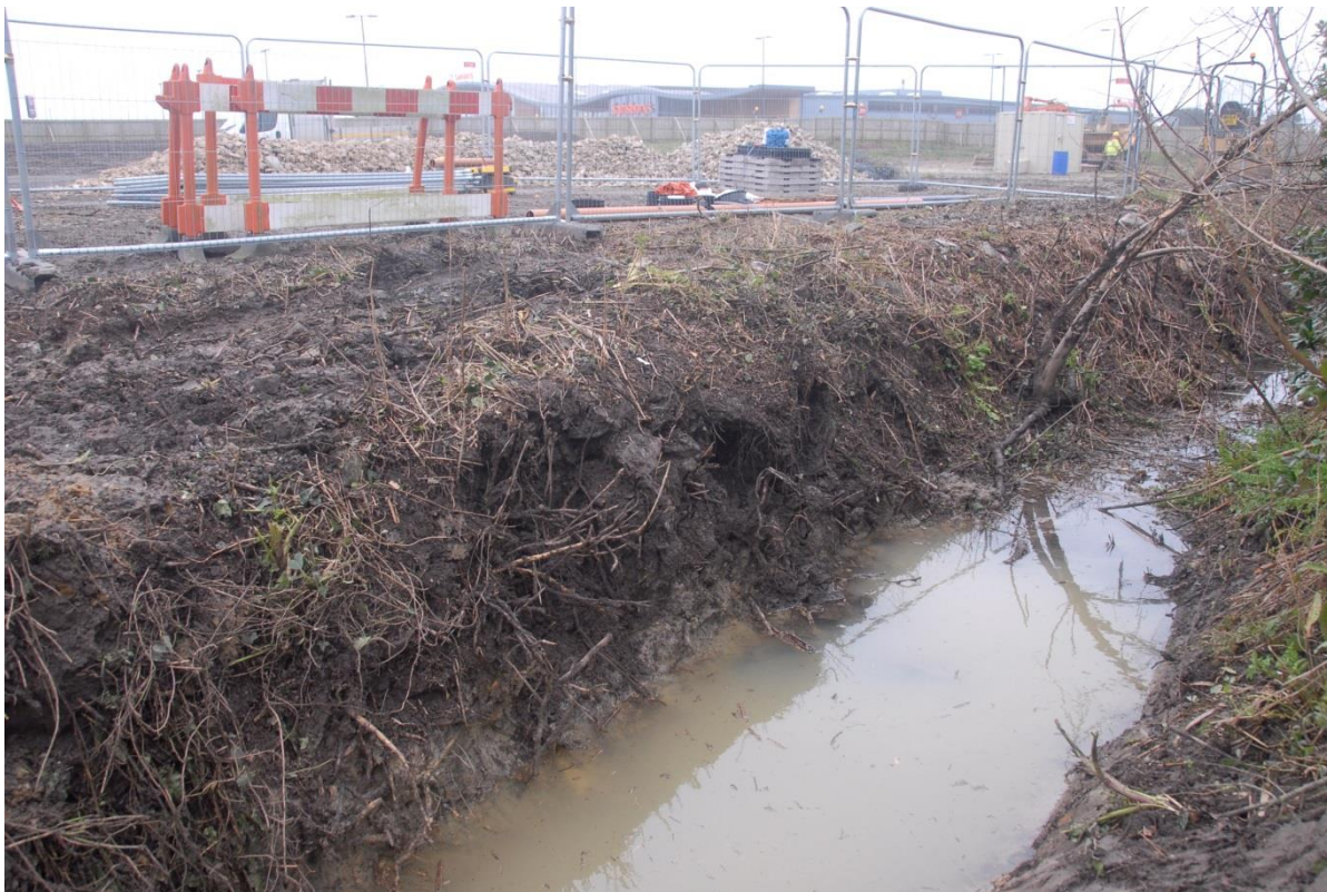
Fig 6. The drainage ditch along the northern side of the site, showing the mixed topsoil at surface overlying the upper parts of the clay into which the ditch had been excavated.
