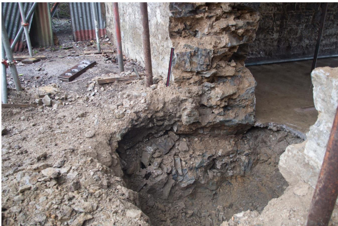
Figure 16 Block D, Rooms 32 and 25 – test pit showing the depth of the rear wall of the main part of Block D.
