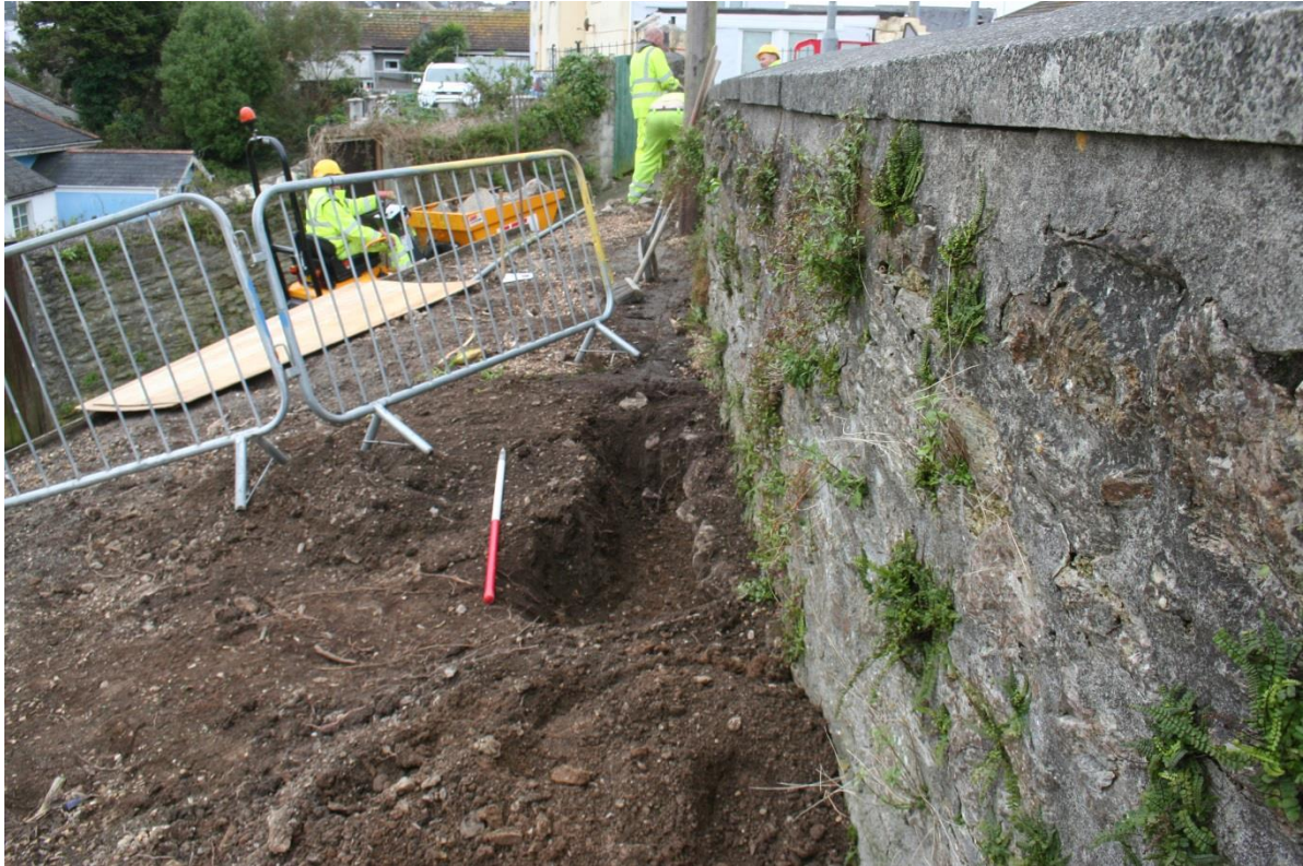
Fig 2 Looking to the test pit at the foot of the Erisey Terrace wall. Note the insubstantial footings to the wall projecting out into the test pit.
