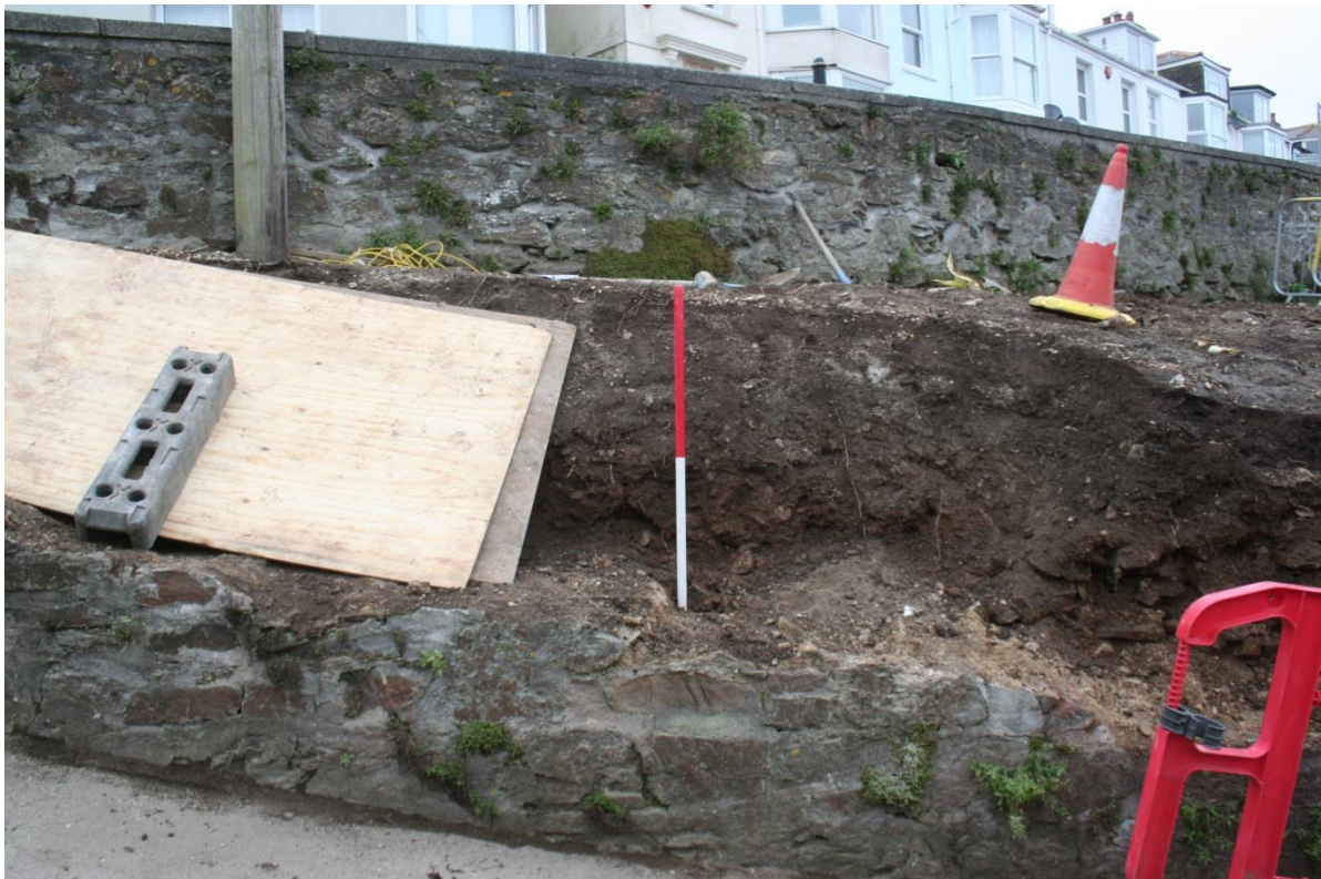
Fig 3 Mid-excitation. The lower revetment wall has been lowered and the depth of the topsoil has been revealed.
