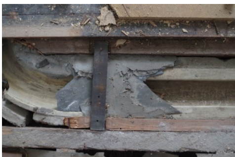
Fig 26 Quadrangle: below floor drainage in science lab (room 51).
