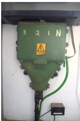
Fig 50 Quadrangle: electricity service head at top of room 60.
