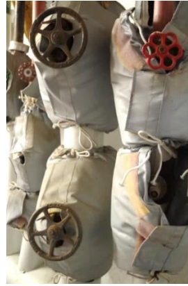
Fig 51 Quadrangle: examples of water faucet handles on pipes in boiler room (room 60).
