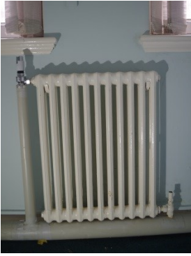
Fig 39 Quadrangle: example of cast iron radiator (room 11).
