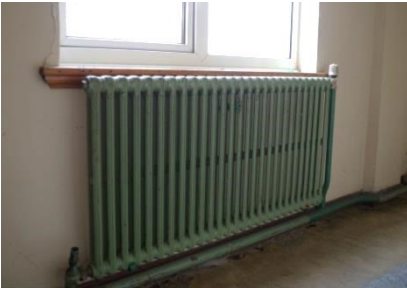
Fig 40 Quadrangle: example of cast iron radiator (room 28).
