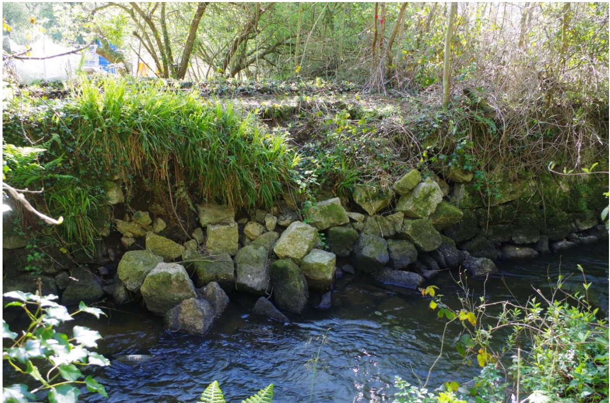
Figure 4. Collapsed embankment prior to work commencing.
