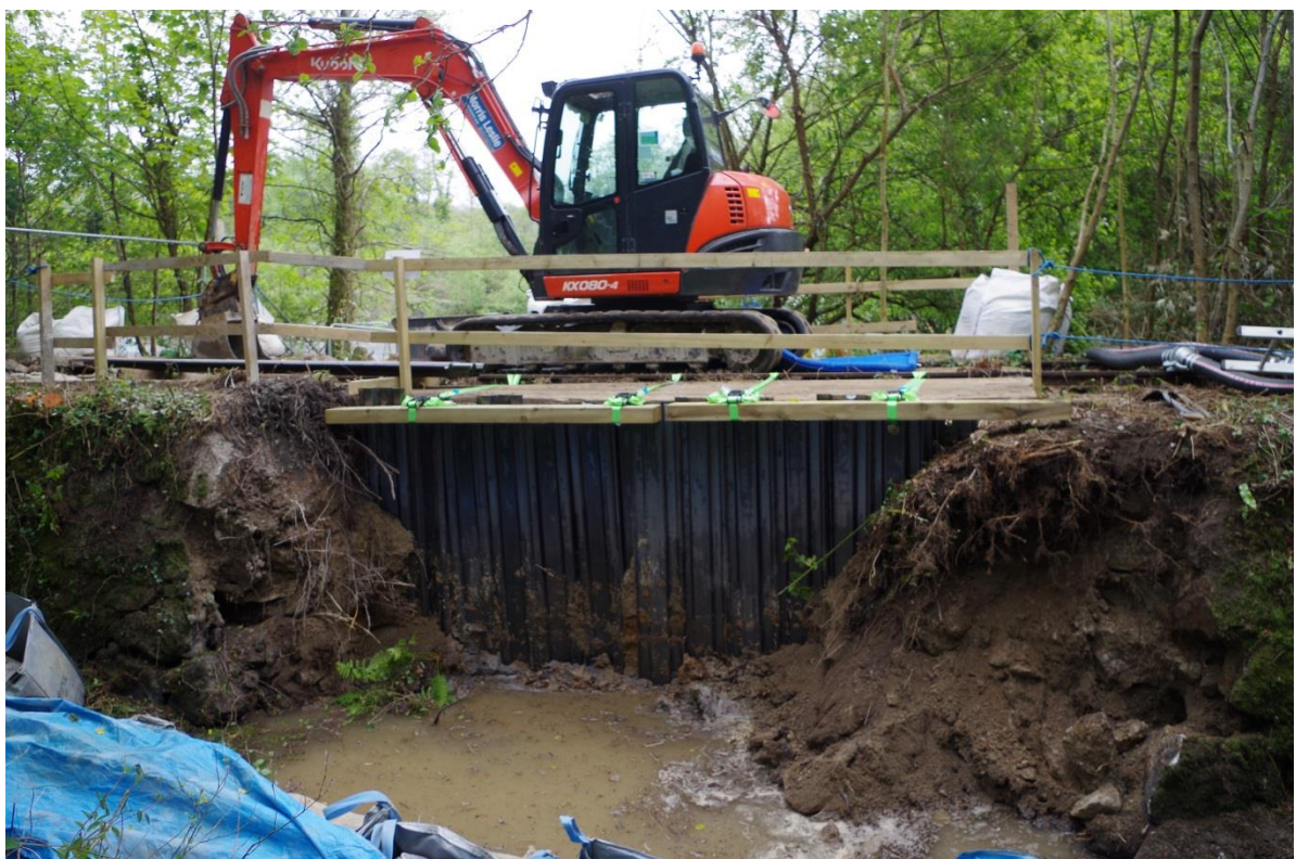
Figure 5. Embankment after clearance of collapse showing location of sheet piling.
