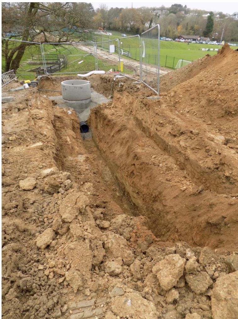
Figure 22. Scheme 9. Priory Park. Storm drain trench. Section to north of manhole A showing nature of ground encountered.
