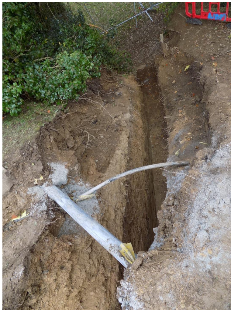
Figure 21. Scheme 9. Priory Park. Storm drain trench. Section on hillside immediately above St Petroc's Well looking south east.
