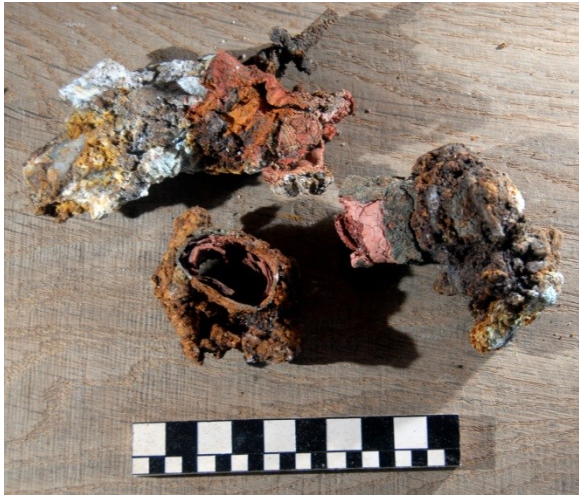
Fig 29. Badly decayed rubber pipe connectors.
