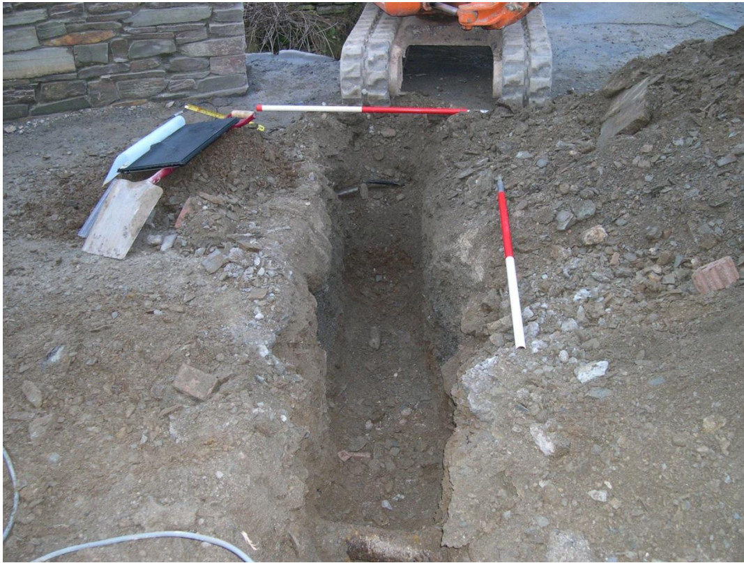
Fig 9. The services trench excavated in Area 4 in 2003 (Dudley 2004) showing the built up material interpreted as a slate processing yard and the iron pipe (bottom centre).
