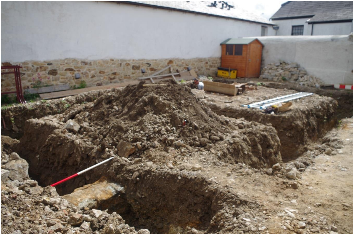
Fig 7. The development area showing the foundation trenches, with wall (3) exposed to the left. The stable block wall behind forms the eastern side of the plot.
