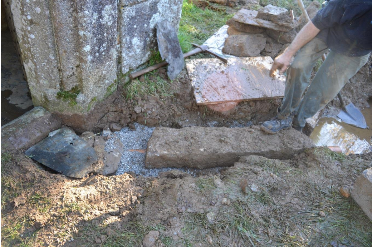
Fig 25. Pea gravel laid around the pipe, and the slate and granite launder replaced where they had been found.
