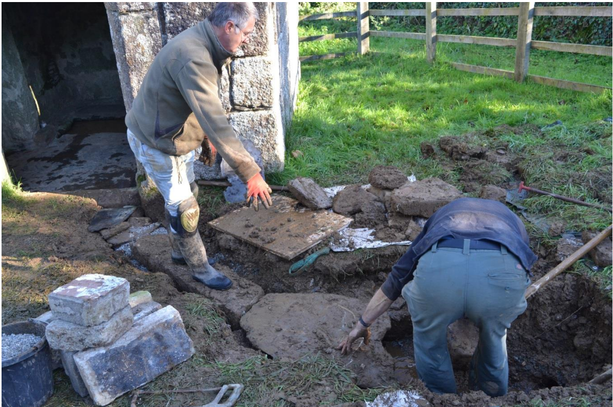
Fig 26. The first slate slab replaced over the rebuilt chamber, close to its original position.
