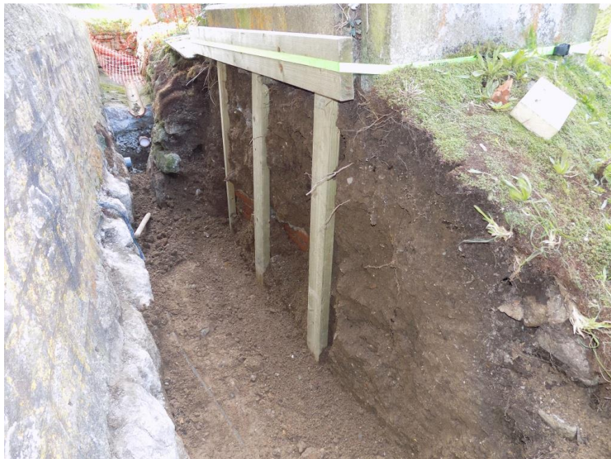
Figure 13. French drain section after removing collapsed wall and cleaning up of the section face. Note traces of brick vault, structure 14.
