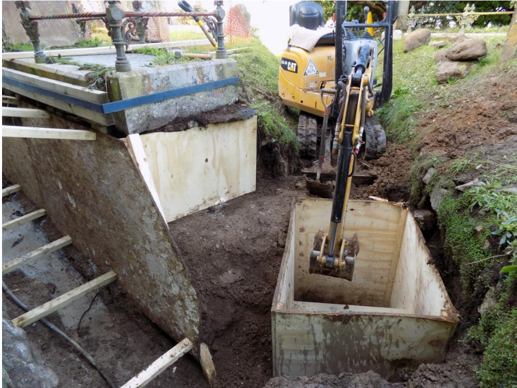
Figure 14. Pumping station pit outside north door of church showing digging box, and shoring around the French drain section.
