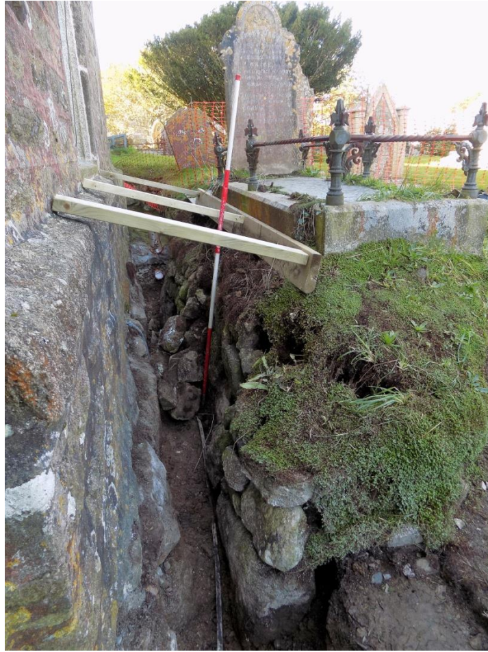
Figure 12. French drain section after revetment wall section collapse.
