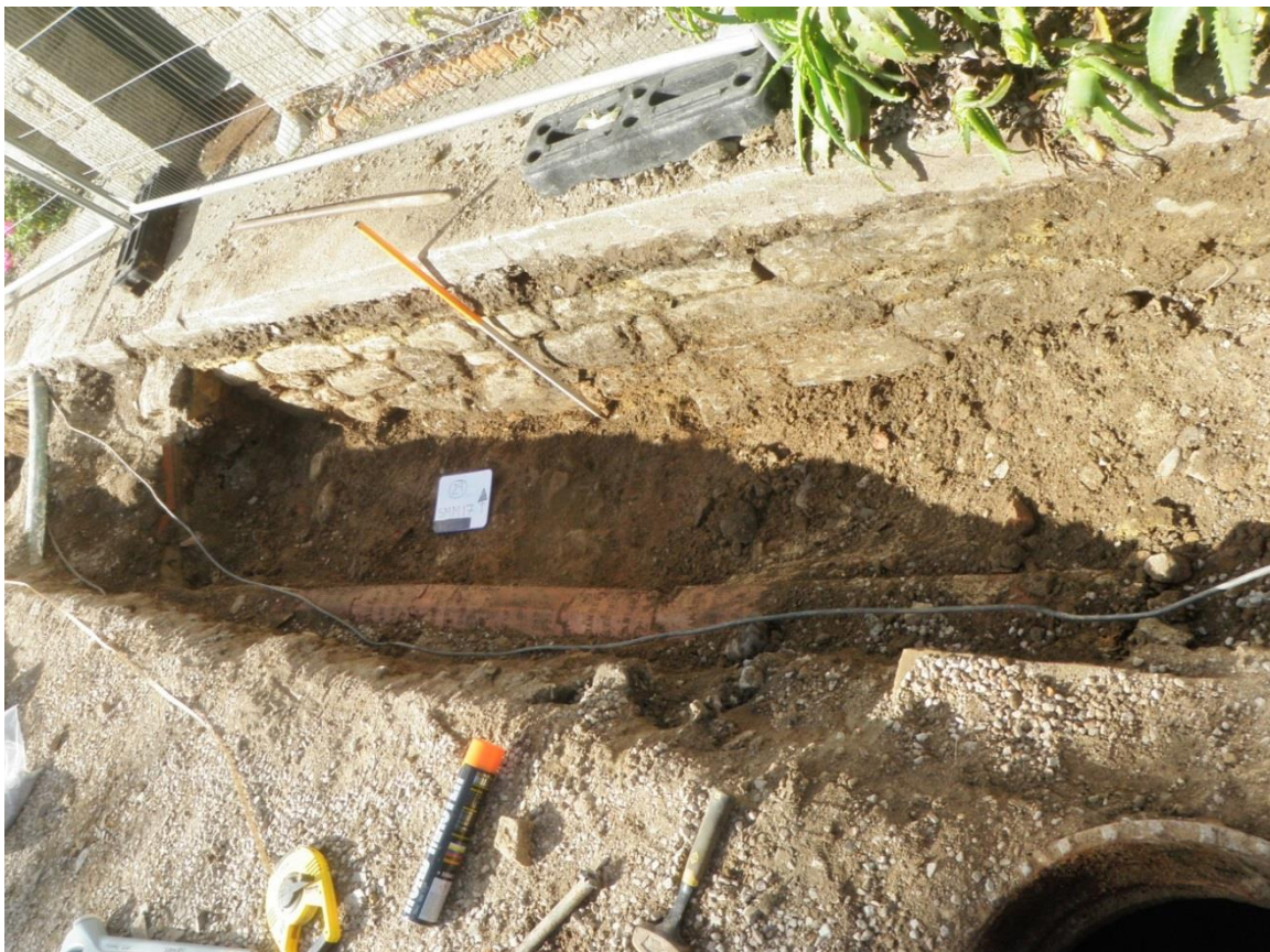
Fig 17 Looking down to the northwest from the eastern end of trench E showing part of wall 25 and an open service hatch on the right.
