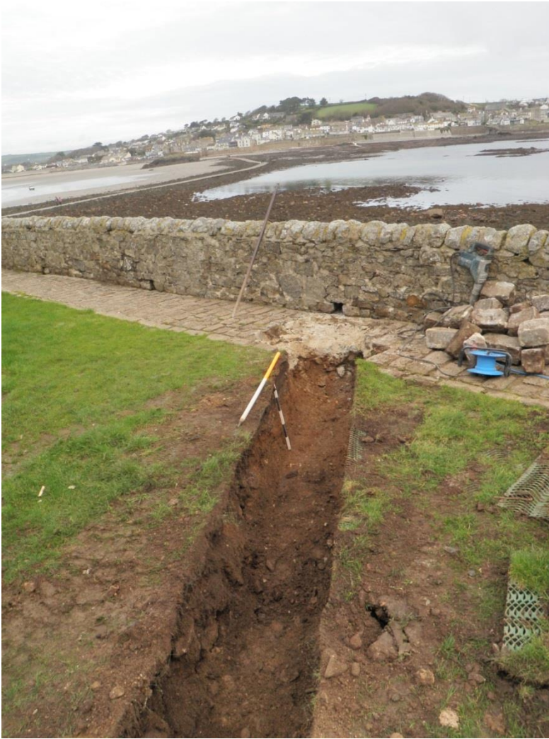
Fig 46 Looking north along the northern end of trench I/2 showing trenching running up to the path and sea wall.
