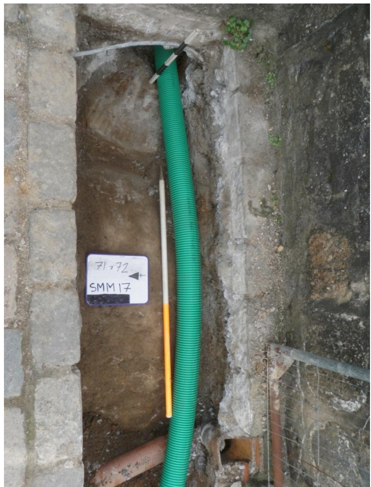
Fig 29 Looking down across the roof of the tunnel 72, showing wall 71 at the top of the photograph beneath the current wall. The green pipe running beneath the wall and over the tunnel roof has just been laid.
