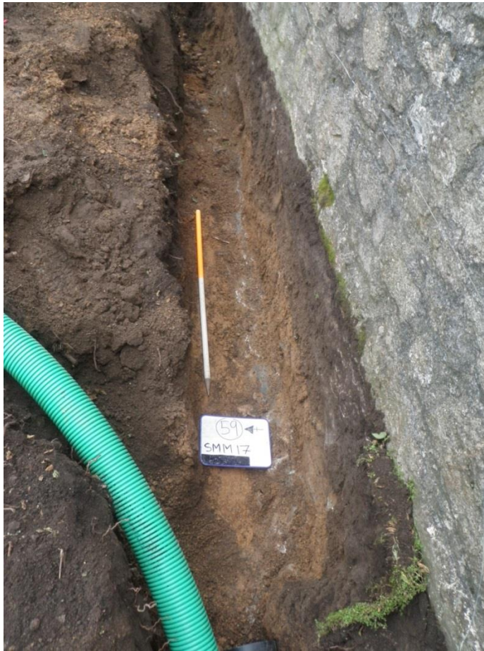
Fig 28 Looking east along trench G/E showing wall 59 at the base of the trench beneath the current standing garden wall.
