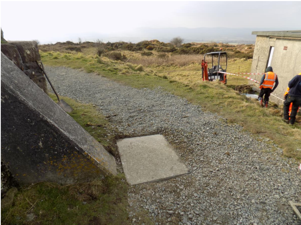
Figure 5. View looking west across site. Draw pit A in foreground, Draw pit B in background in front of the person wearing a reflective jacket.
