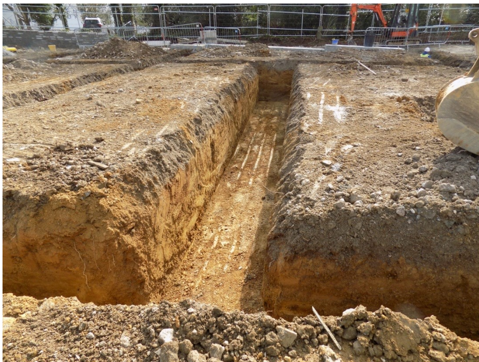
Figure 14. Overview of building foundation trenches in vicinity of profiles 13 and 15, looking south, clearly showing levelling layer (8) spread across the area overlying the natural (9).
