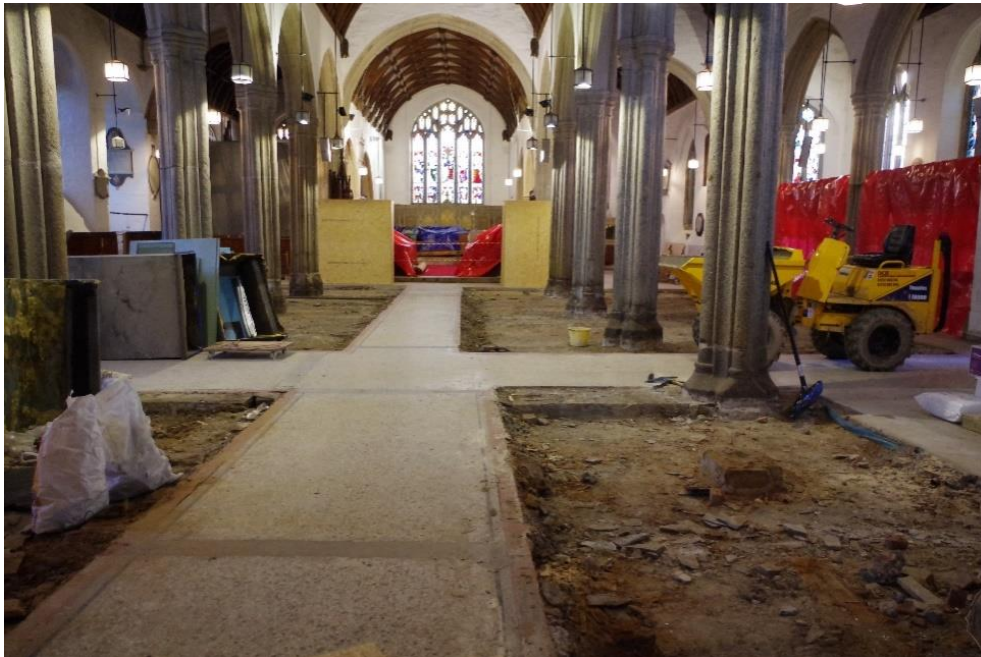
Figure 2: General overview of the floor to be removed, looking east down the centre of the Nave.
