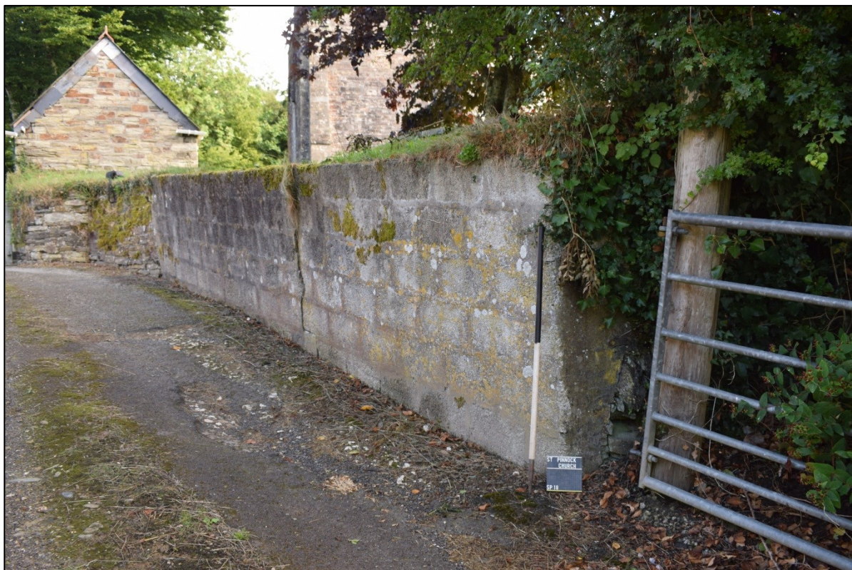
Figure 3: Pre-works view of the section of wall to be re-built. (1m scale looking north).
