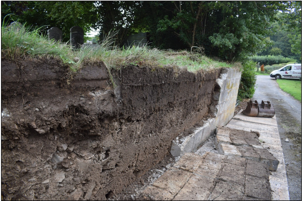
Figure11: Looking south-east after the removal of the north-western section of the wall.
