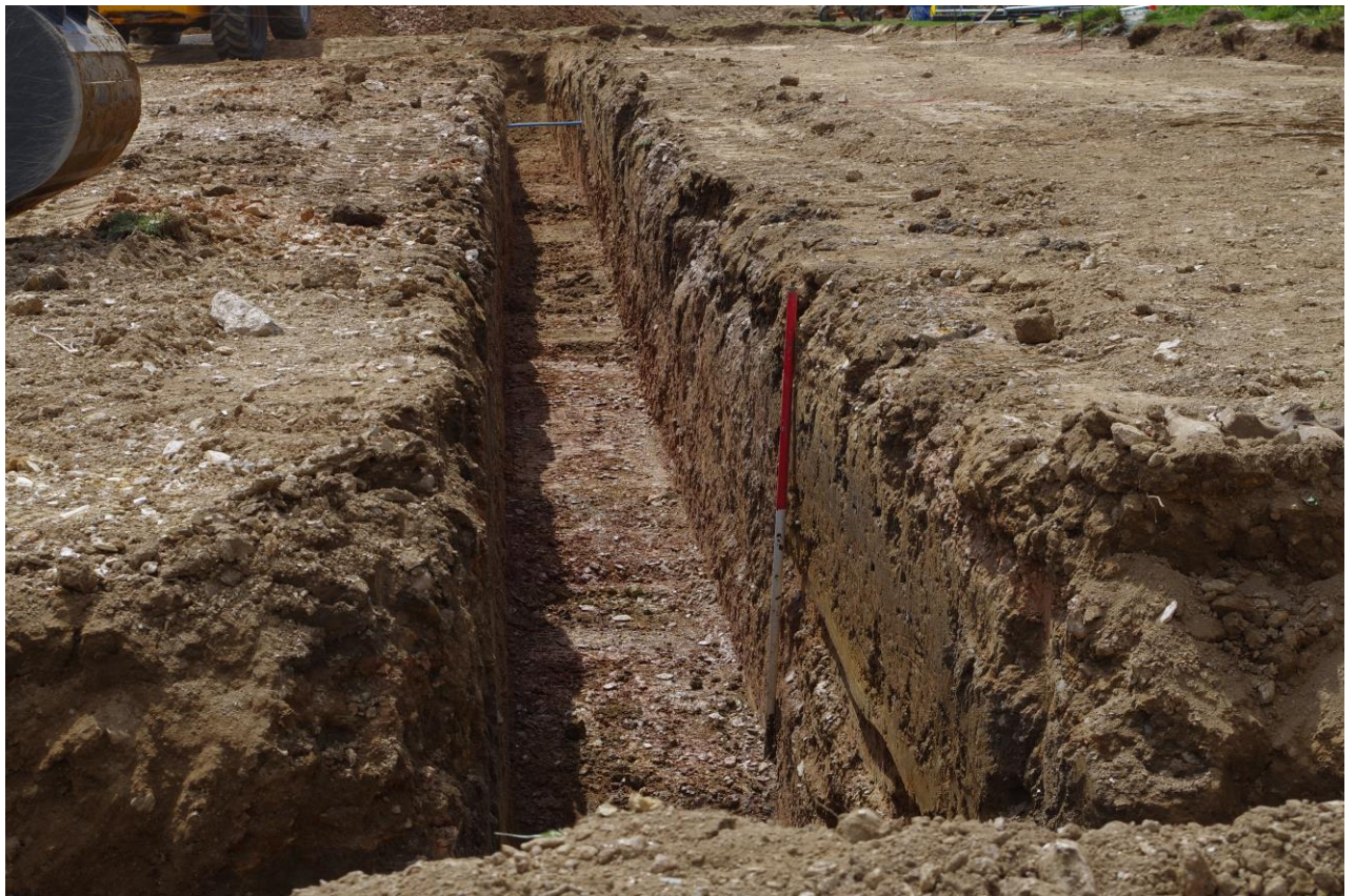
Fig 7 North east trench, looking NW, showing uniformity of make-up of ground with distinct stony layers extending across the site.
