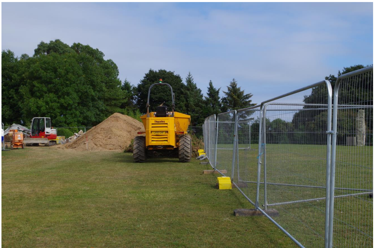
Fig 10 Spoil heap south of site at the conclusion of the watching brief, showing the Longstone protected from any direct impact.
