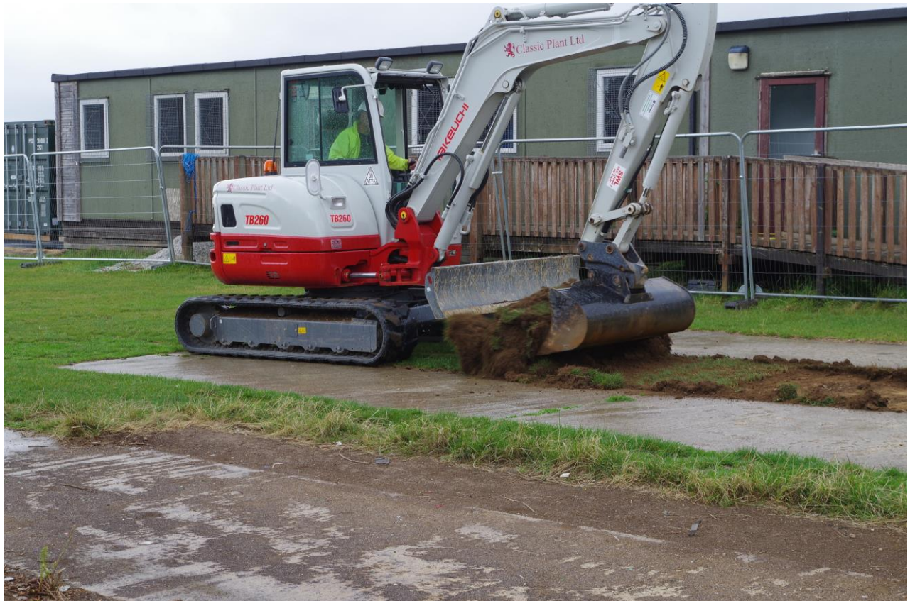
Fig 4 North west side of site at start of works, showing existing concrete standings, looking west.
