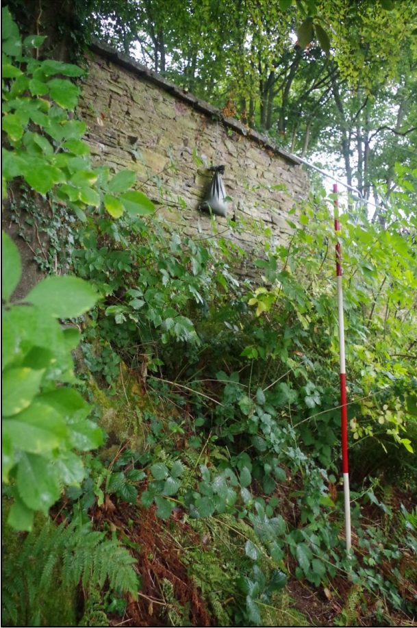
Figure 11. Eastern (The Woodlands) side of the boundary wall showing 'embankment' in foreground, and two construction phases to the wall.
