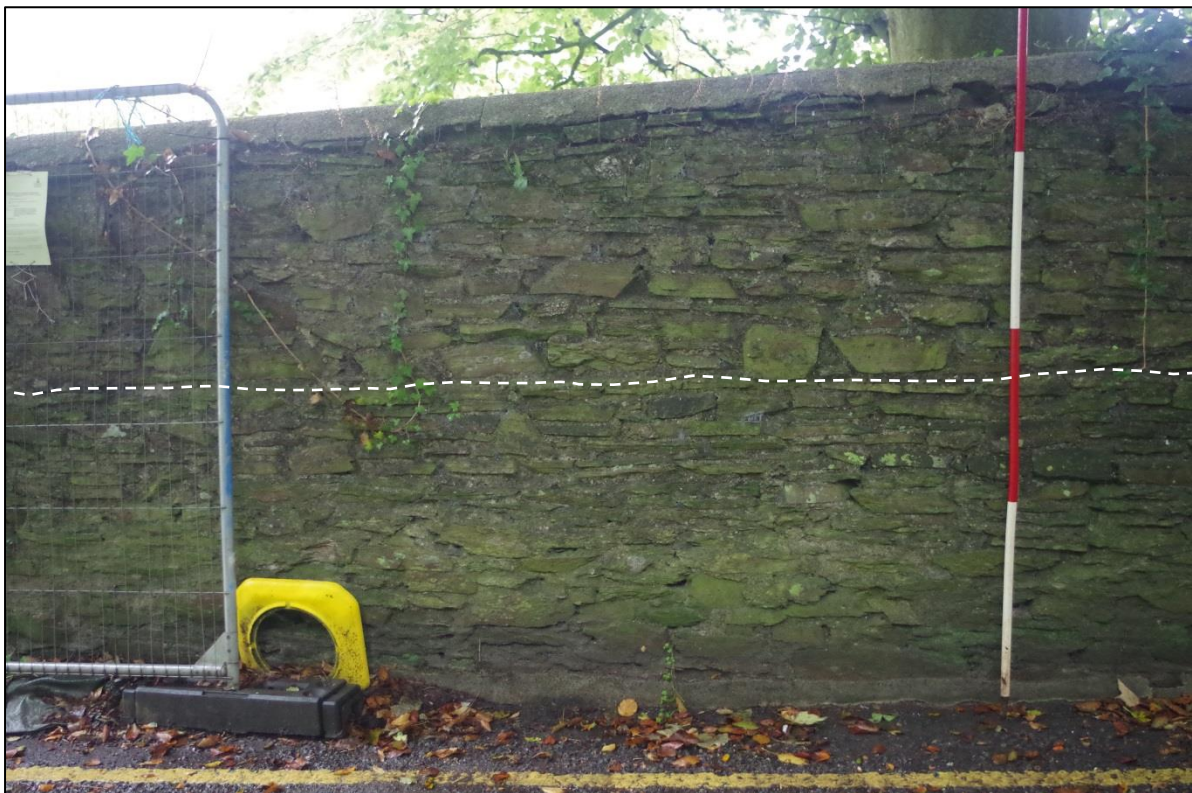
Figure 10. Detail of walling on the New Road side showing the two phases of construction.
