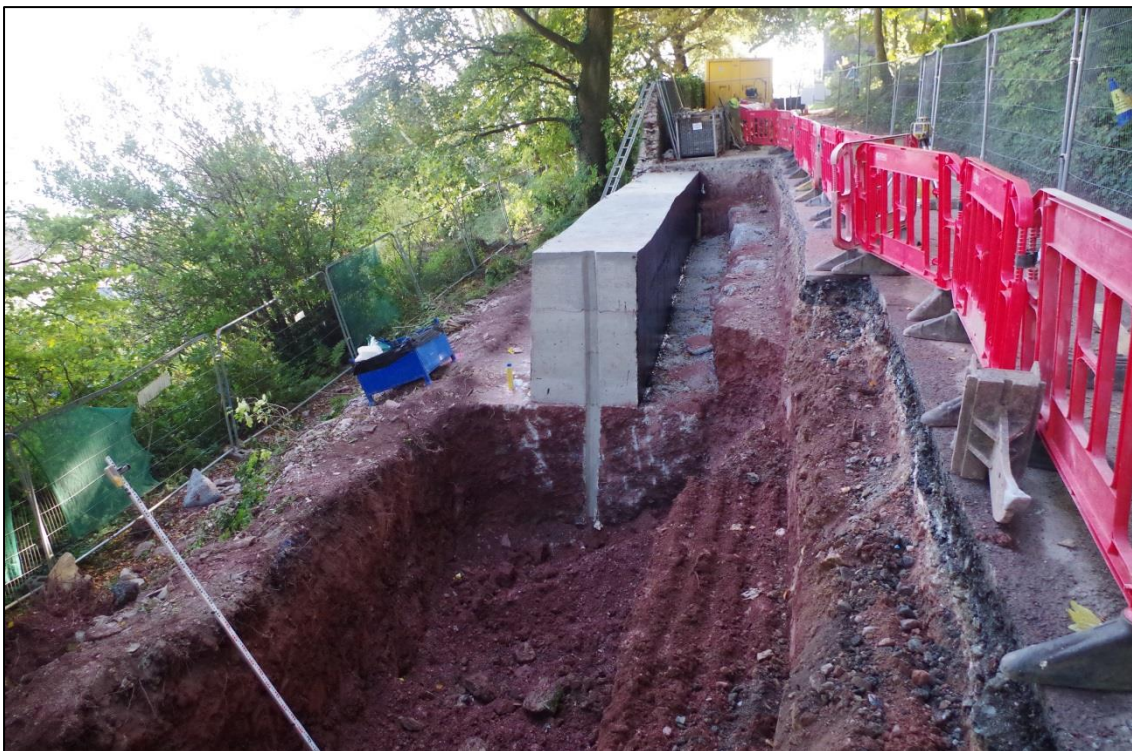
Figure 16. View looking south east showing concrete platform foundation and core to new wall.
