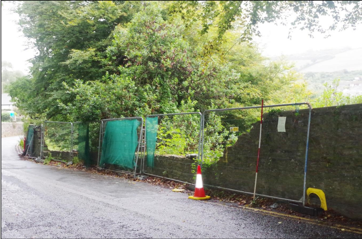
Figure 9. View of damaged walling looking north.
