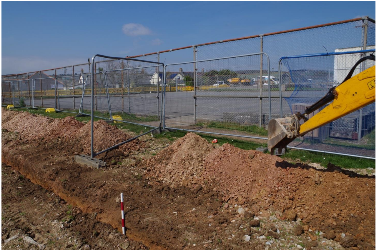
Fig 5 Southern part of pipeline trench, looking north west, showing typical section with 1m scale.
