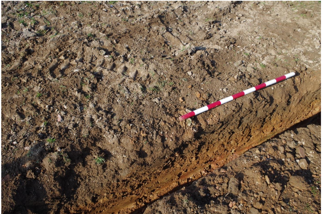
Fig 6 Southern part of pipeline trench, looking north east, showing detail of typical section with 1m scale.
