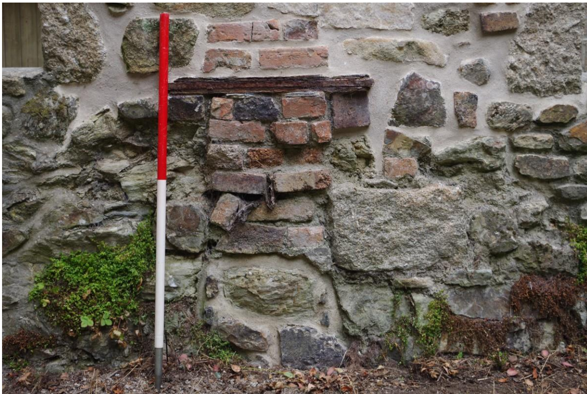
Fig 21. Detail of the repair works surrounding the flue opening near the base of the wall. The joints between the blocking bricks have not been repointed, and no stabilisation treatment has been applied to the iron lintel.
