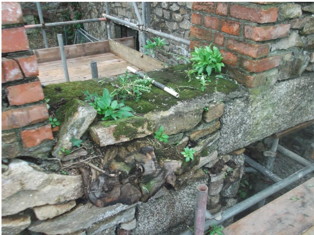
Fig 9. A view of the area around the upper floor window following the cutting back and stump treating of the Buddleia, showing the size of some of the destabilising root growth.
