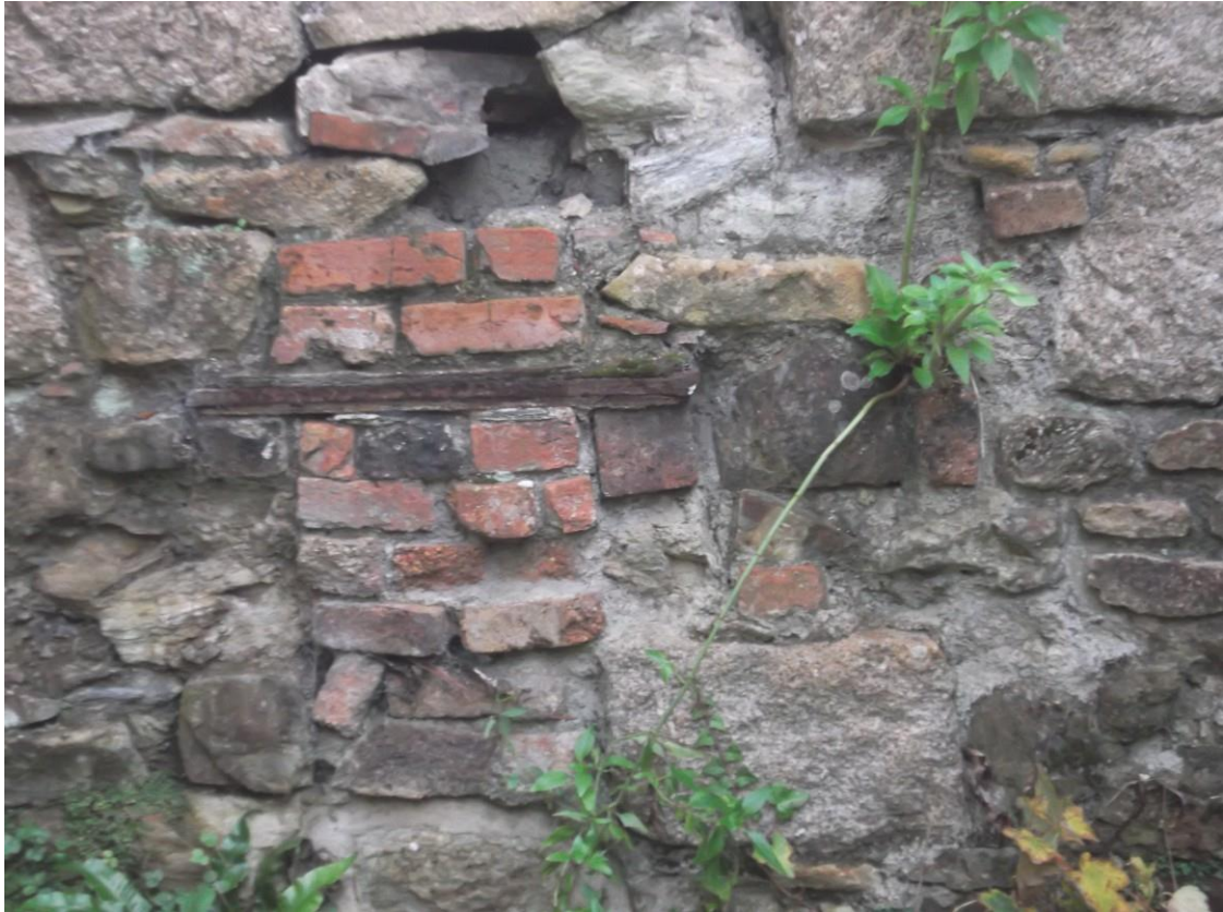
Fig 12. The blocked flue opening on the internal elevation of the section of wall which was repaired.
