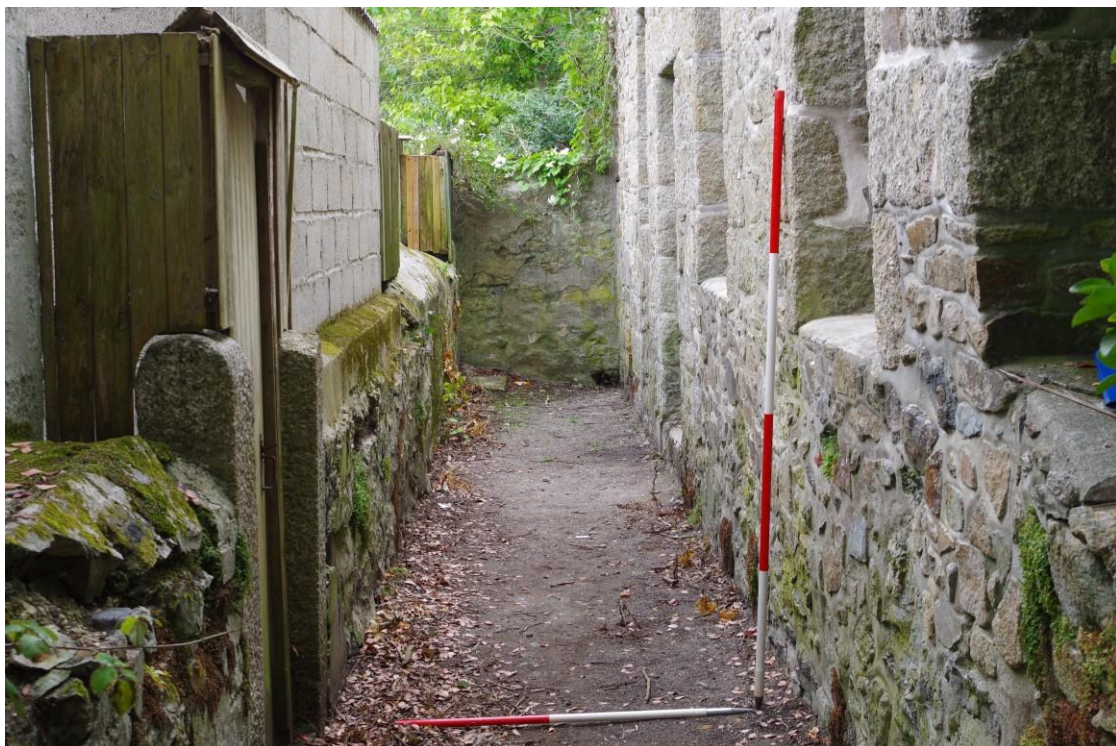
Fig 19. A view of the repair works from the footpath to the east of the building.
