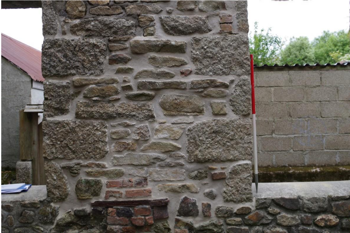
Fig 20. Detail of the partially reconstructed and fully repointed stonework forming the wall panel between the two windows, this incorporating the integral flue.
