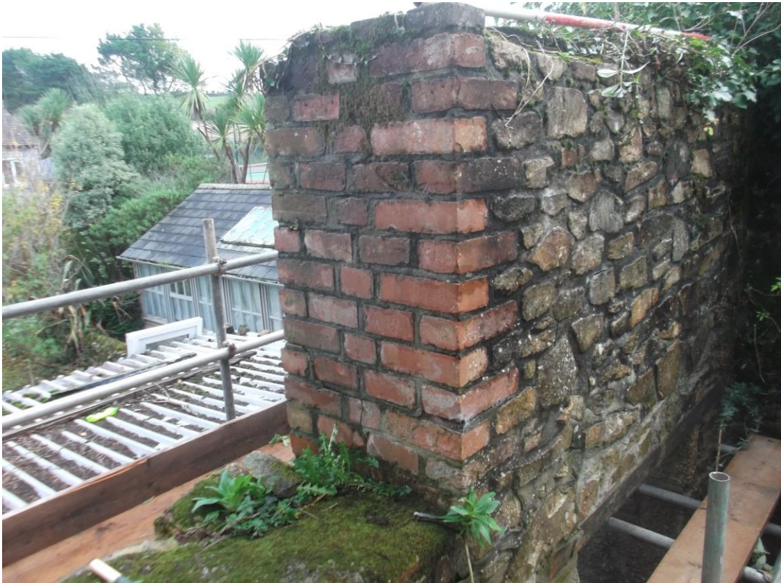
Fig 10. The southern reveal of the upper floor opening, showing the vegetation growth on the cill and wall capping.
