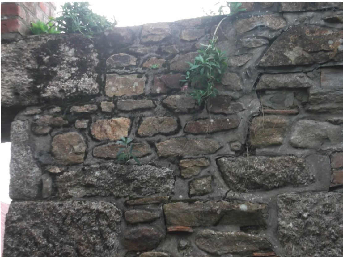
Fig 13. A view of the section of walling between the wall openings showing its cementitious pointing, Buddleia growth and eroded or cracked wall joints.
