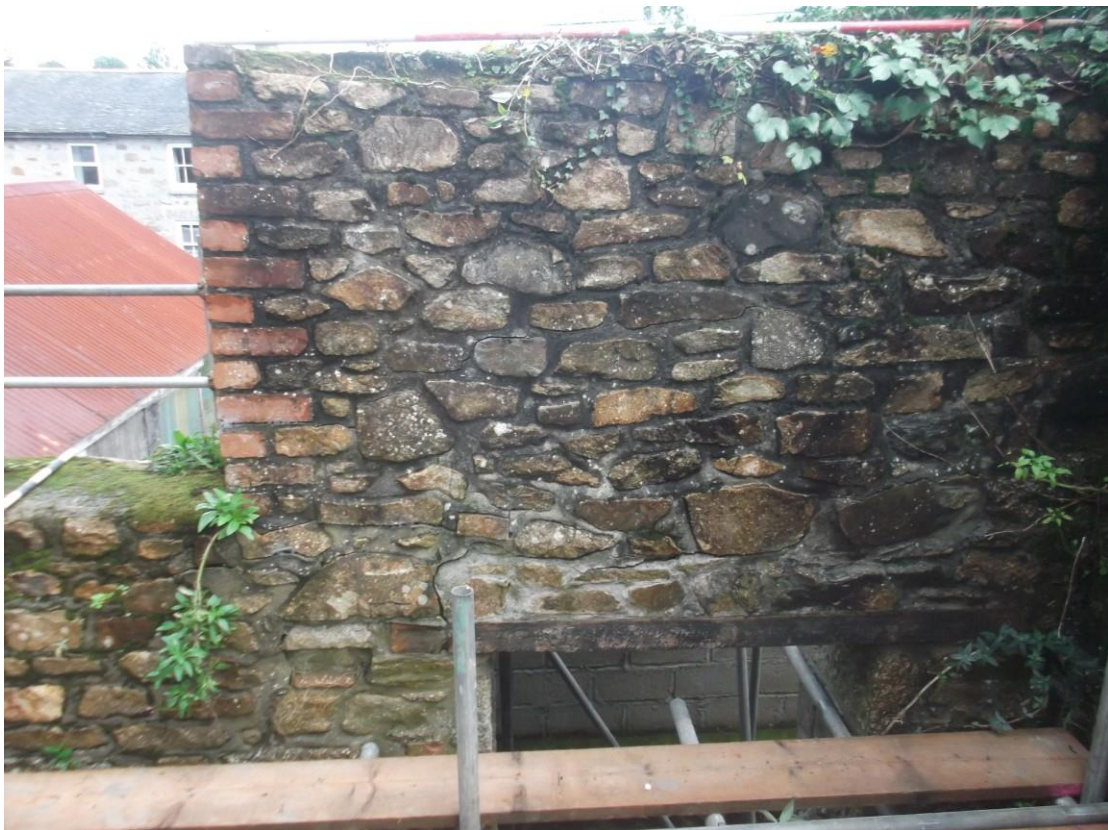
Fig 11. The original (replacement) timber lintel to the ground floor wall opening. As can be seen in this view, this had begun to fail and cracking had appeared within the pointing of the walling it supported.
