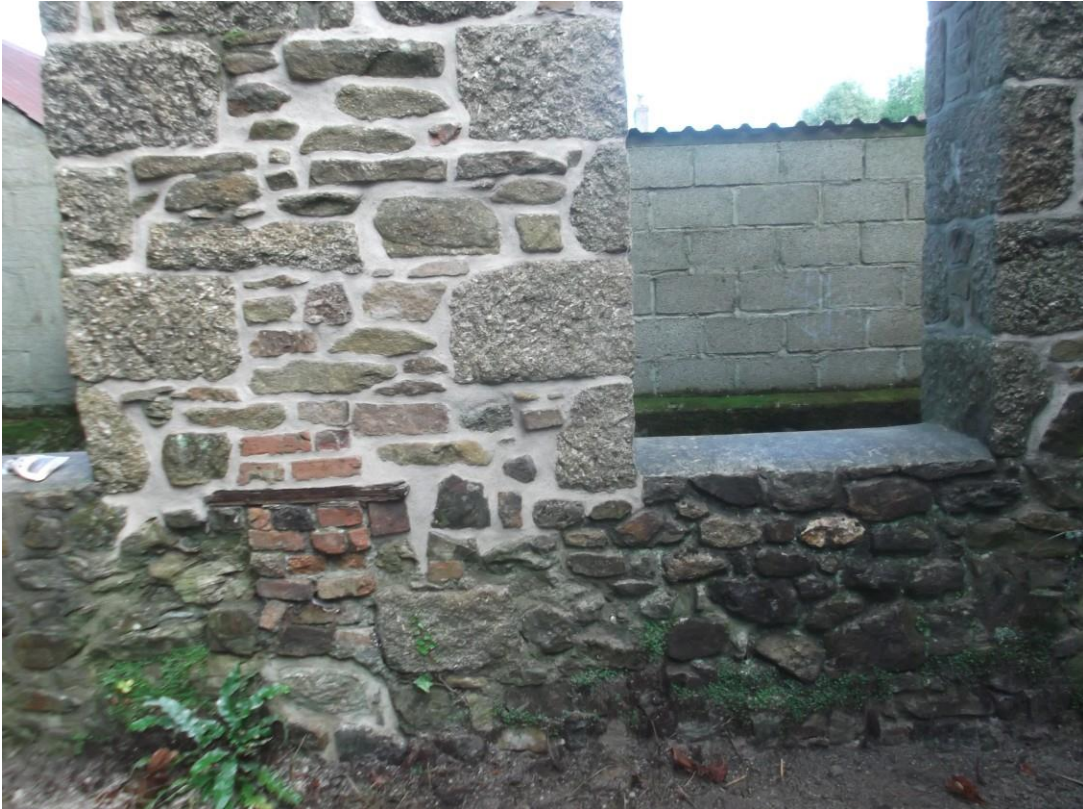
Fig 16. Repointed and partially rebuilt stonework adjacent to the flue opening on the internal wall face.
