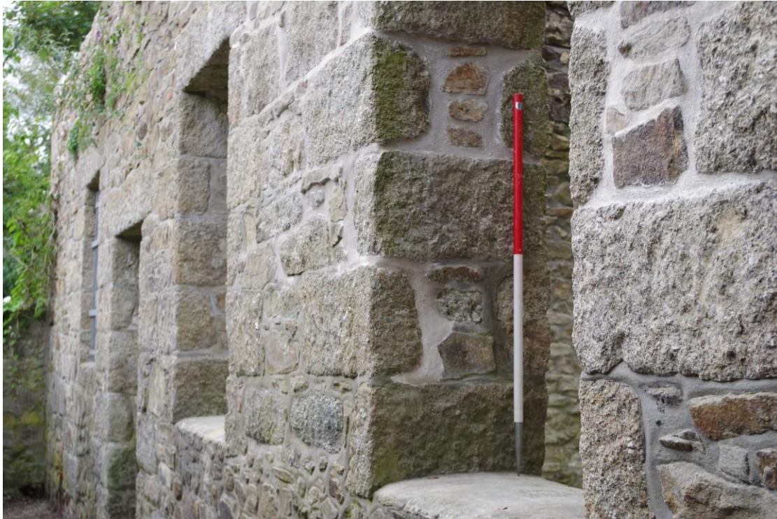
Fig 18. A view of the repair works to the exterior of the building and a window reveal, showing the appearance of the replacement pointing.
