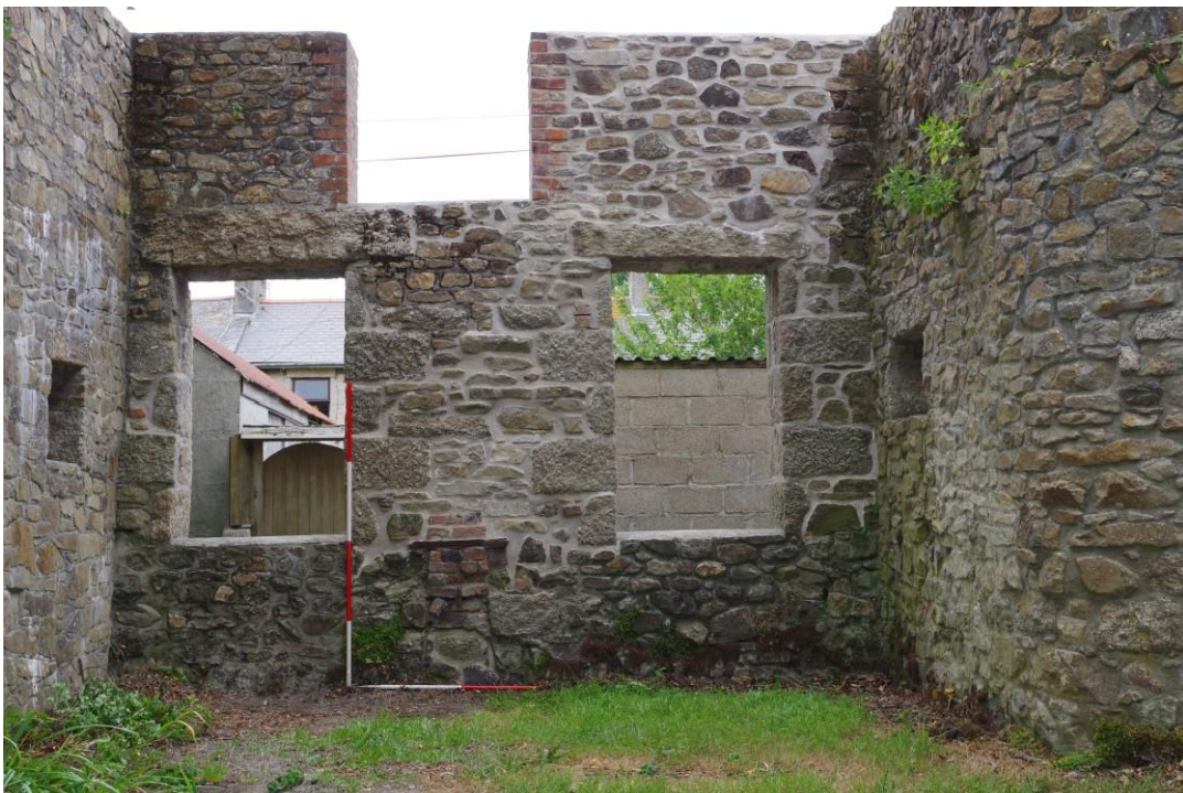
Fig 17. A view of the reconstructed and repointed section of the eastern wall of the building, including (right) the replacement granite lintel.
