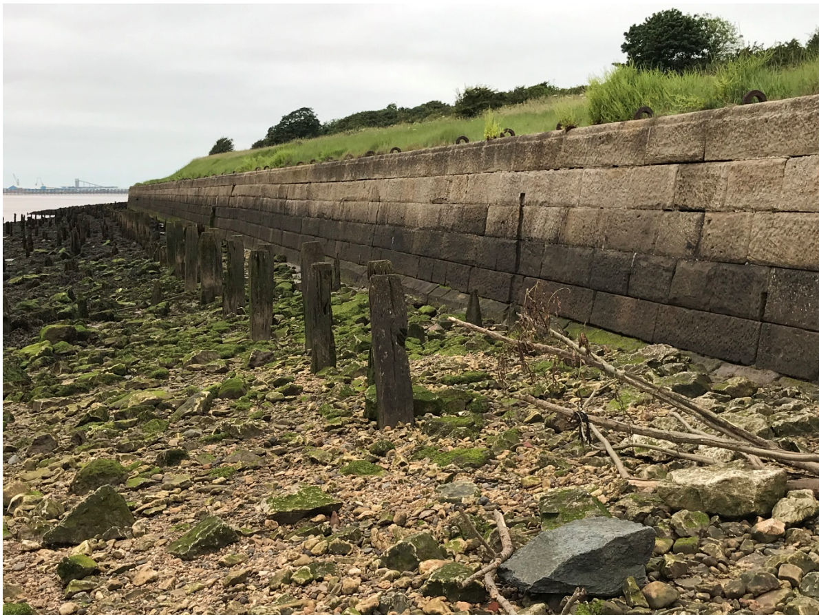
Figure 11.1 Paull Point Coastal Battery – in places it is at risk of coastal erosion.
