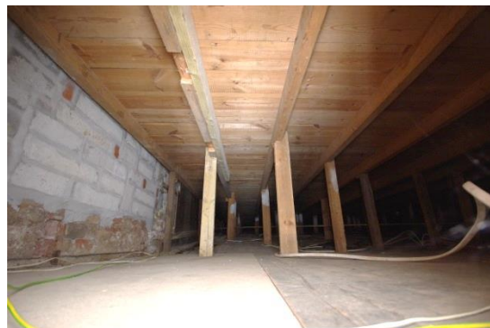
Fig 80 Room 8: Void between dance floor and earlier cinema floor beneath. Looking north from the hatch in room 1.
