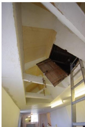
Fig 127 Room 14: Bar and canteen (former small hall) Raised area in Canteen ceiling with hatch door to roof space.
