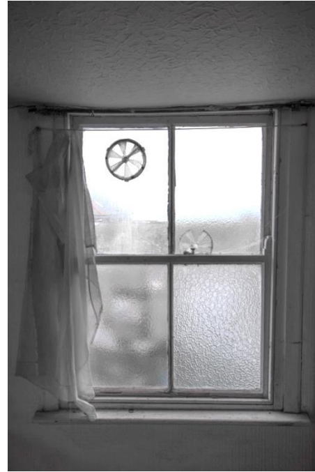
Fig 121 Room 14: Bar and canteen (former small hall) late 19 th or early 20 th century sash window in bar area's east wall.
