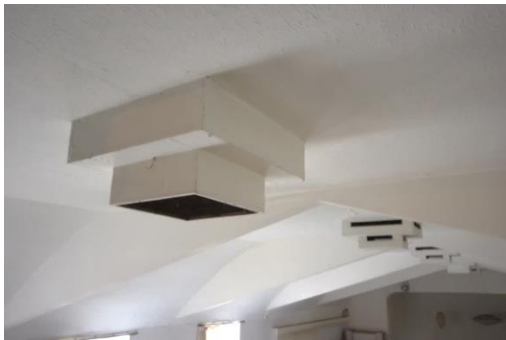
Fig 159 Room 22: Dancehall, 1950s ventilation ducts in the ceiling.
