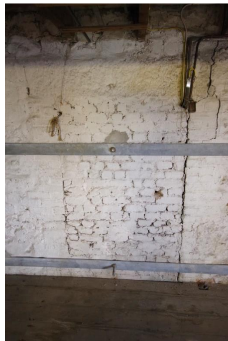
Fig 105 Room 11: Lower workshop (former store) blocked window opening in north wall at mezzanine level.
