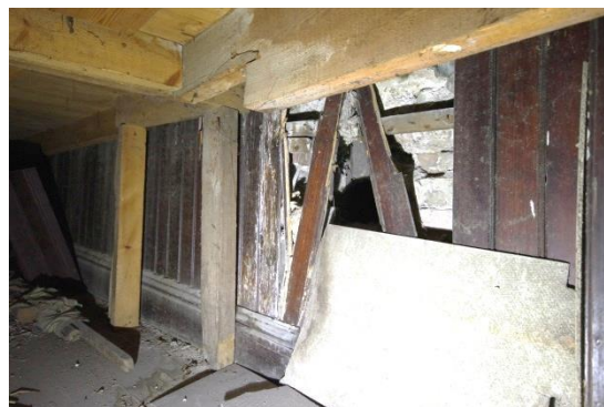
Fig 82 Room 8: Void between dance floor and earlier cinema floor showing matchboard panelling on cinema wall to east.
