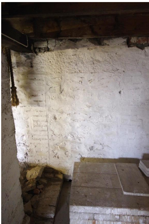
Fig 107 Room 11: Lower workshop (former store) blocked window opening in west wall at mezzanine level.
