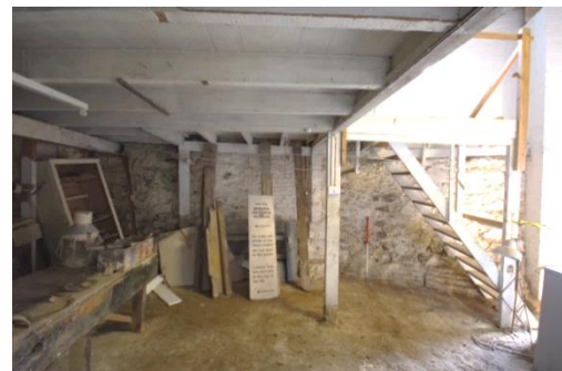
Fig 97 Room 11: Lower workshop (former store) looking east at northern end of ground floor level.
