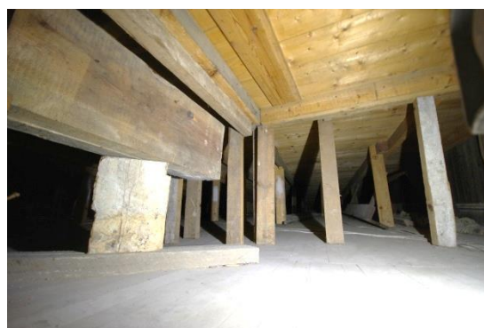
Fig 81 Room 8: Void between dance floor and earlier cinema floor looking north with later boards above where staircase has been removed.
