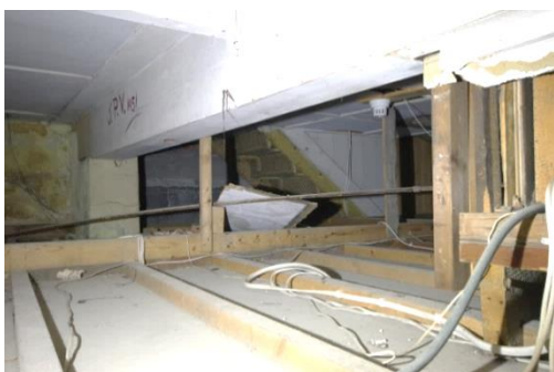
Fig 84 Room 8: Void between dance floor and earlier cinema floor looking south and showing latticed iron structure of main staircase.
