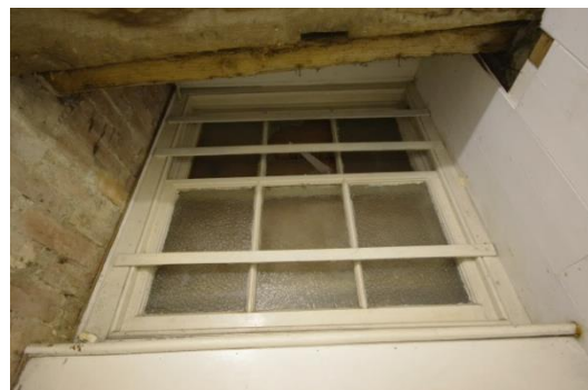
Fig 68 Room 5: Office (former box office and cloakroom) 19 th or early 20 th century sash window.
