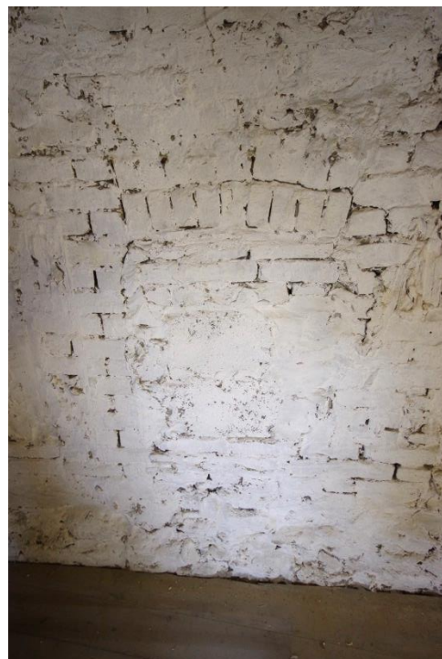
Fig 109 Room 11: Lower workshop (former store) blocked window opening in south part of west wall at mezzanine level.
