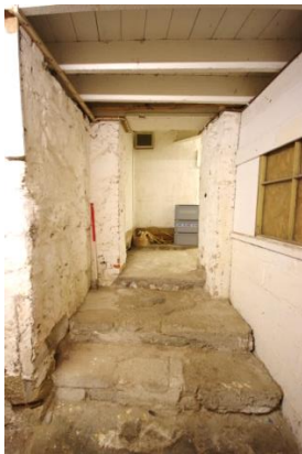
Fig 93 Room 10: Store looking west at door opening and steps inserted by Hepworth.
