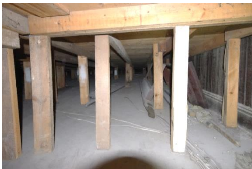
Fig 83 Room 8: Void between dance floor and earlier cinema floor looking north showing upwards slope.
