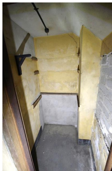
Fig 171 Room 25: Projection room, cupboard at top of Projection room stairs looking east.
