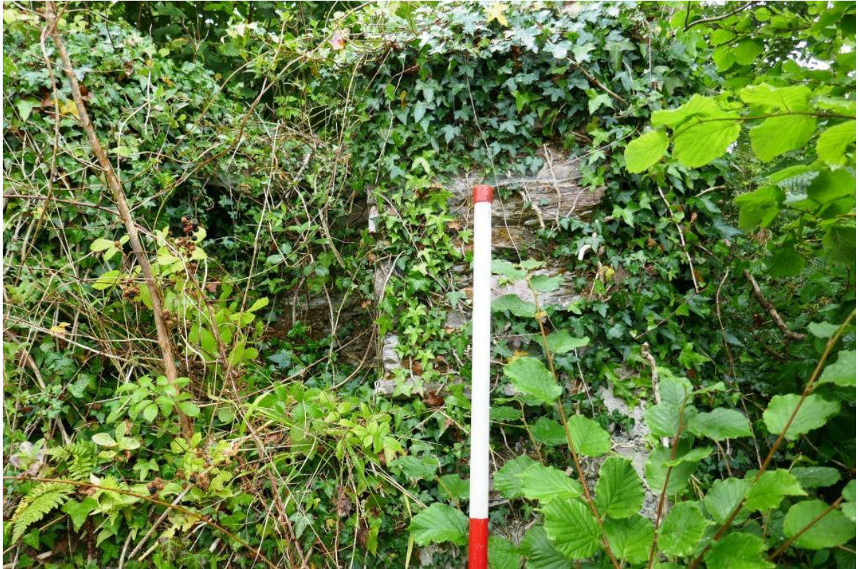
Fig 20 Possible opening and return wall in upper storey inside west end of building 5 on south east.
