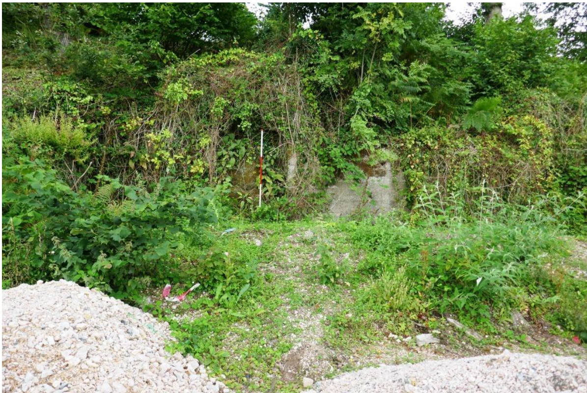
Fig 19 South east building at site 5 before works, looking south, showing rock cut on east (left), and overgrown concrete and stone rear wall (2m scale).
