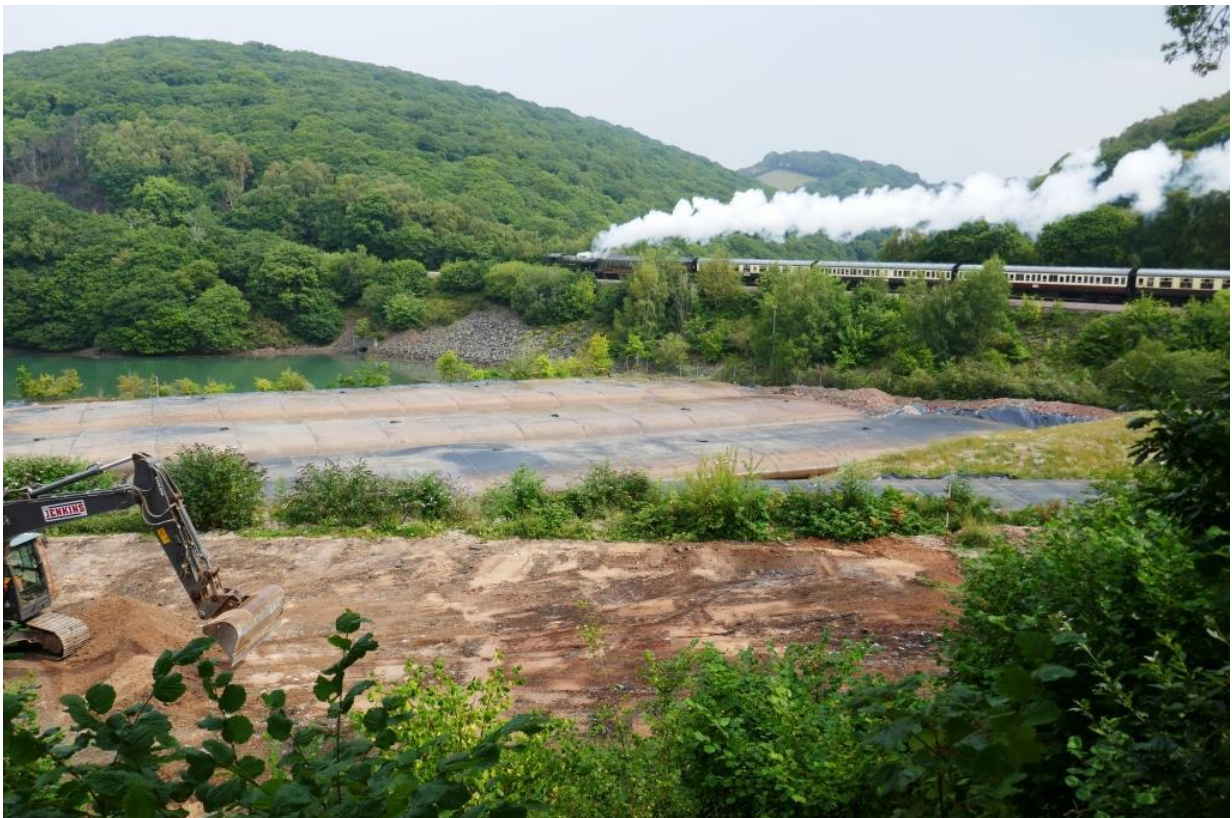
Fig 11 Looking north east during stripping of gravel (112), showing railway (formerly carried across Point and creeks), wooded spur with barrow to left, and hillfort right of centre. The large modern holders at the creek are stores for dredged silt.
