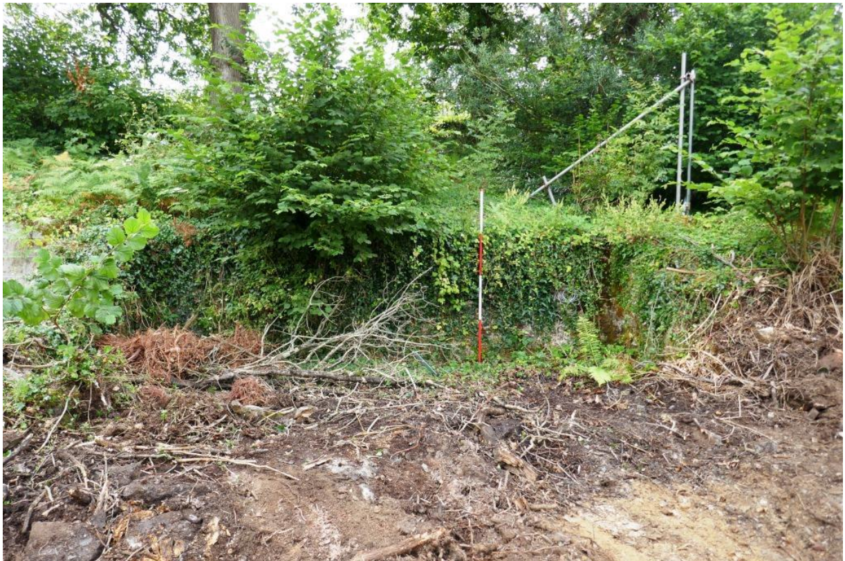
Fig 27 West part of south west building at site 7 at start of works with overgrown walling and mixed loose fill (110) which proved to contain asbestos (2m scale).
