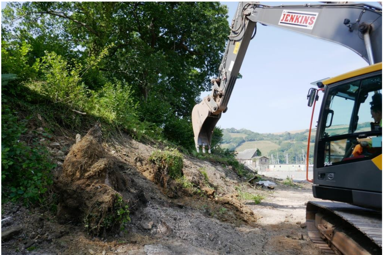
Fig 23 Grading the scarp on the south revealed several large tree stumps. Under topsoil much of the scarp was cloaked in debris tipped from above including asbestos.
