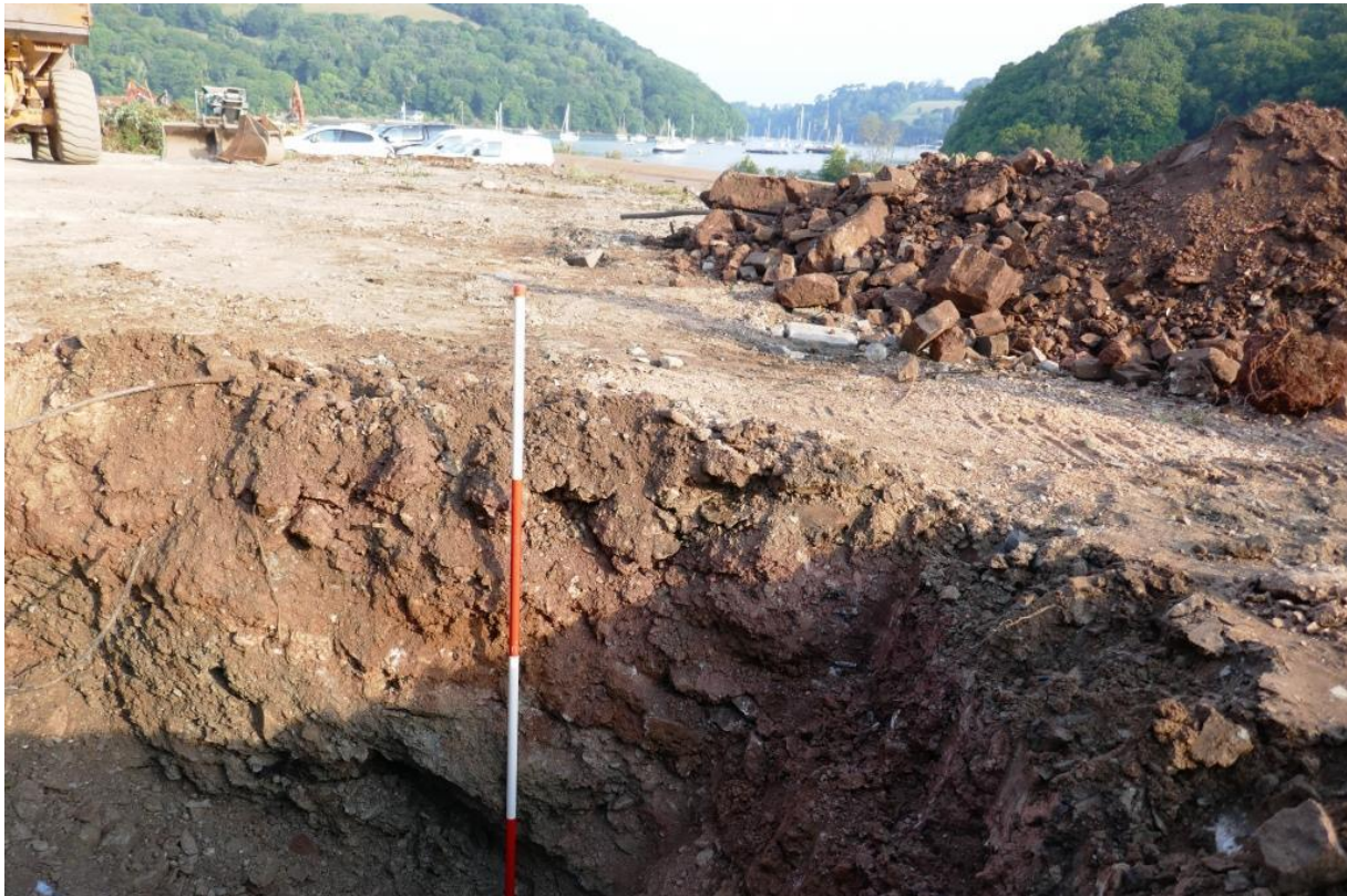
Fig 31 South facing section exposed by test pit east of centre of car park area, with layers of very stony infill (113) and (115) deposited from the south side in the 20th century to reclaim the ground from the creek beyond (2m scale).
