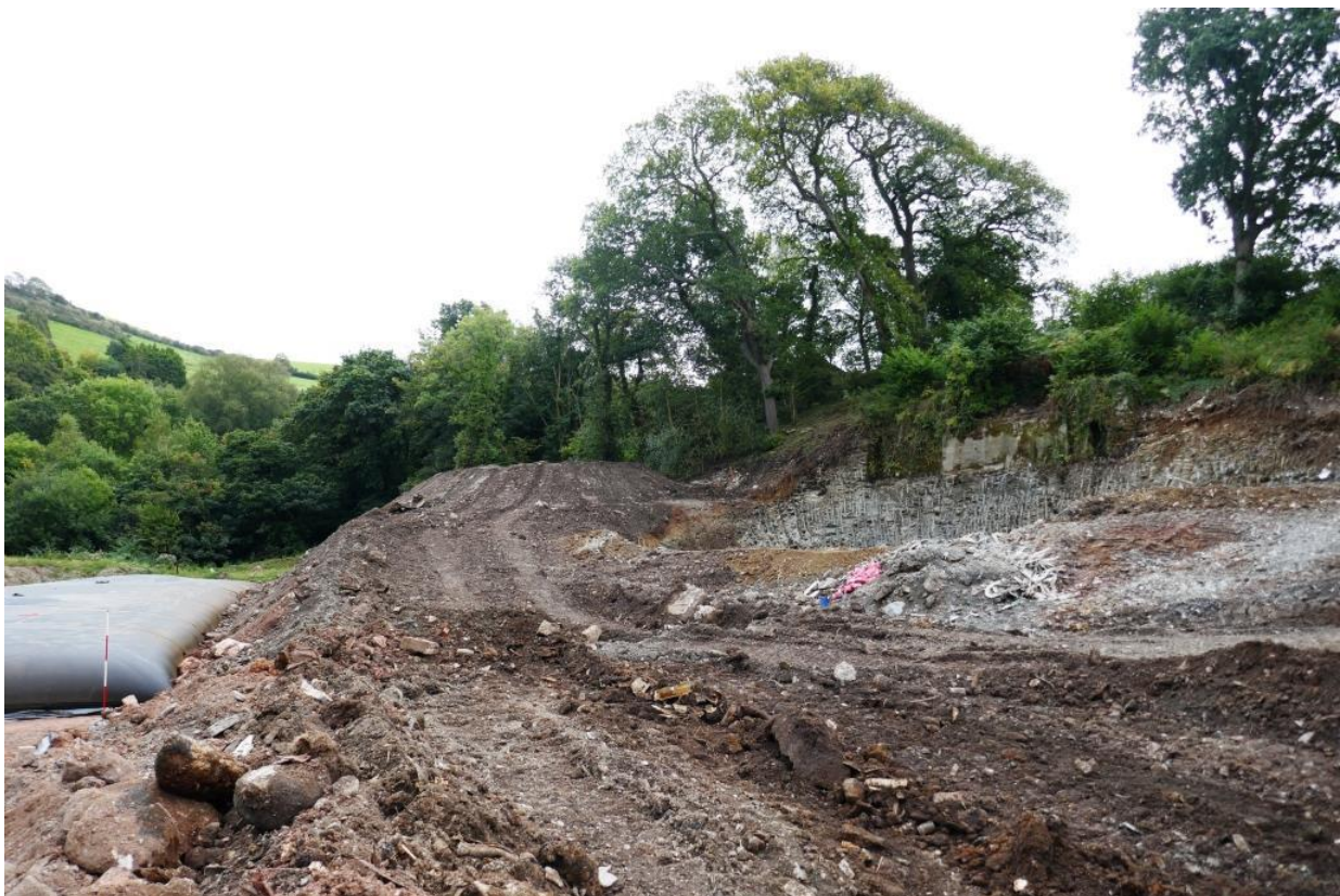
Fig 35 Site looking south east from silt storage area beside creek below, at conclusion of monitoring (2m scale).
