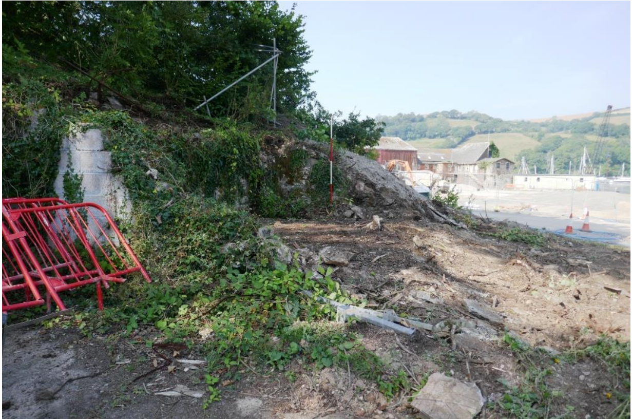
Fig 26 South west building at site 7 at start of works. Of its two roughly equal-sized parts, the nearer one appears relatively recent with concrete walls and floor 111; the further part appears modern though primary with narrow stone walls (2m scale).
