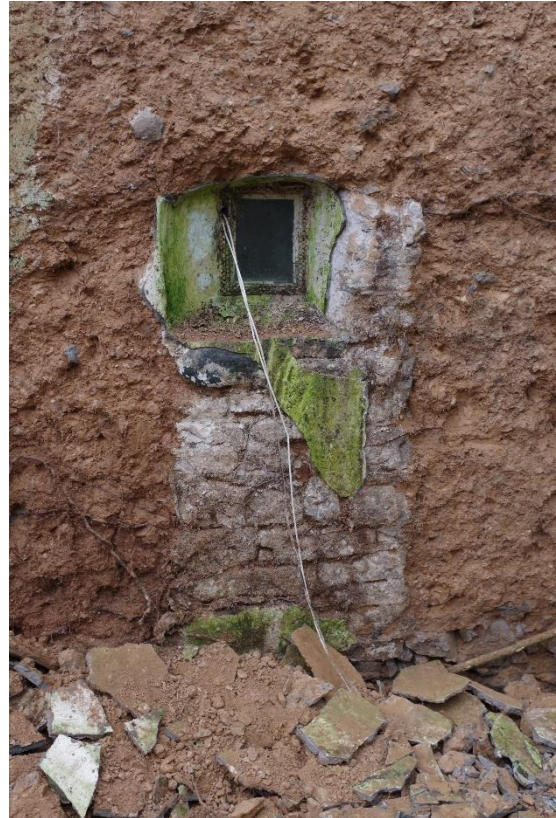
Fig 41 Blocked back door opening in north wall of phase 1 house.
