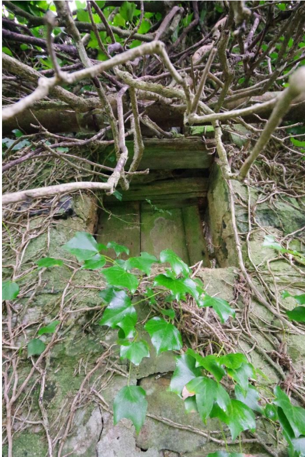
Fig 11 Small timber shuttered window opening in west elevation of phase 2 western extension.
