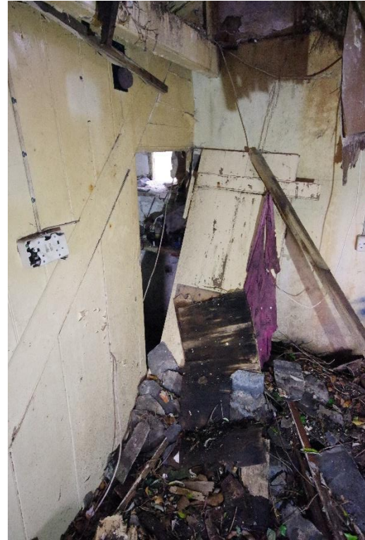
Fig 27 Room 4 door opening to Room 5 with detached door ledged door.
