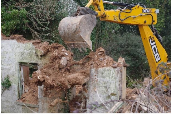
Fig 48 Mid demolition of front wall showing earth bonding in granite rubble wall.
