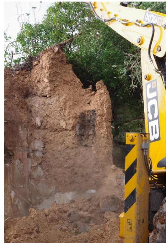
Fig 47 Blocking removed from fireplace in west wall of room 2, showing soot on cob.
