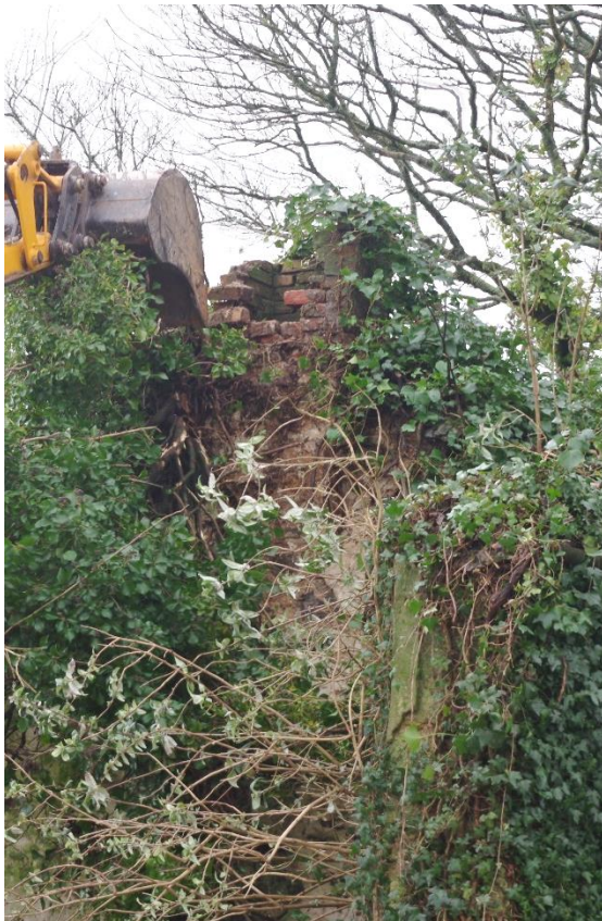
Fig 49 Demolition revealed a brick chimney stack in the west gable which had previously been obscured.
