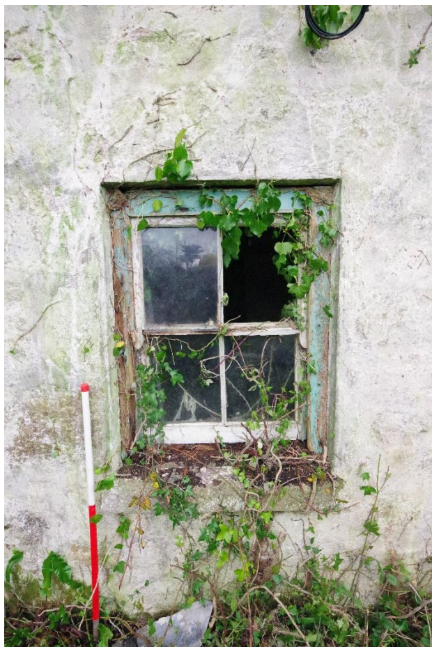
Fig 8 Early-mid 20th century replacement sash window to east of front door in south elevation.
