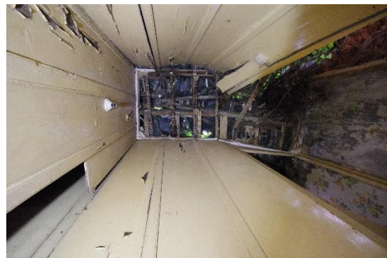
Fig 22 Room 3 plank and muntin partition walls enclosing the landing and stairwell at first floor level. looking upwards to exposed roof.
