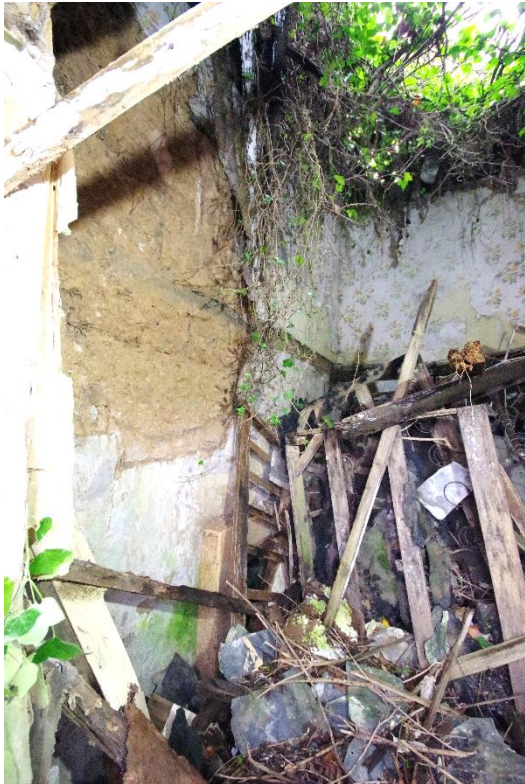
Fig 19 Room 2 north and west walls. Tiled fire surround just seen to left of collapsed timbers.
