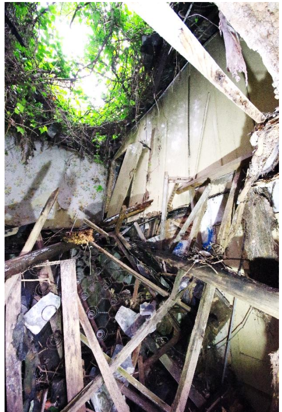
Fig 18 Room 2 north and east walls showing first floor plank and muntin partition wall to the east.
