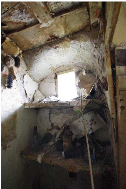
Fig 31 Room 5 blocked phase 1 door opening in north wall.
