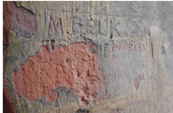
Fig 44 Detail of general graffiti on internal walls.
