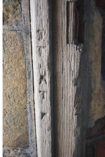
Fig 42 Detail of graffiti on door frame.
