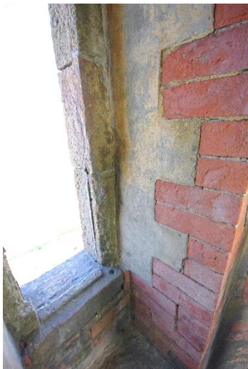
Fig 41 Detail of window reveal and elvan frame showing scars where the windows have been removed.
