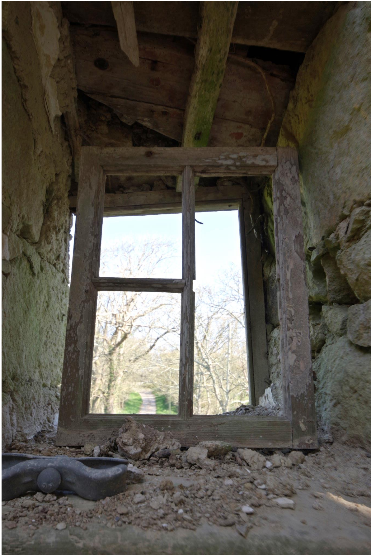
Fig 13 Remains of timber four-pane, fixed window at first floor level in north wall.
