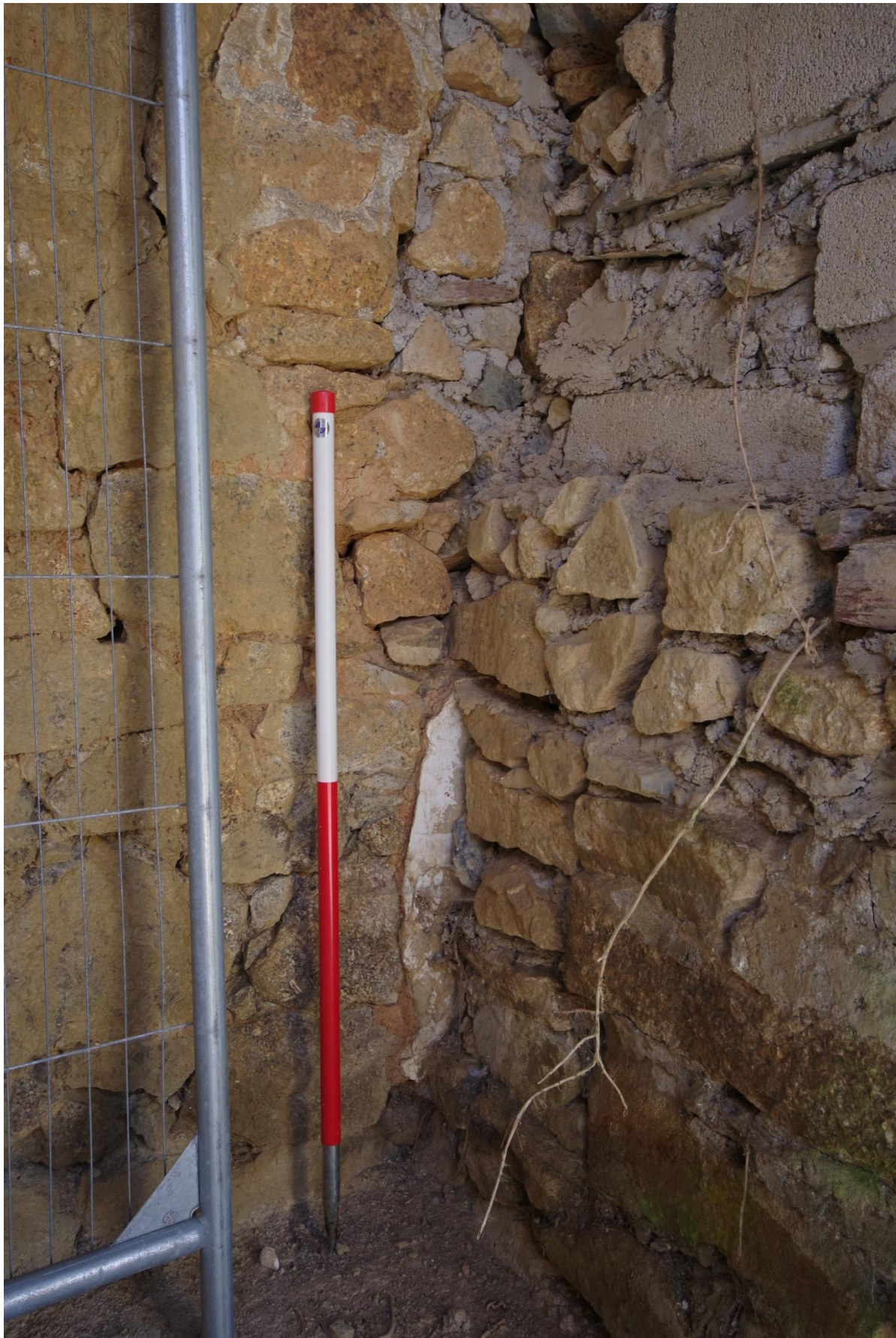
Fig 14 Showing the south wall (right) abutting the east wall (left) and covering the earlier plastered face of the east wall.
