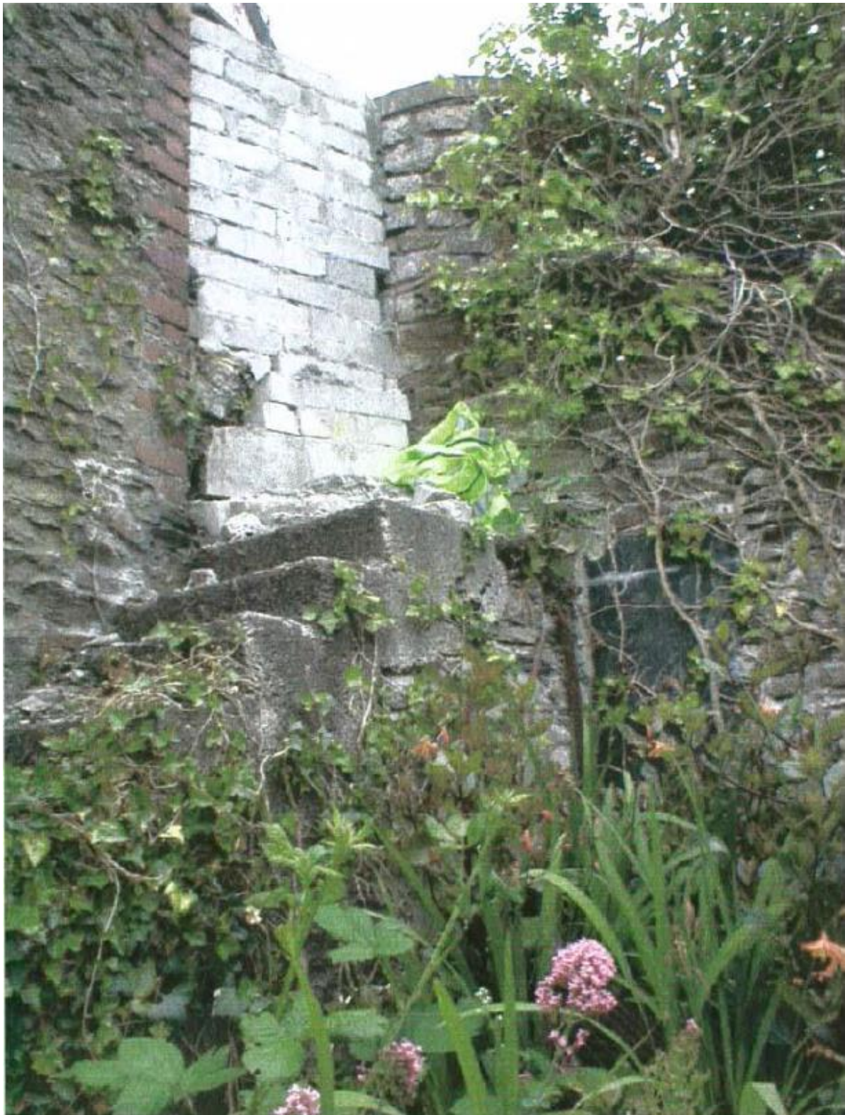
Fig 45 Section K west elevation, steps up to blocked gate opening to Shutta Road in 2003 (The Design & Maintenance Consultancy 2003b).
