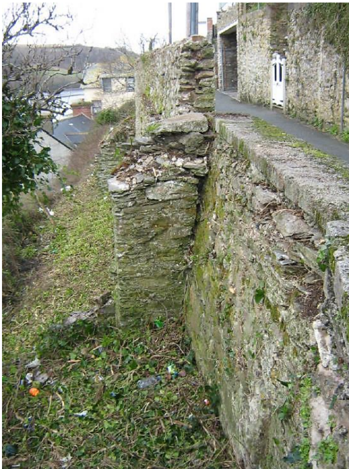
Fig 21 Section D west elevation before demolition, taken in 2008 (The Design & Maintenance Consultancy).
