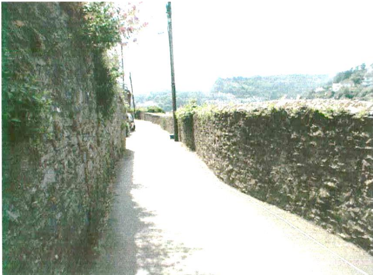
Fig 47 Section L in 2003 prior to demolition (The Design and Maintenance Consultancy 2003c).
