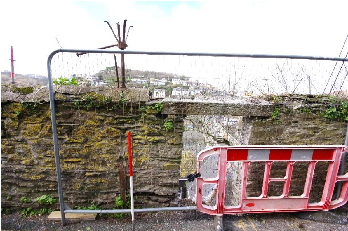
Fig 29 Section F north end and Section G south end of east elevation in March 2021 prior to demolition, showing iron gas lamp fitting.
