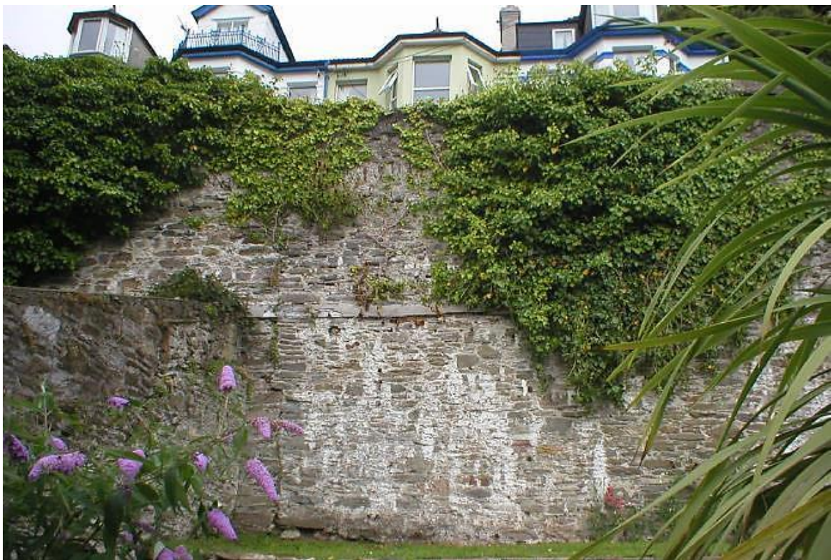
Fig 17 Section C west elevation in 2003 (The Design & Maintenance Consultancy 2003a) showing position of former building.
