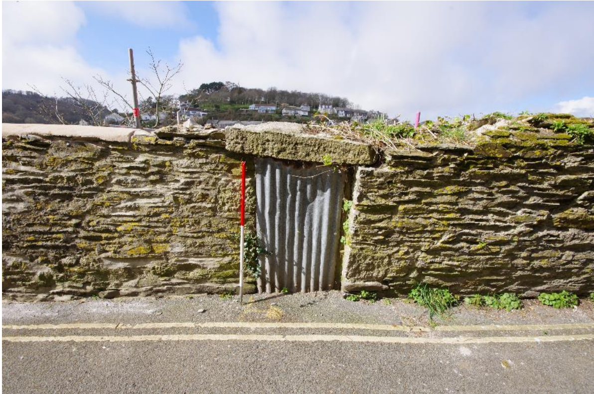
Fig 26 Section F east elevation of south end in March 2021 prior to demolition.
