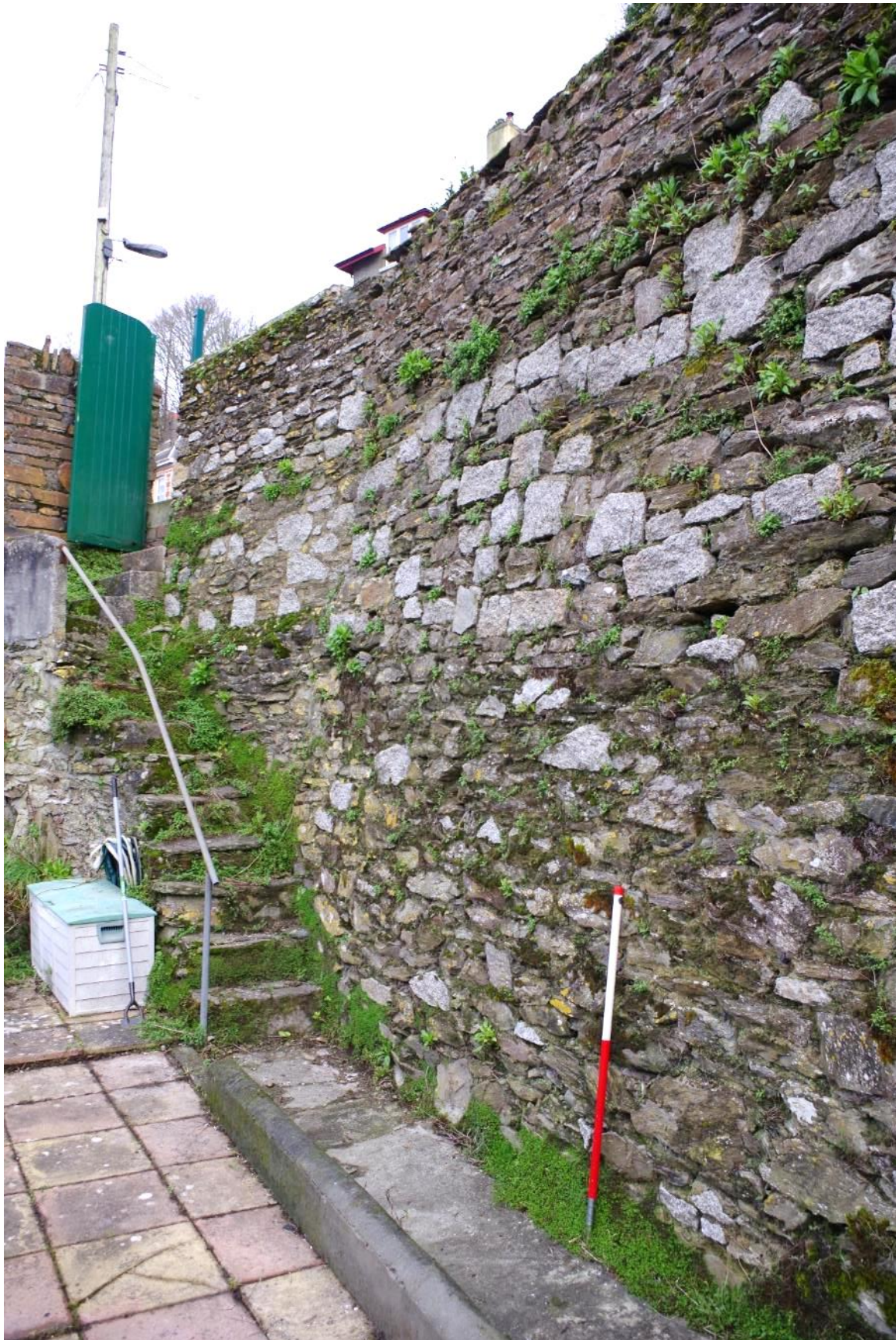
Fig 60 Sections O (right) and P (left), west elevations in January 2021 prior to erection of scaffolding.
