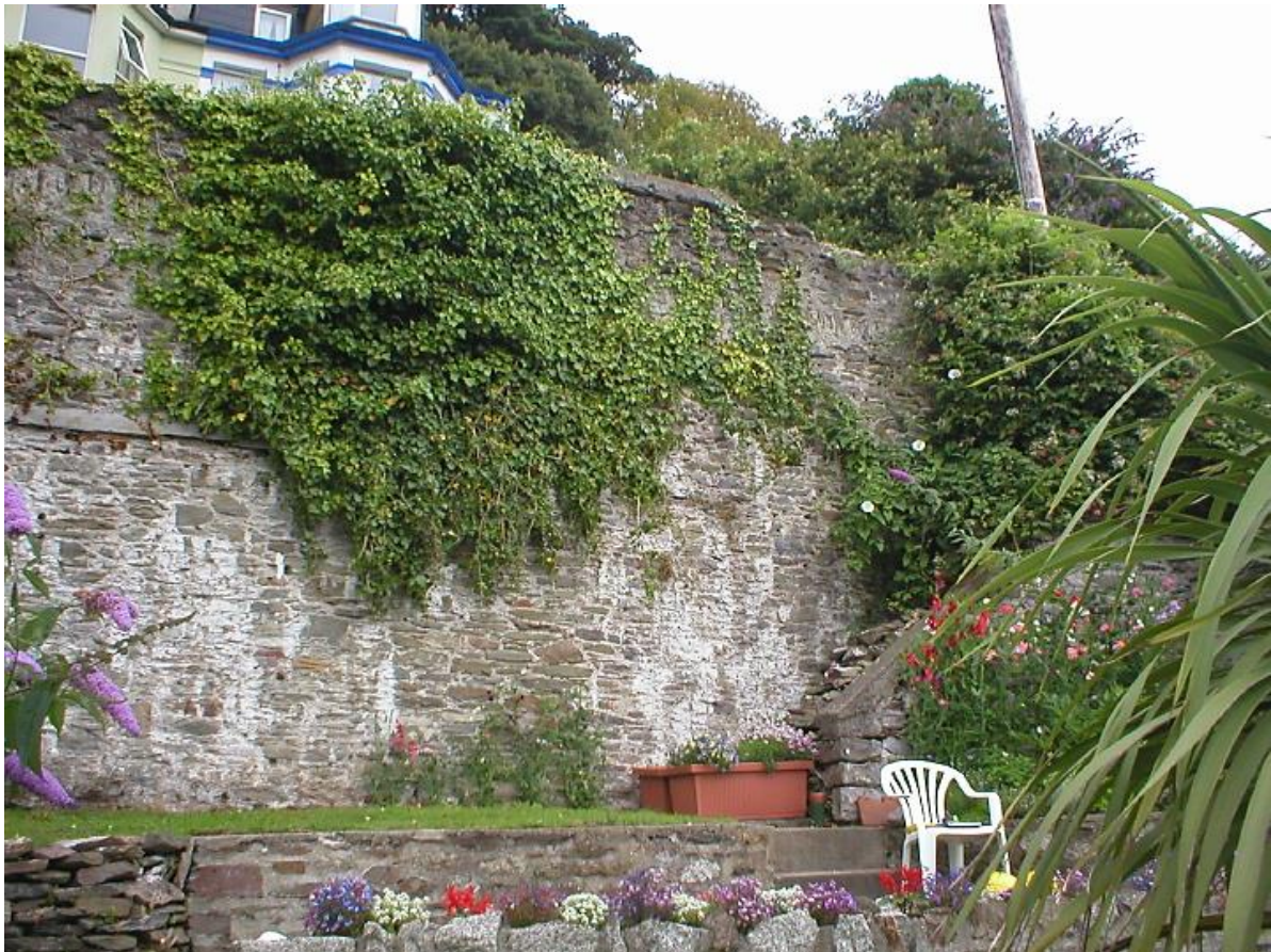
Fig 16 Section C west elevation in 2003 (The Design & Maintenance Consultancy 2003a) showing steps.
