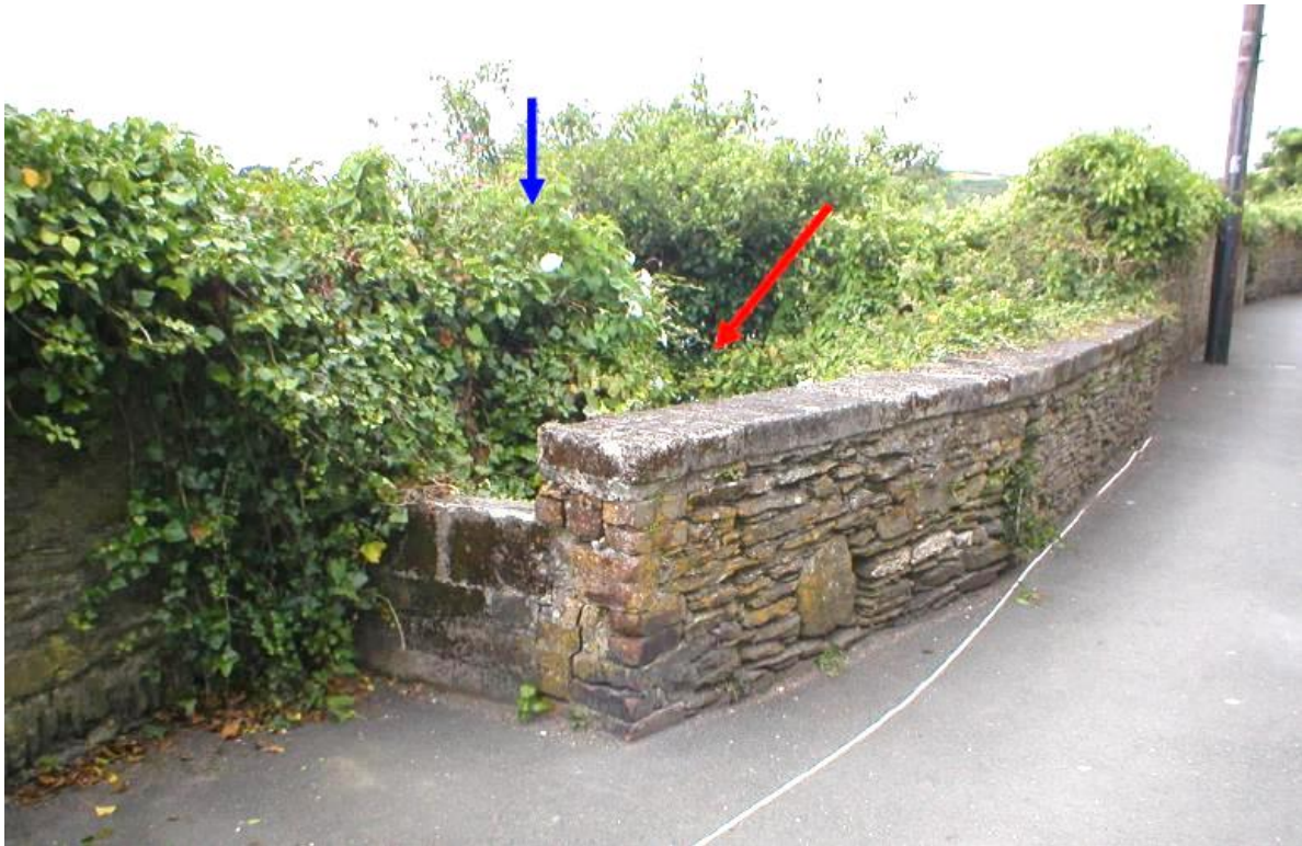
Fig 20 Section D prior to demolition, taken in 2003 (The Design & Maintenance Consultancy 2003a).
