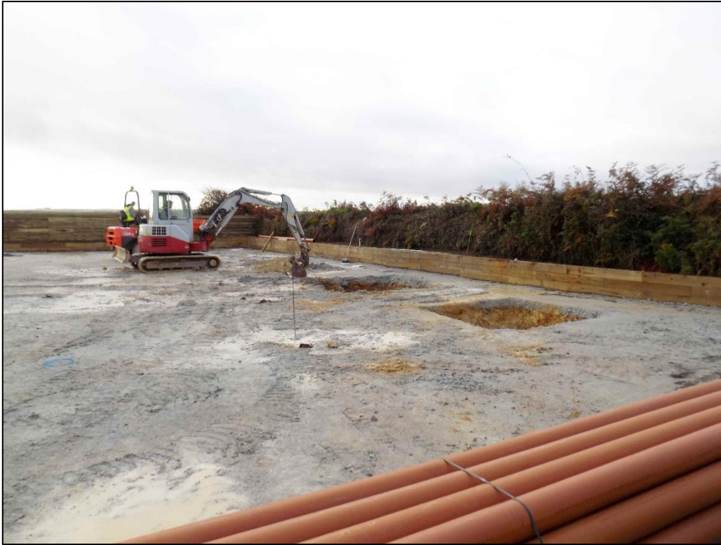
Fig 11 Bolt box pits being excavated on the west side of the site, looking south.
