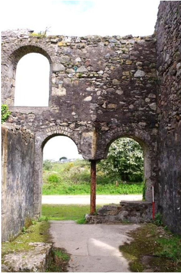
Fig 76 Room 9 north wall showing iron pipe reused as pillar to replace former window and door jambs. Room 10 is at first floor level.
