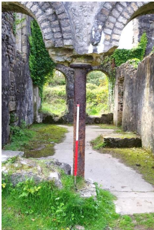
Fig 11 North elevation, east end showing reused iron pipe for missing window and door jambs.
