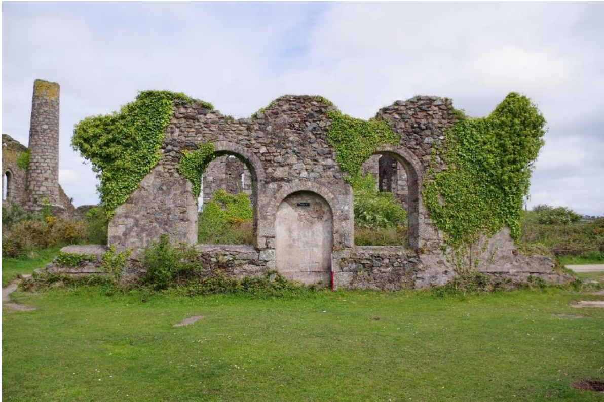
Fig 52 Room 5 north wall, extant central section showing original door opening now blocked.
