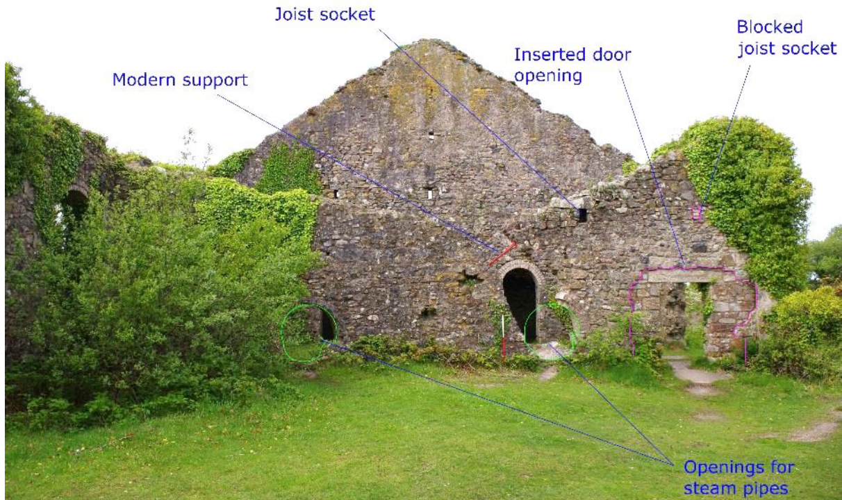
Fig 58 Room 5 west wall before repairs.
