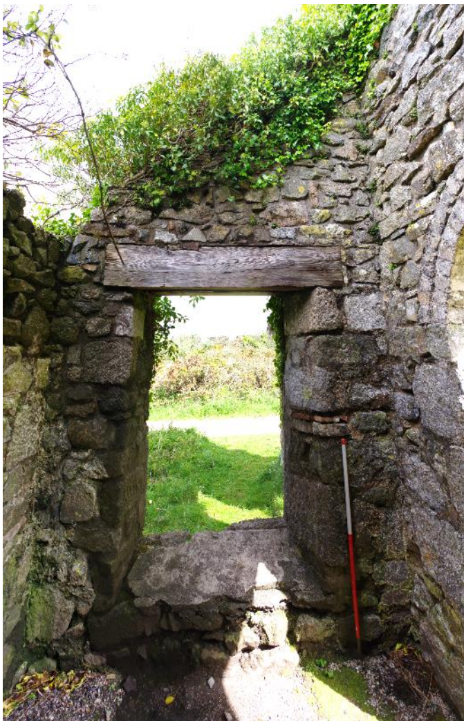
Fig 35 Room 3 north wall before repairs.
