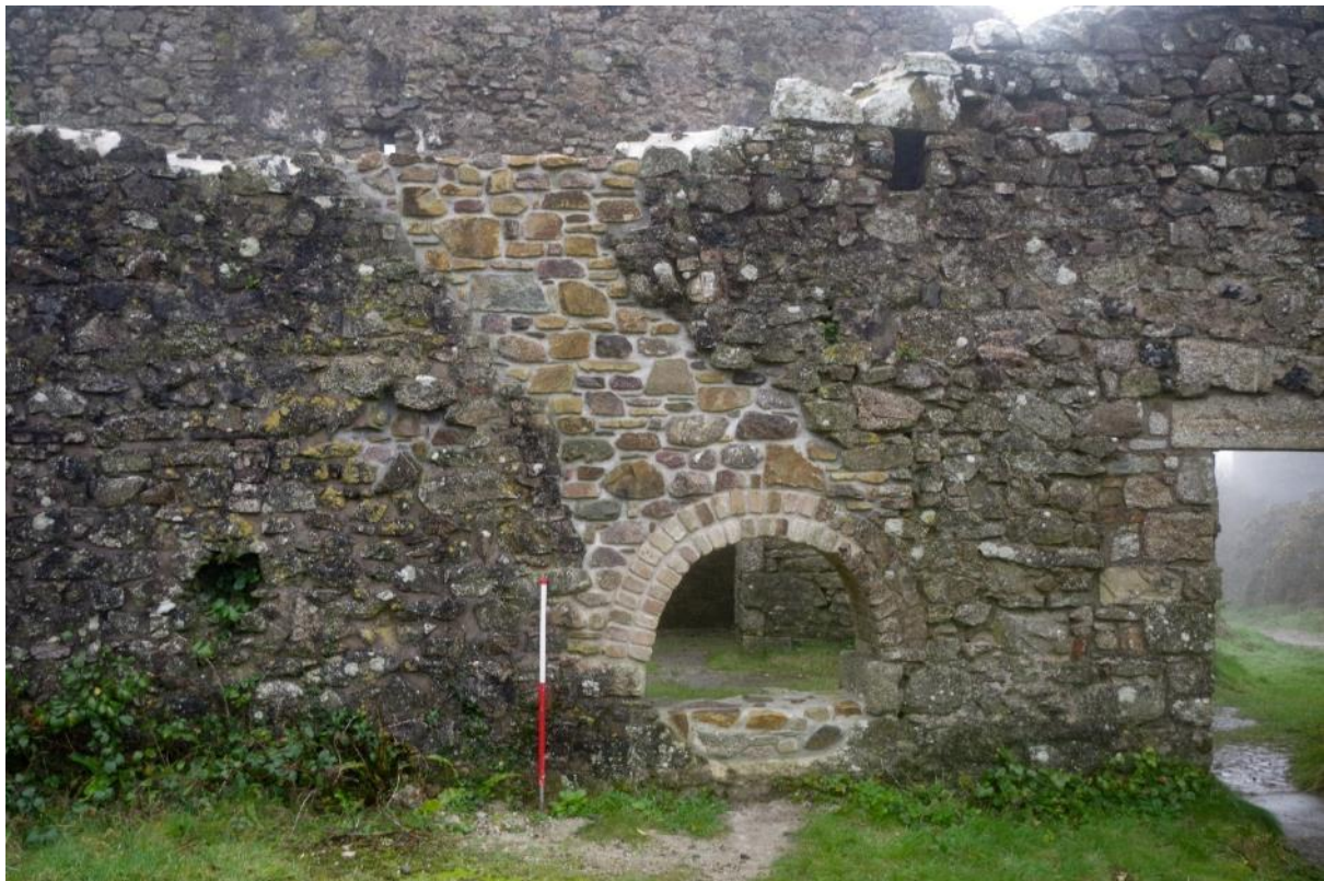
Fig 59 Room 5 west wall following reconstruction of missing wall and brick arch for northern steam pipe opening.
