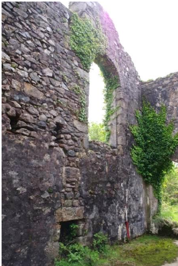
Fig 79 Room 9 east wall looking southeast, with loading door opening into room 10 at first floor level.
