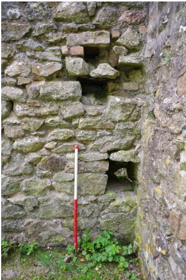
Fig 47 Room 4 east wall, blocked openings for pipework at southern end of wall.
