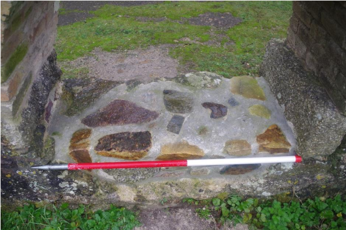
Fig 60 Room 5 west wall following repair to the base of the northern steam pipe opening.
