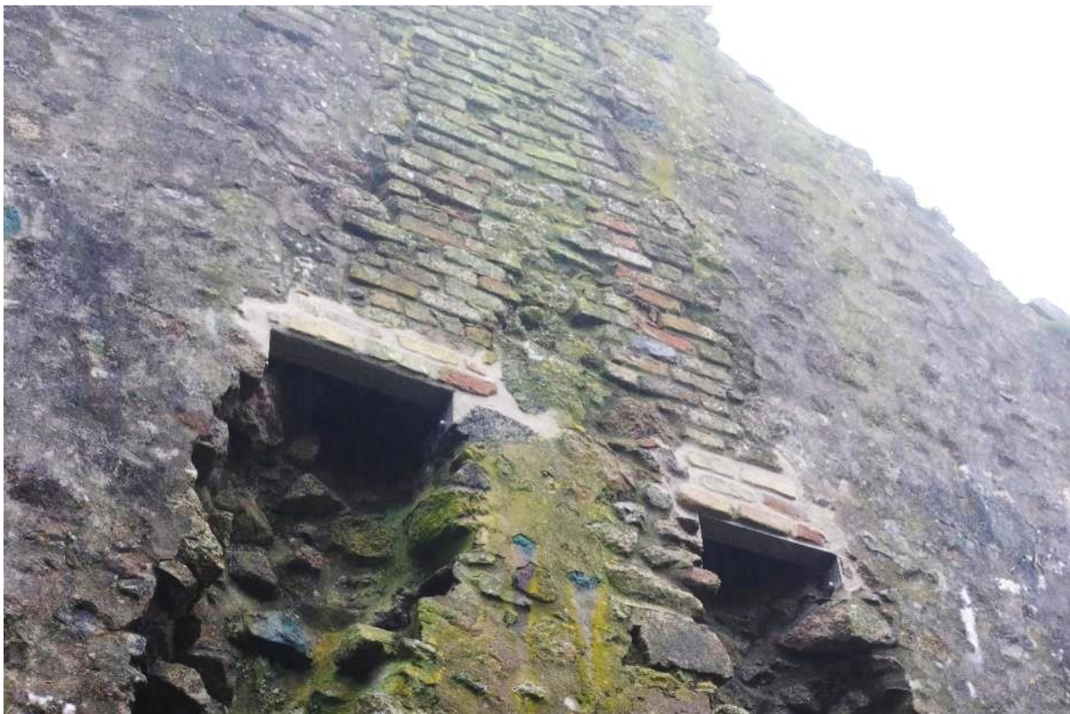
Fig 85 Room 10 following repairs to the brickwork of the flues in the west wall.
