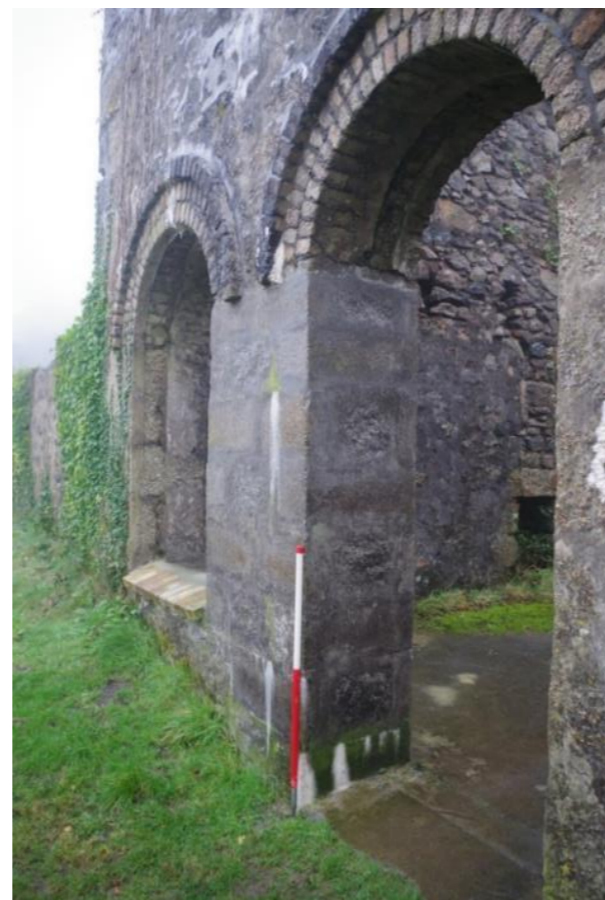
Fig 12 North elevation, east end following repairs, showing rebuilt window and door jambs around iron pipe.
