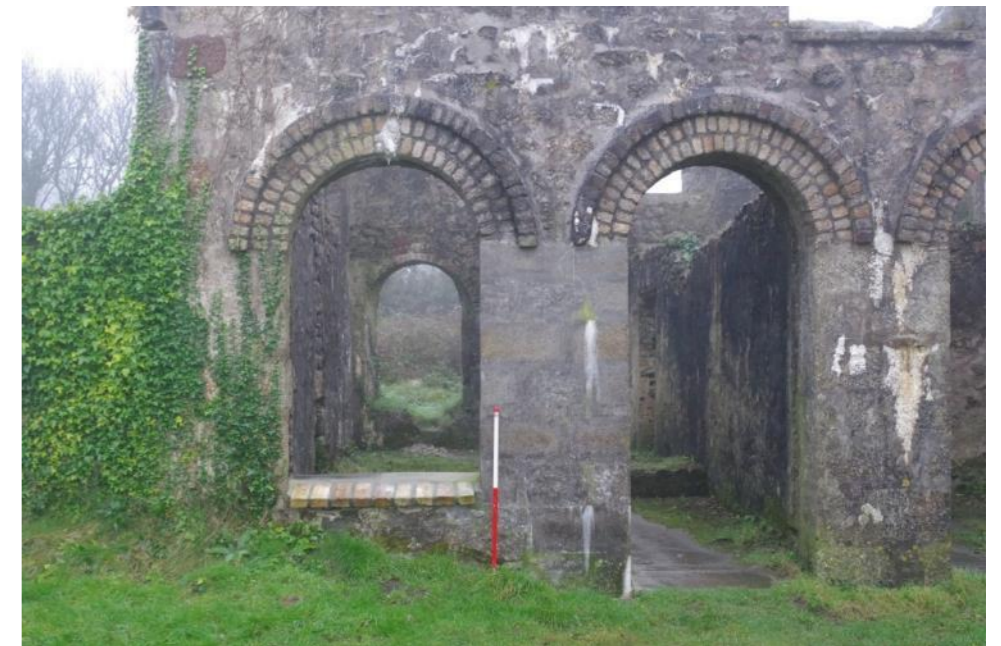
Fig 13 North elevation, east end following repairs, showing rebuilt window and door jambs around iron pipe and new brick sill.
