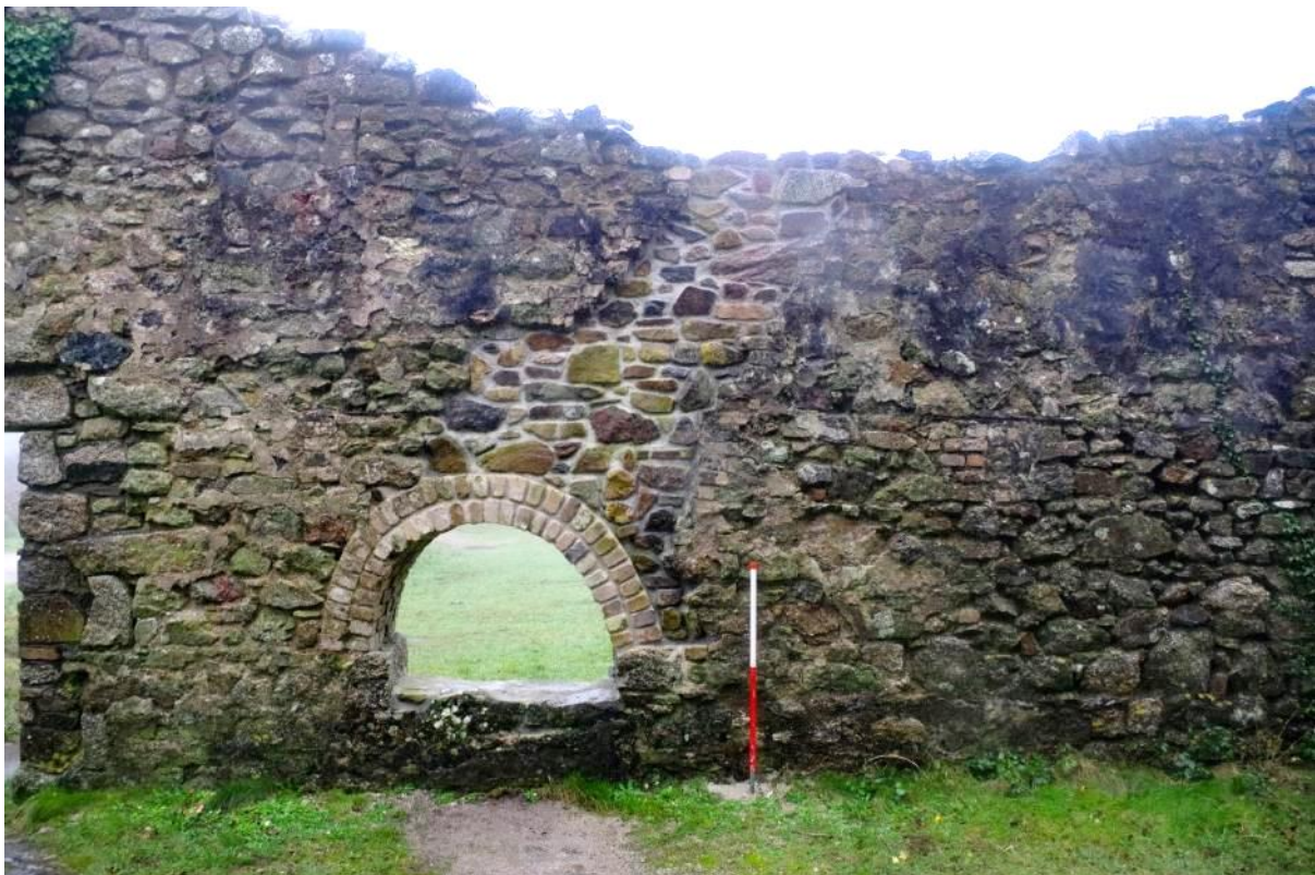
Fig 45 Room 4 east wall following reconstruction of missing wall and brick arch for northern steam pipe opening.
