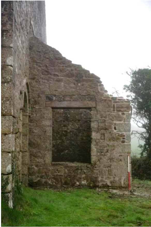
Fig 22 North exterior elevation of Room 3 following repair of the quoin and lintel.
