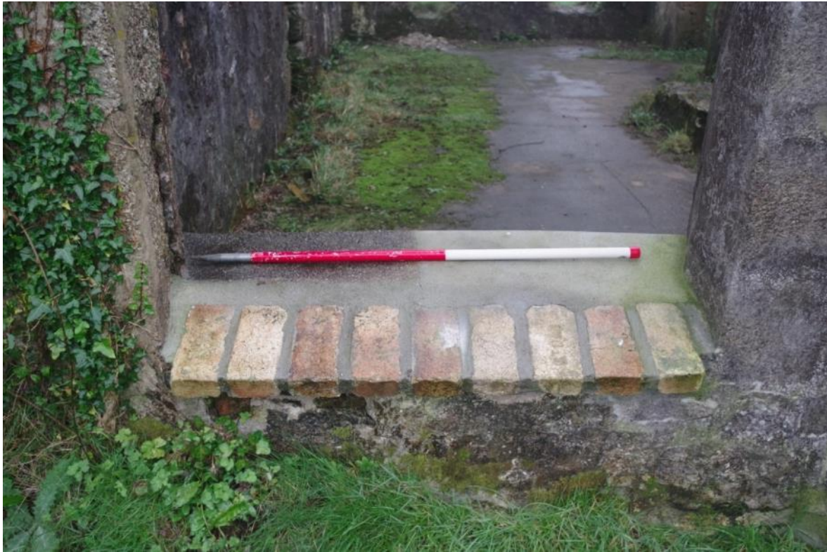
Fig 14 North elevation, east end following repairs to the window sill of room 9.
