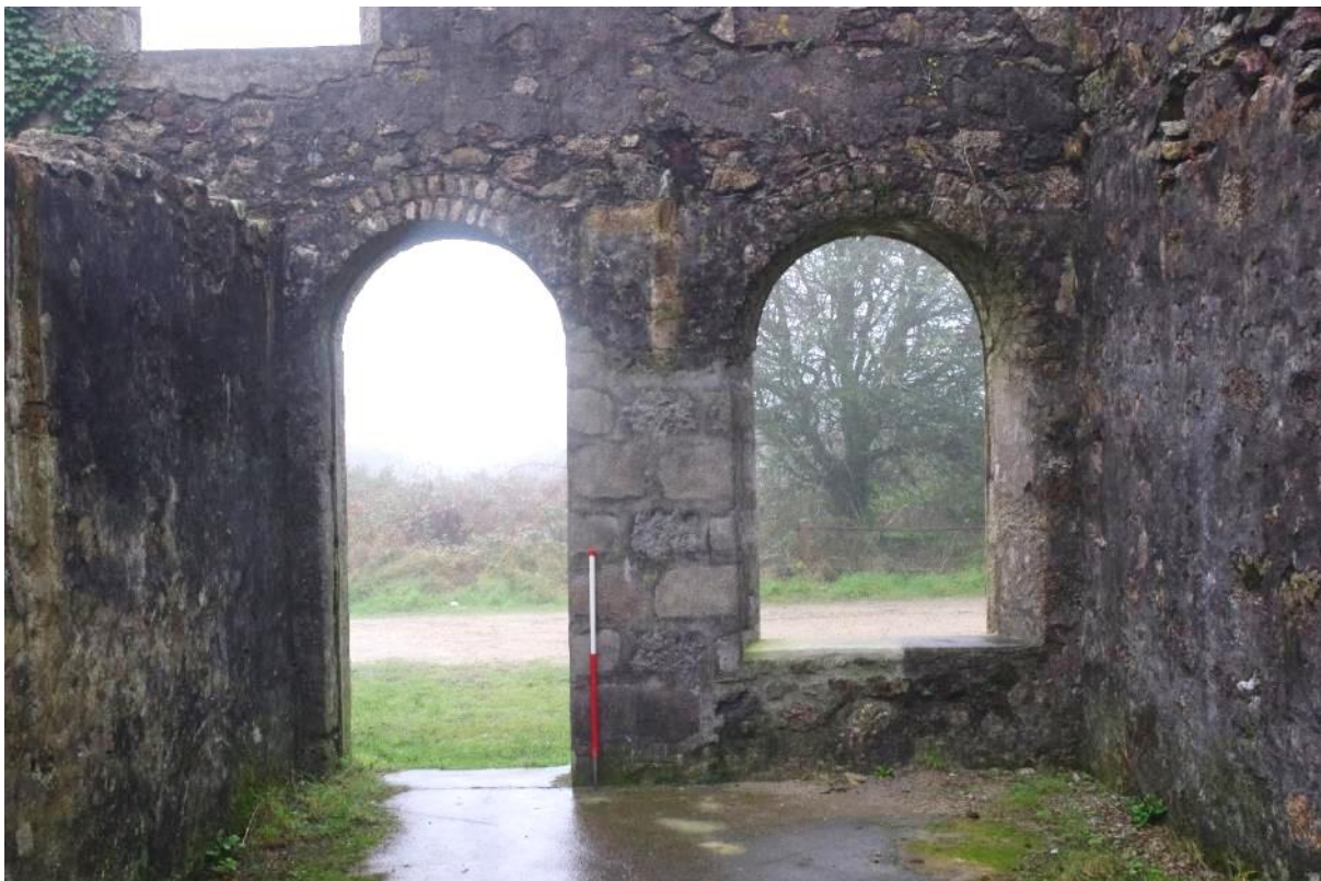
Fig 77 Room 9, north wall following repairs and showing rebuilt jambs around iron pipe.
