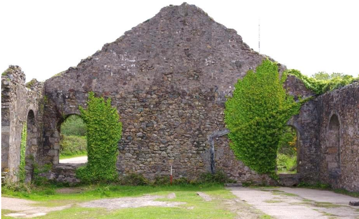
Fig 54 Room 5 east wall, showing location of former, inserted phase 3 lean-to to the right.
