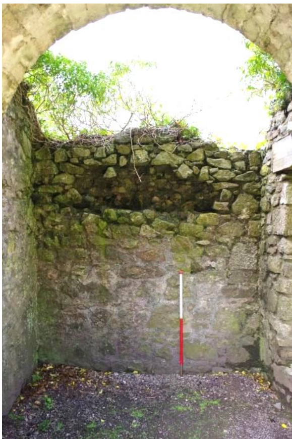
Fig 39 Room 3 west wall before repairs.
