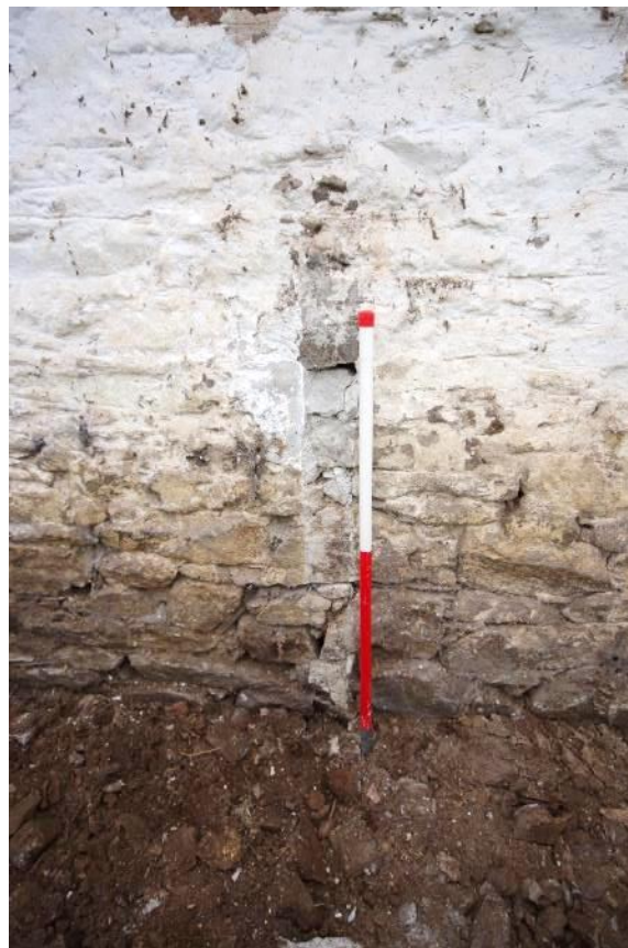
Fig 44 Southeast wall showing the position of the removed concrete block-built partition wall and an earlier rail socket (blocked with cement mortar).
