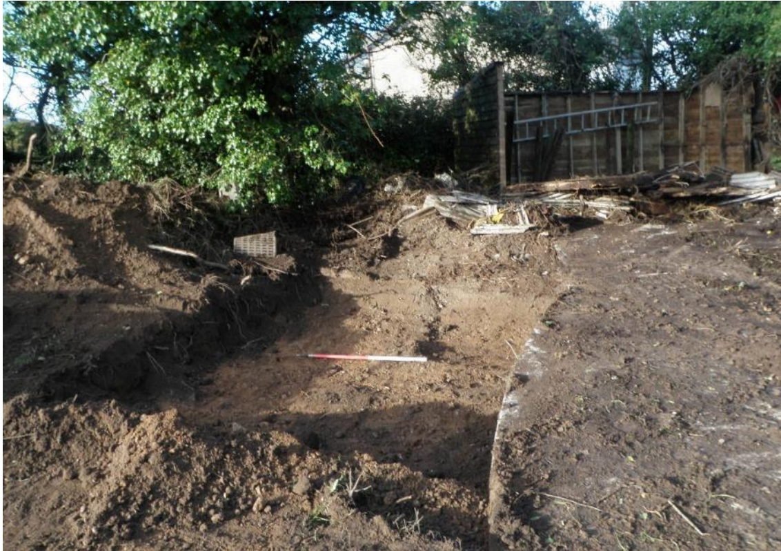
Fig 16: showing the attenuation tank during stripping. Note the concrete hard-core and collapsing shed, which required a change in the planned for tank's alignment.
