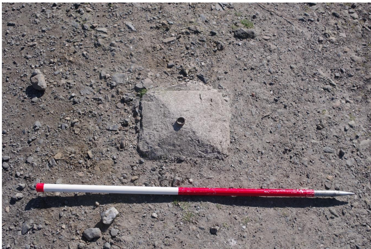
Fig 29 Metal fitting in the track surface.
