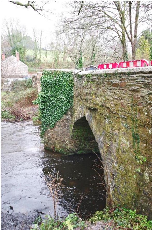
Fig 17 (07) South end of the west elevation showing pushed out parapet wall.
