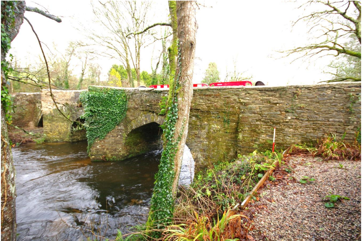
Fig 13 (05) Southern part of the west elevation showing pushed out walling over the arch and straight joint to the right.
