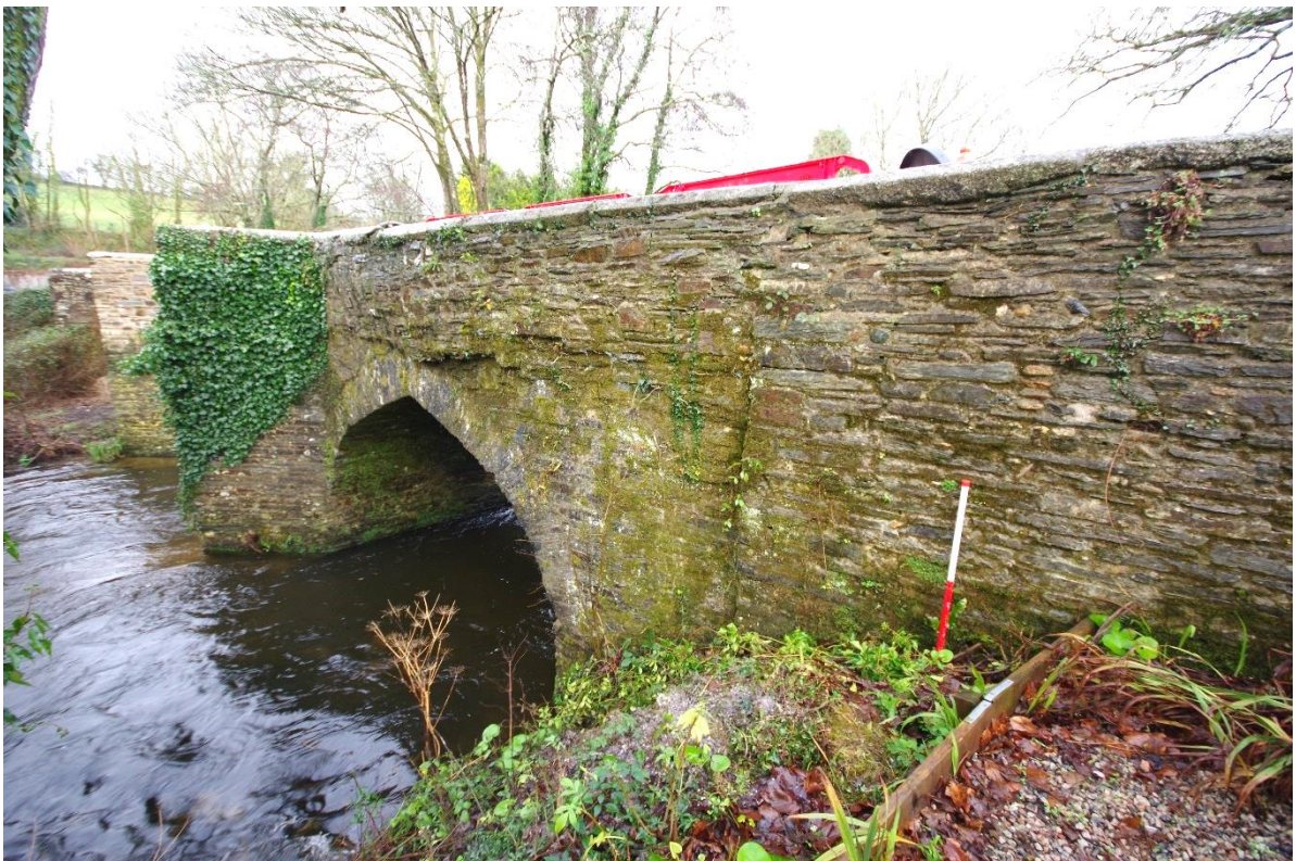
Fig 16 (01) South end of the west elevation showing pushed out walling over the arch.
