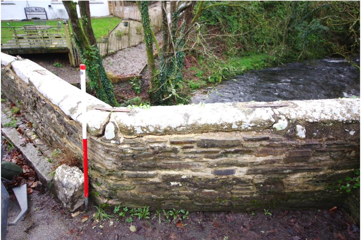
Fig 25 (31) Recently repaired (2021) parapet wall in the refuge immediately north of the damaged area.
