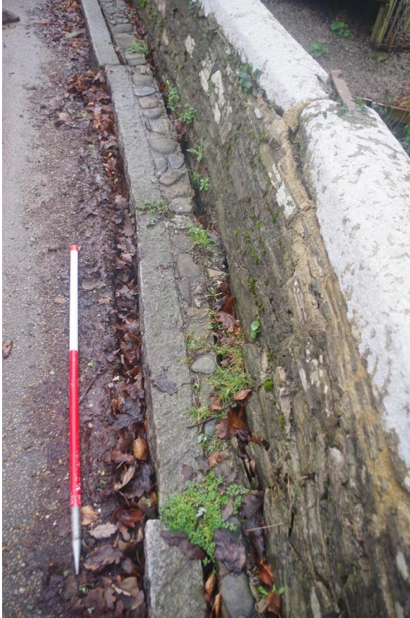
Fig 19 Gaps created by the collision on either side of the modern kerbing adjacent to the pushed out parapet wall.
