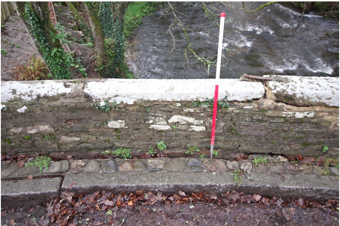
Fig 22 (25) East elevation of the damaged area of parapet wall immediately north of Figure 21.
