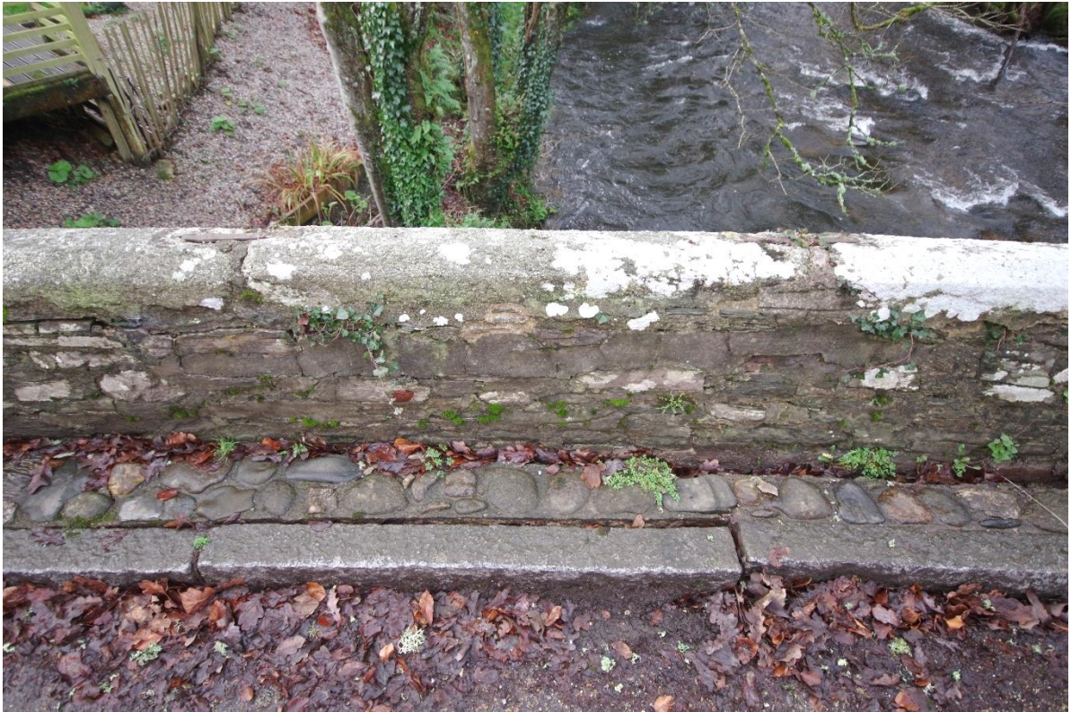
Fig 21 (24) East elevation of the damaged area of parapet wall immediately north of Figure 20.
