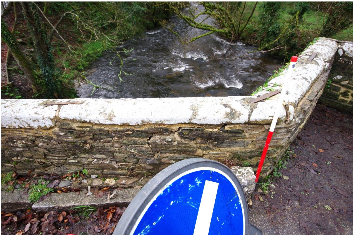
Fig 24 (28) East elevation of the damaged area of parapet wall immediately north of Figure 23.
