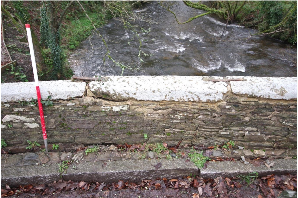
Fig 23 (26) East elevation of the damaged area of parapet wall immediately north of Figure 22.
