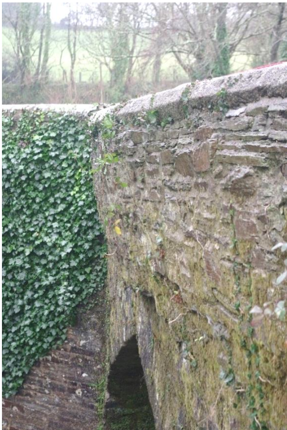
Fig 18 (10) Close up of pushed out parapet wall.
