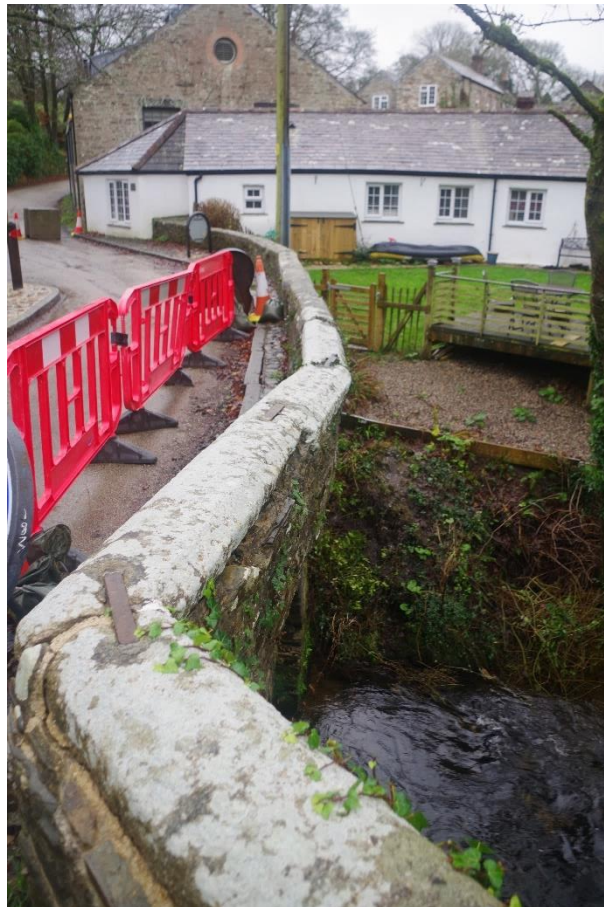
Fig 26 (14) View looking south along the top of the damaged parapet wall.
