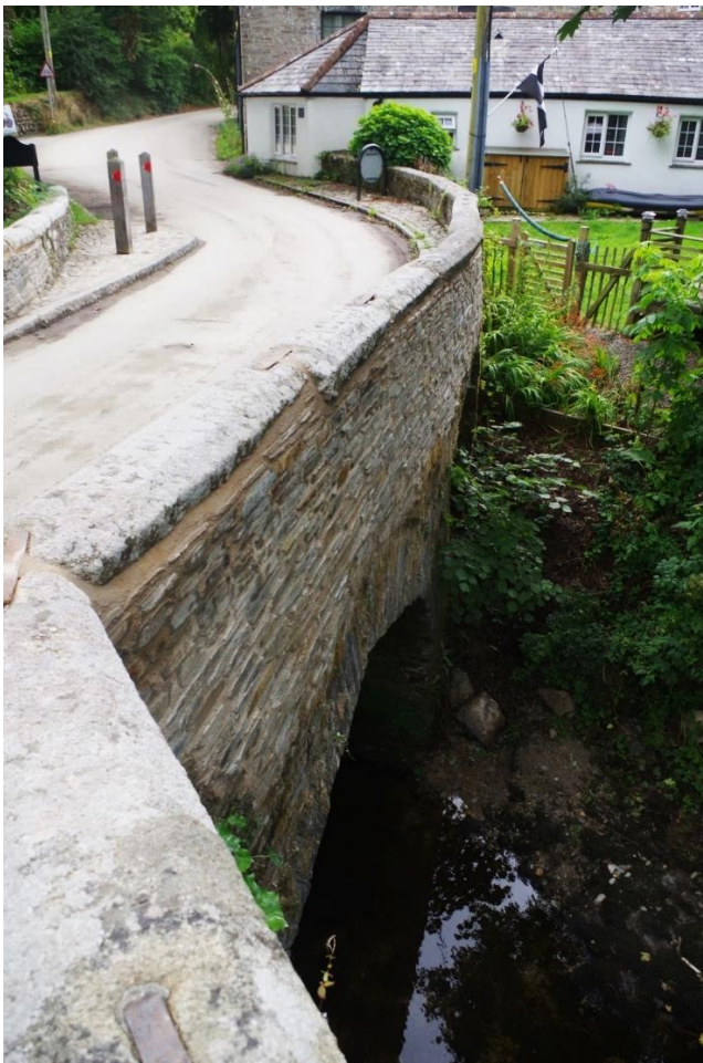
Fig 36 (43) West elevation of new parapet and spandrel wall following reconstruction looking south.
