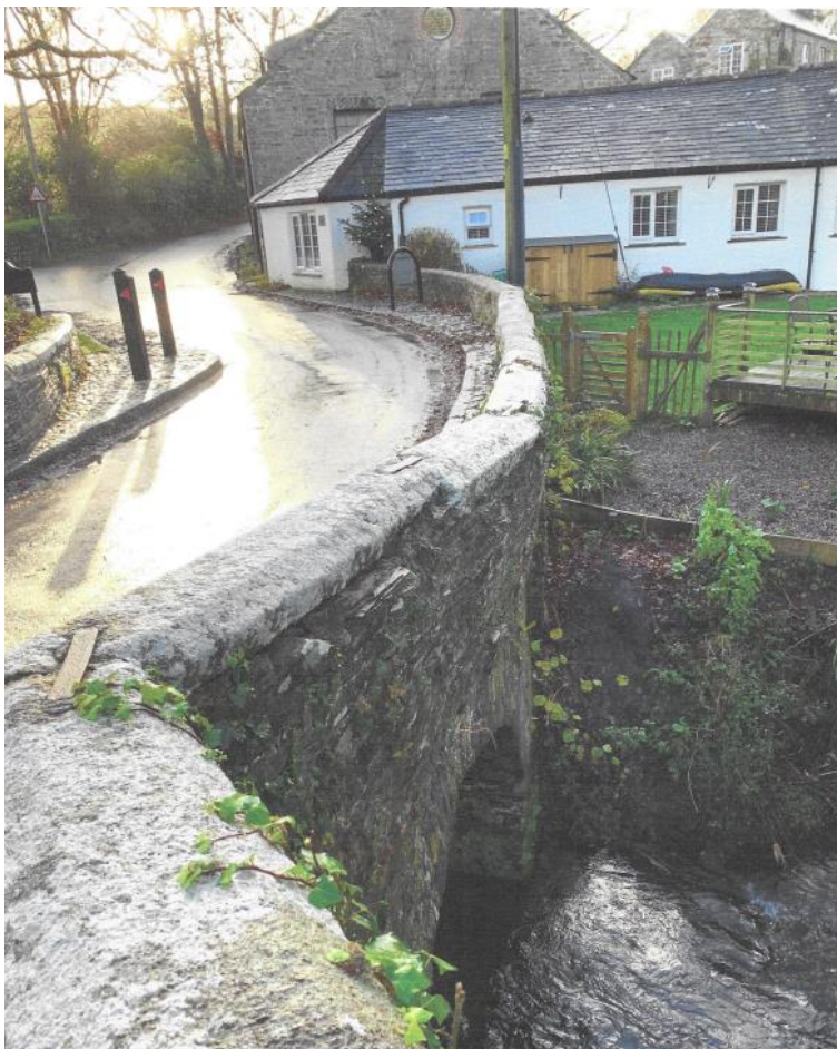
Figure 4 Photograph of recent damage, looking south along the western side of the bridge showing the parapet and walling below pushed outwards.
