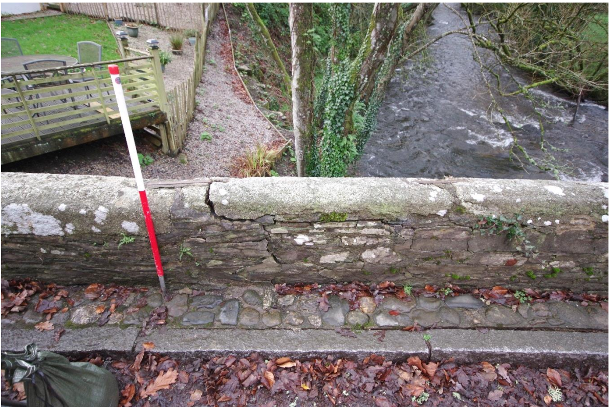
Fig 20 (23) Southern end of the east elevation of the damaged area of parapet wall.
