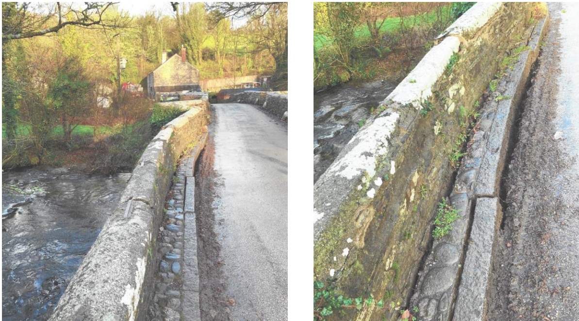
Figure 3 Photographs of recent damage, looking north along the western side of the bridge.
