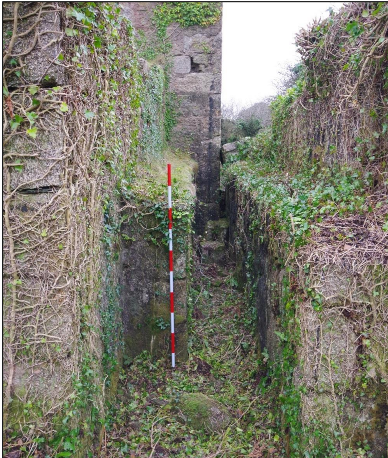
Fig 13 View of flywheel slot in loadings before remedial works.
