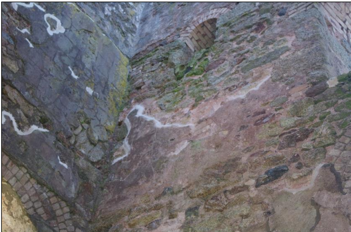
Fig 26 Interior north-west wall following small patch repair around edges of incised plaster.
