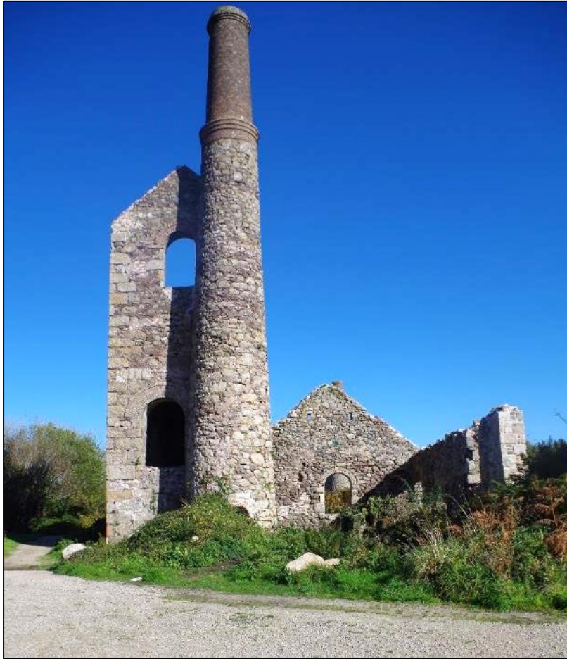
Fig 51 South-west elevation of the engine house following ivy clearance, patch repairs and capping of gable ends.
