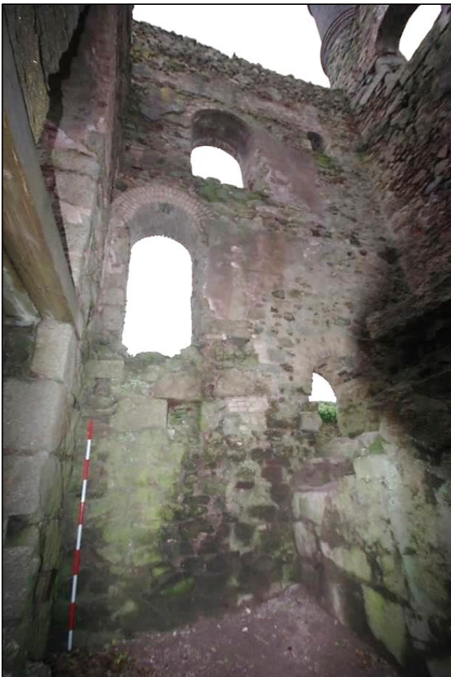
Fig 38 Interior south-east wall before remedial works.
