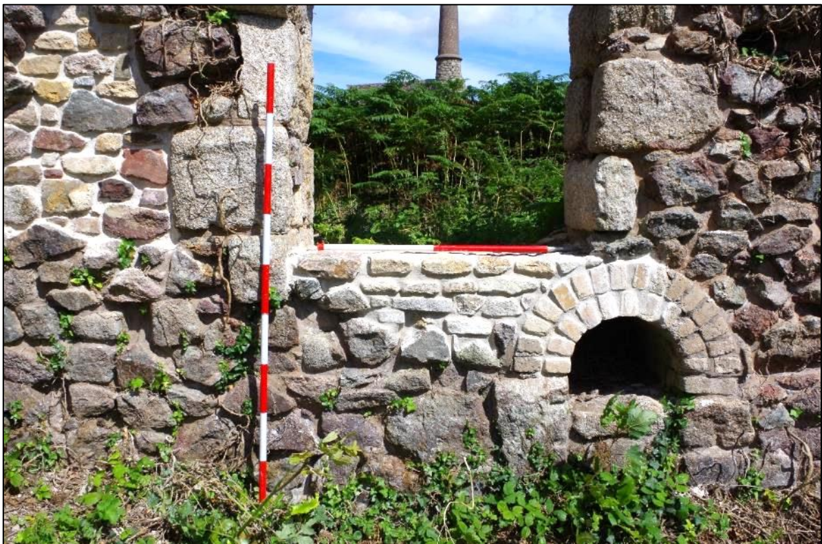
Fig 64 Interior south-west wall of boiler house following patch repairs to wall and arch.
