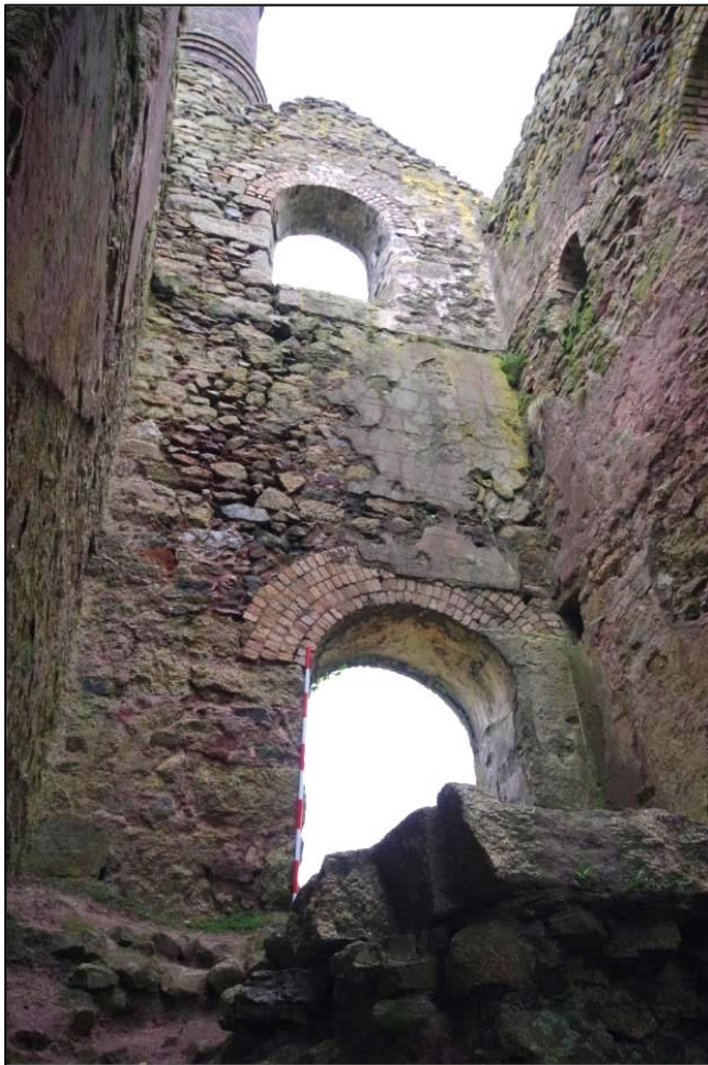
Fig 66 Interior south-west wall of engine house before remedial works.
