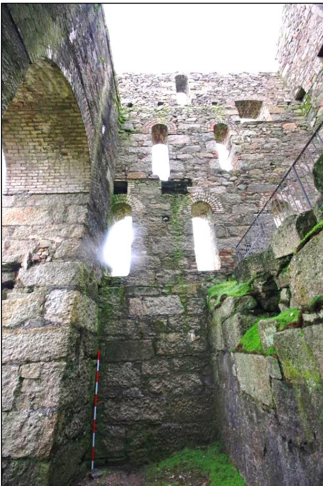
Fig 74 Interior north-east wall from the cataract pit before remedial works.
