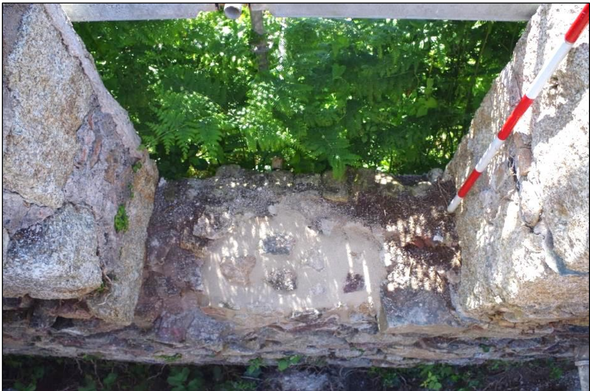
Fig 46 South-east wall of the boiler house following patch repair to window sill.
