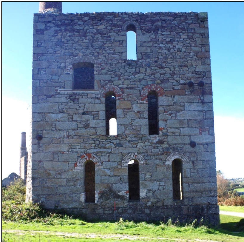
Fig 72 North-east elevation following the installation of a new lintel and repairs to window arches and jambs.
