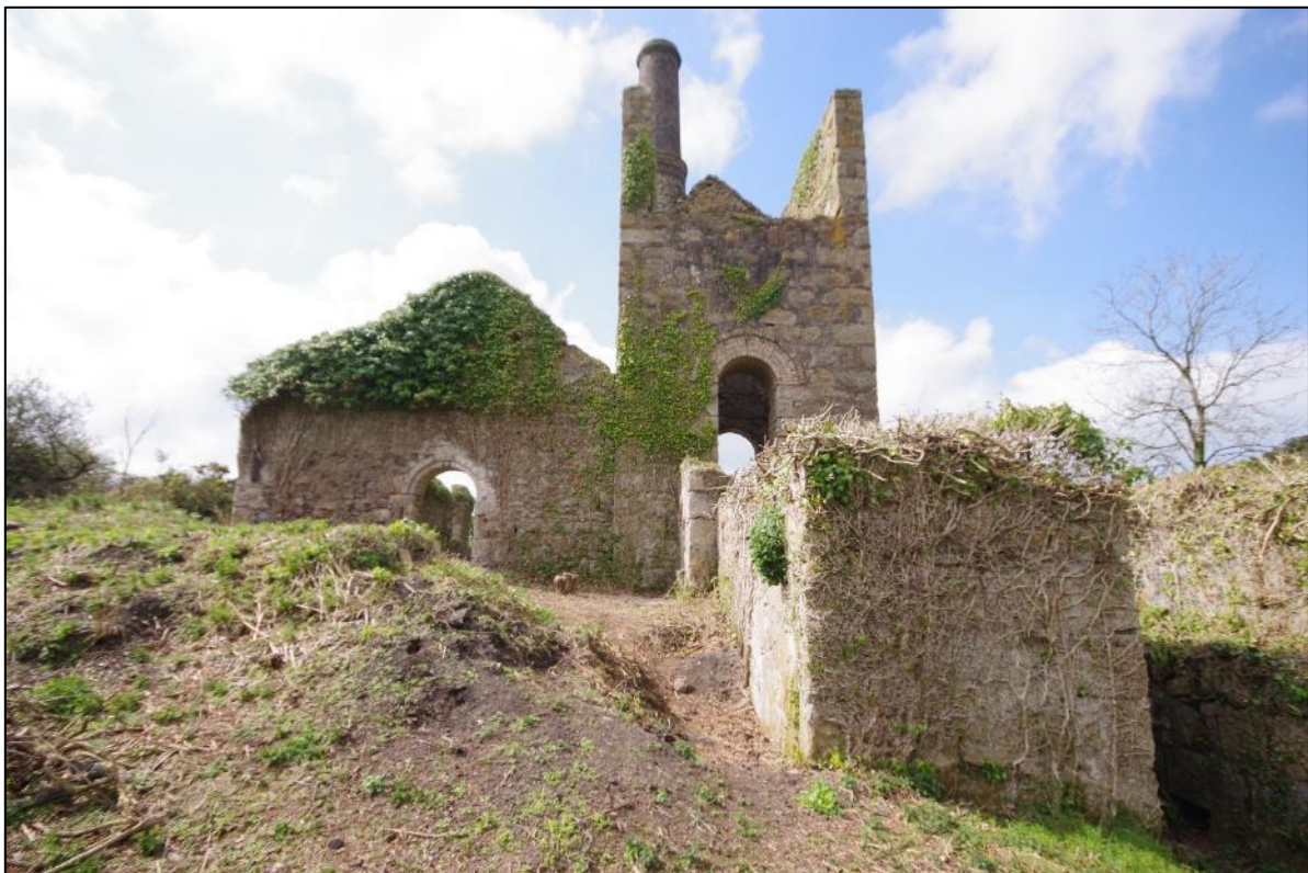
Fig 14 North-east elevation following vegetation clearance and repair work to the boiler house window opening.
