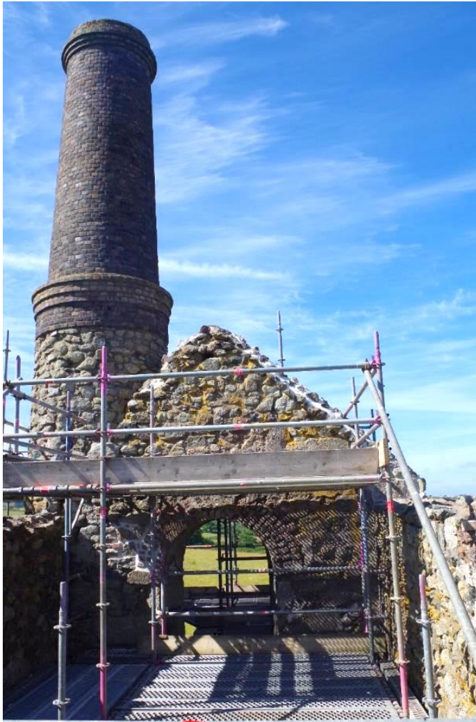
Fig 53 Interior south-west engine house wall following patch repairs and gable end capping.
