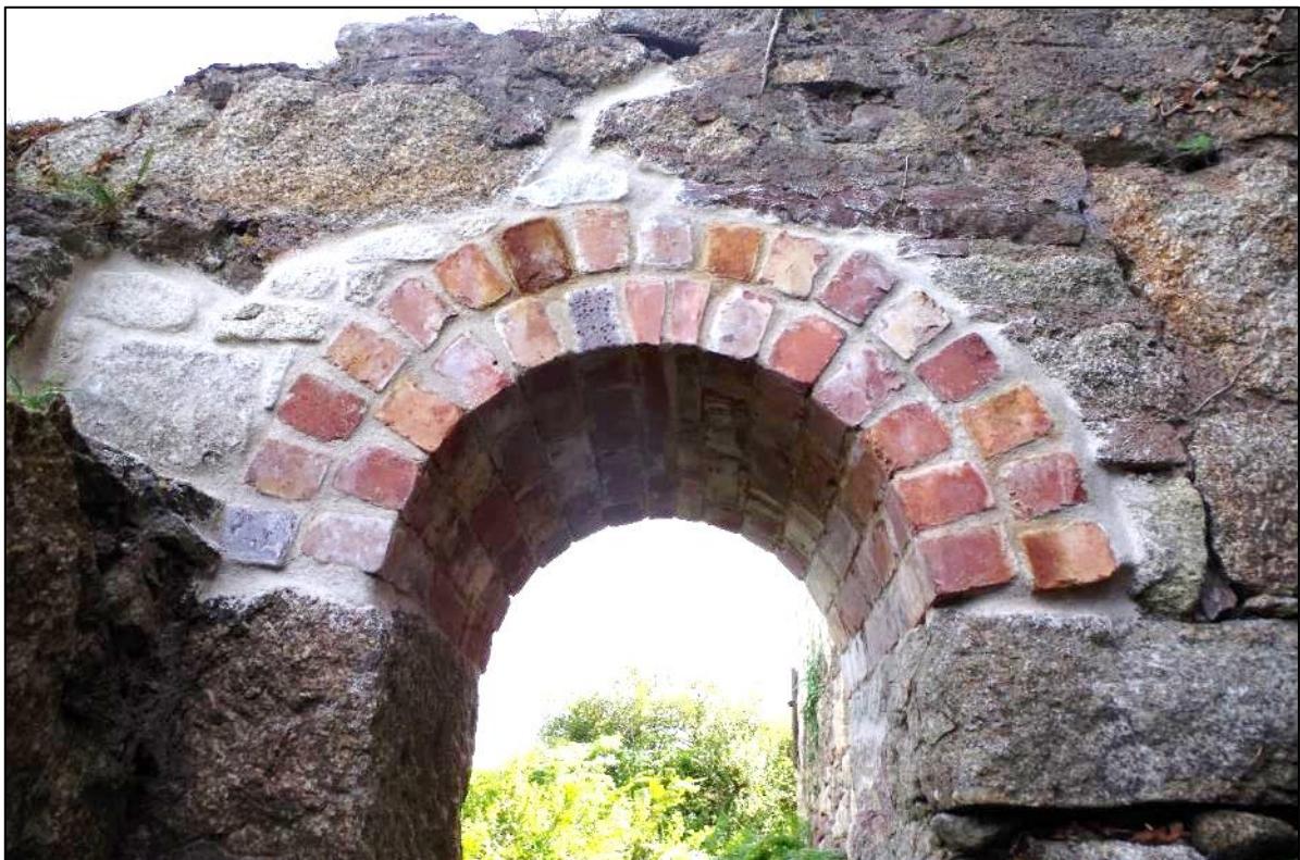
Fig 42 Interior south-east wall of the condenser pit showing repaired arch over opening.
