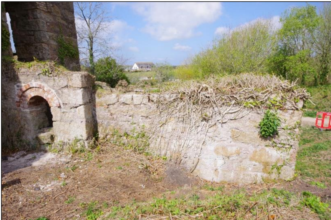
Fig 36 South-east elevation of the loadings following patch repairs and some ivy clearance.
