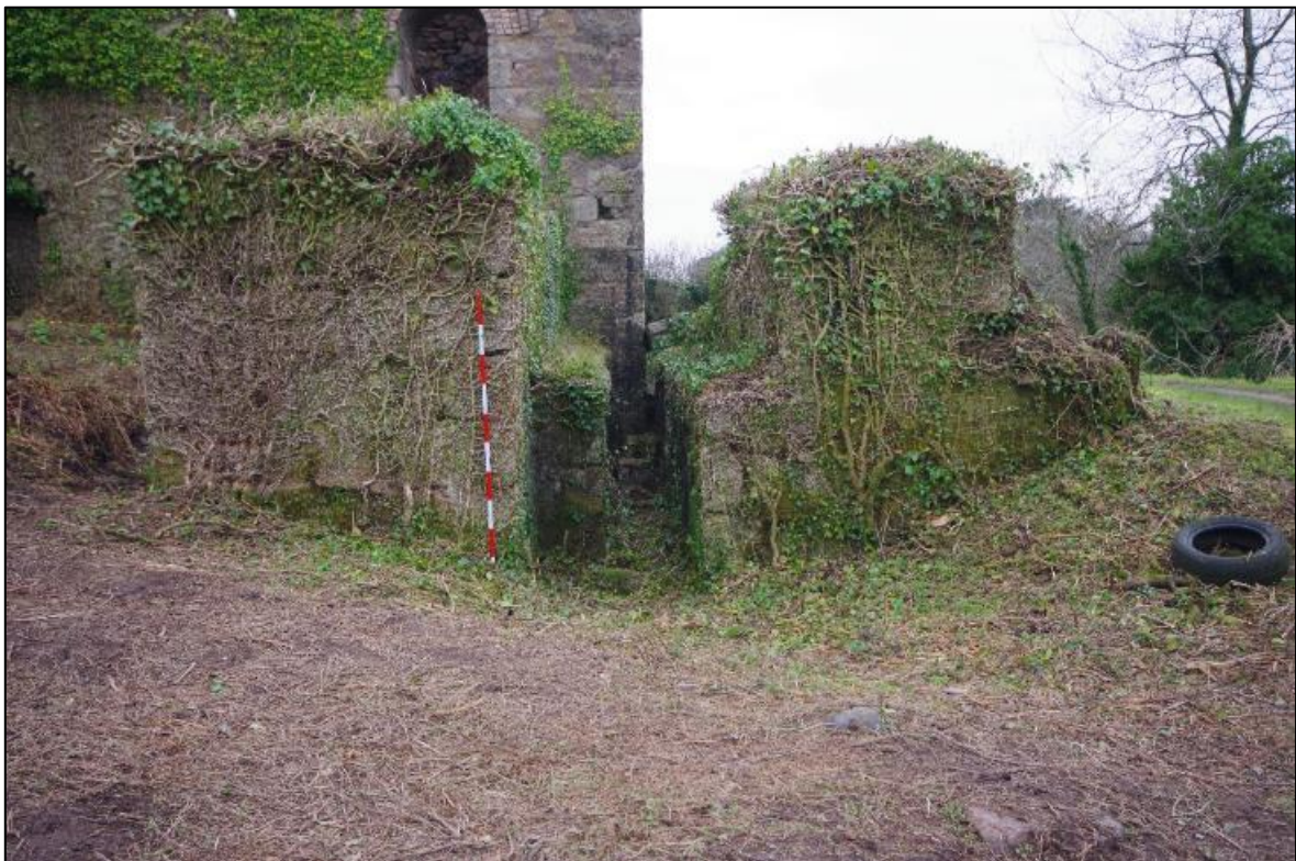
Fig 12 North-east elevation of loadings and flywheel slot before remedial works.
