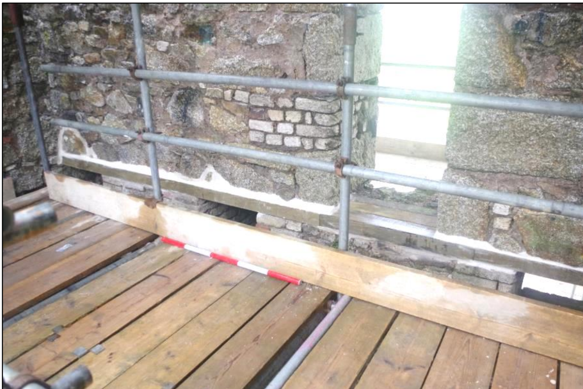
Fig 92 Interior south-east gable wall following replacement of lintel above spring beam slots.
