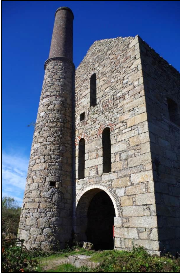
Fig 85 South-east elevation following repairs to cylinder arch, small patch repairs and capping of the top of the gable.
