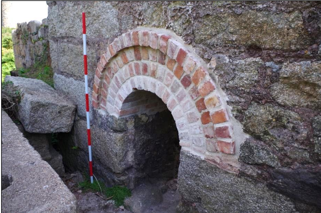
Fig 23 North-west elevation of engine house: arch leading to cataract pit following repair work.
