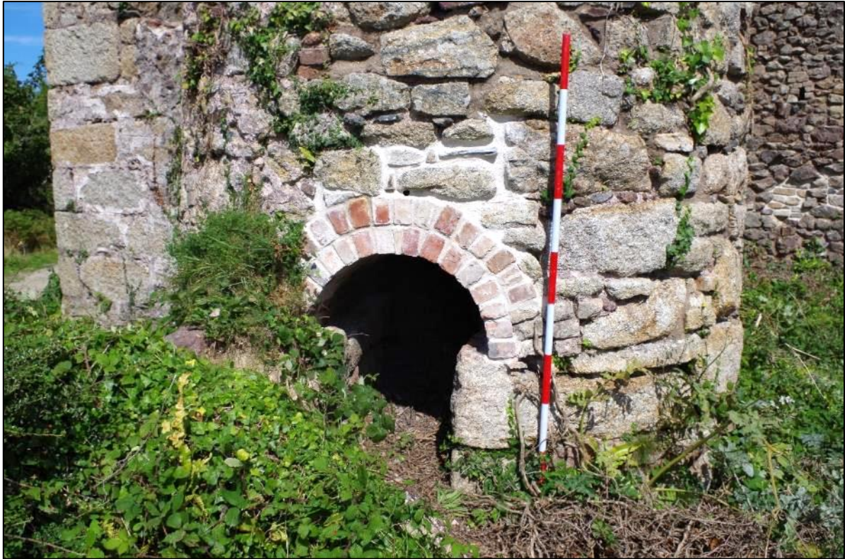
Fig 63 Repairs to the arch of the boiler flue opening at the base of the chimney stack.
