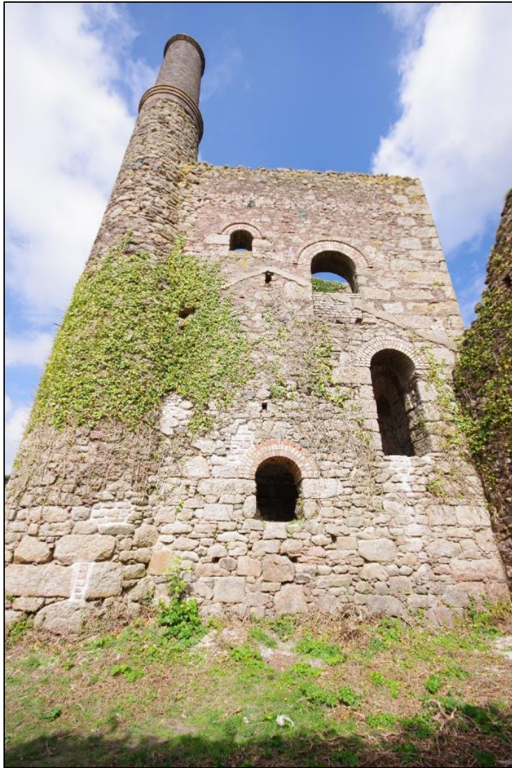
Fig 29 South-east elevation of engine house following patch repairs and some ivy clearance.
