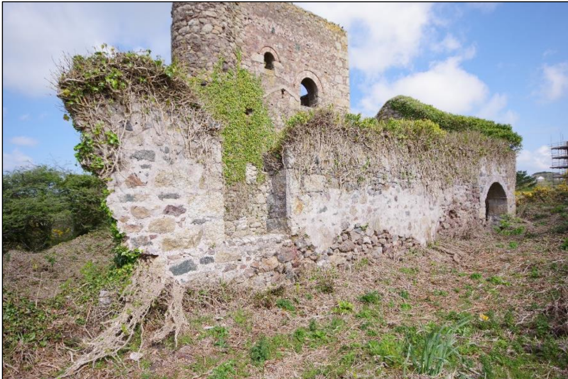
Fig 35 South-east elevation of the boiler house following patch repairs and some ivy clearance.
