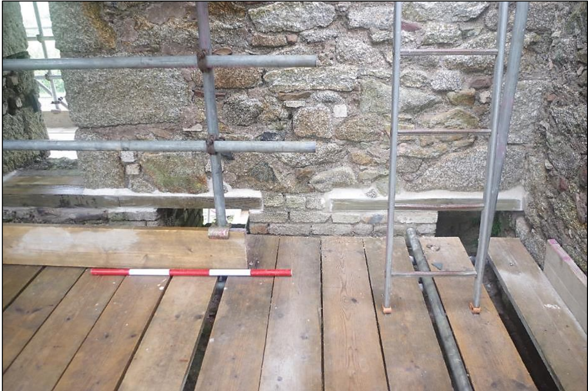
Fig 93 Interior south-east gable wall following replacement of lintel above spring beam slots.
