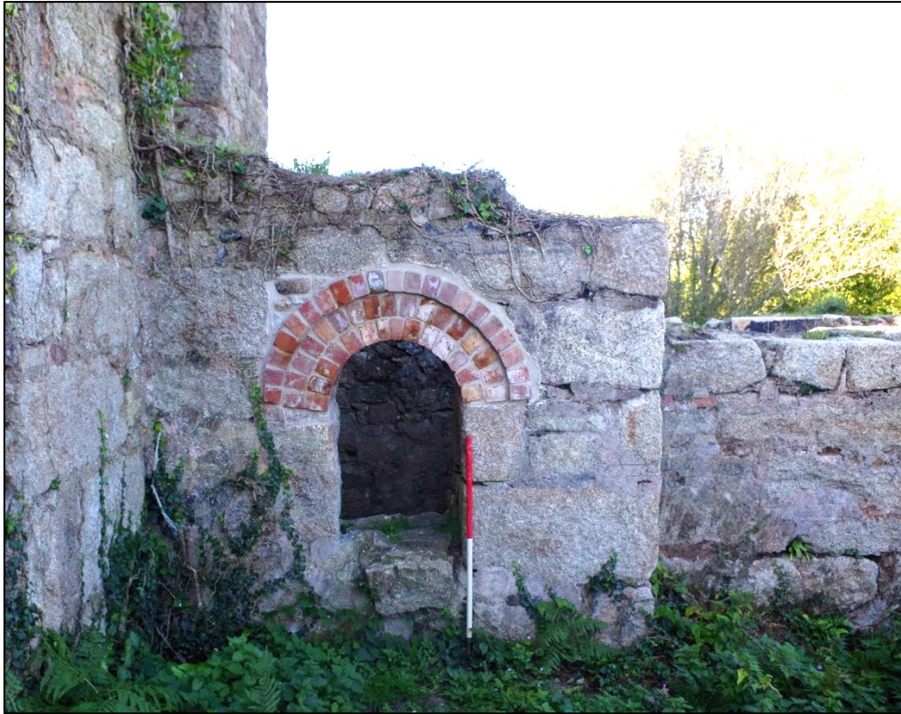
Fig 37 South-east elevation of the loadings: repaired arch of the condenser pit opening.
