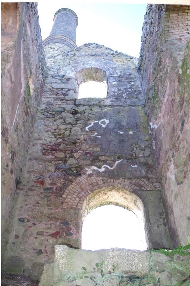
Fig 67 Interior south-west wall of engine house following small patch repairs to incised plaster.
