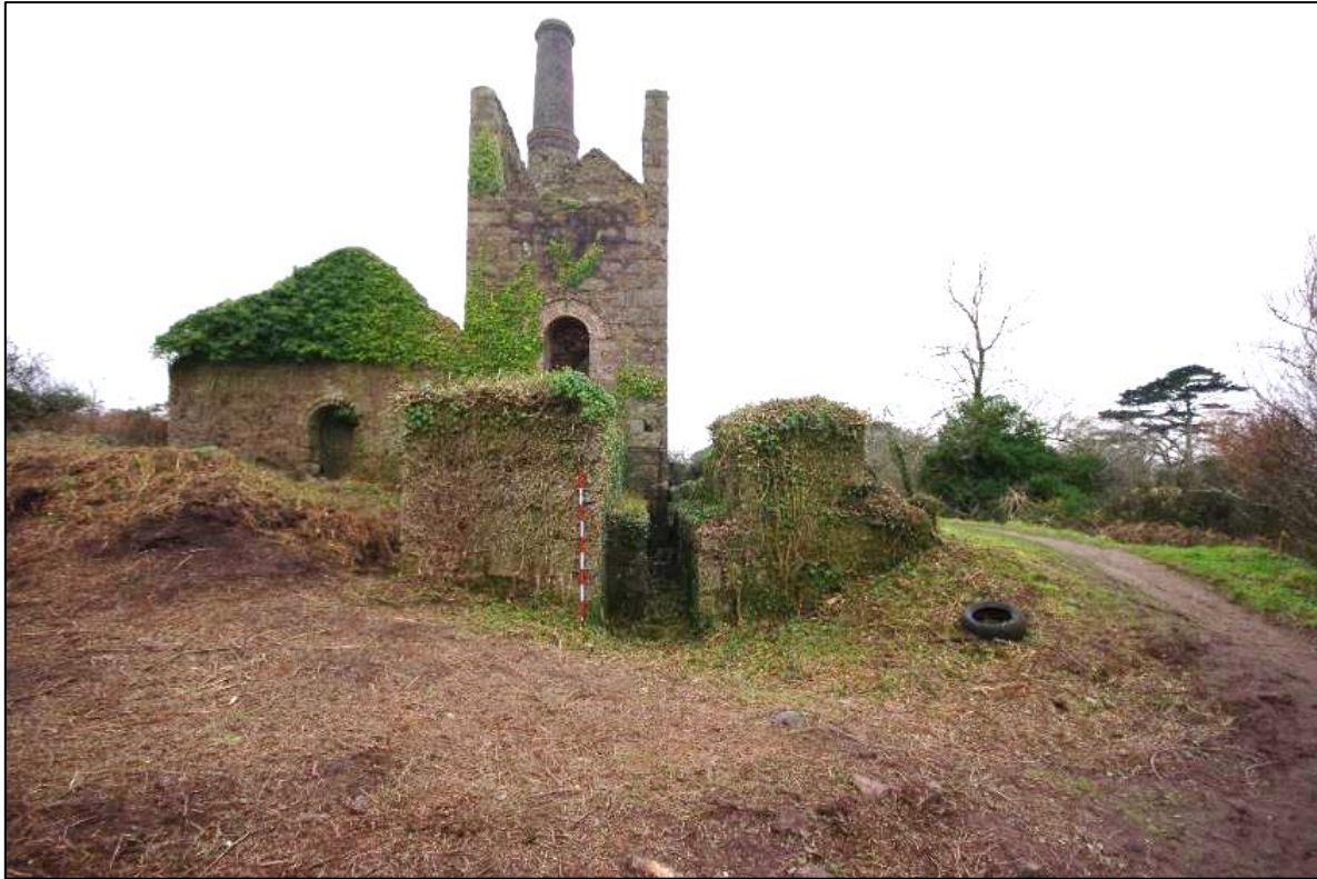
Fig 11 North-east elevation before remedial works.
