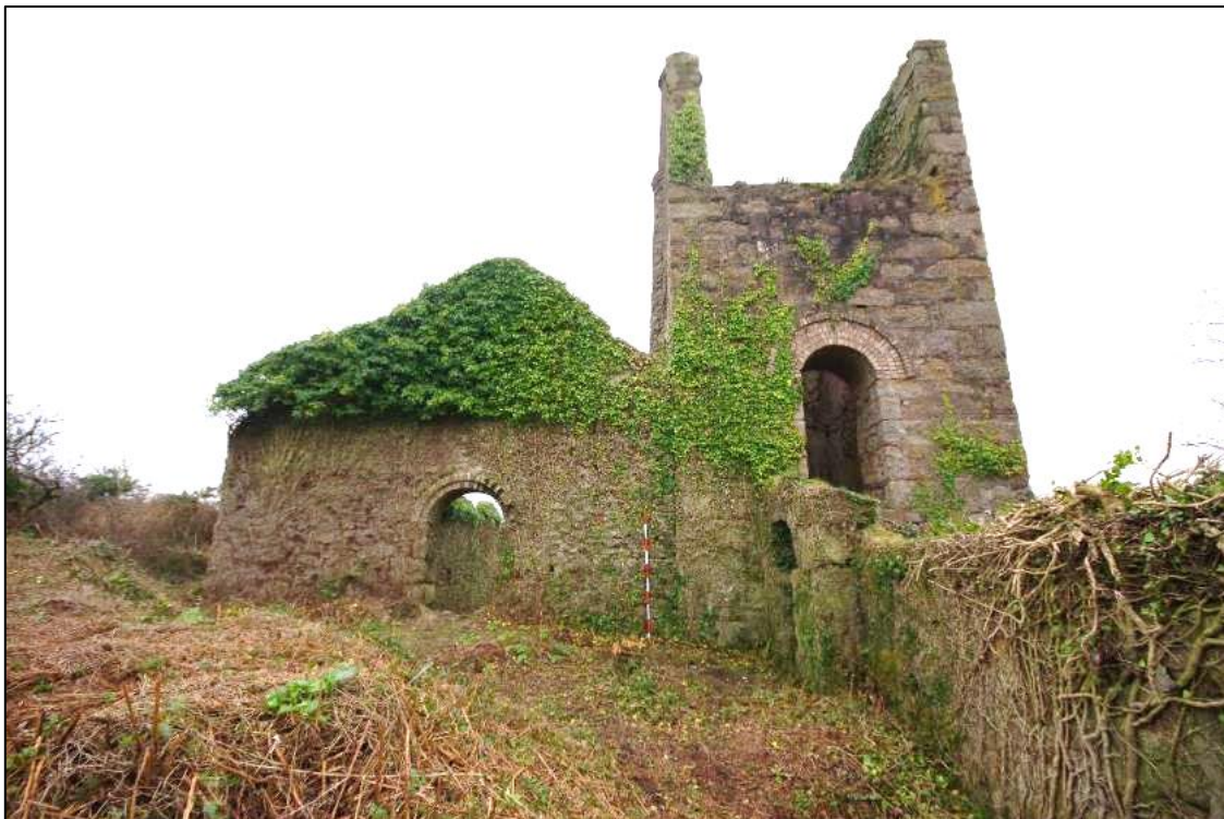
Fig 10 North-east elevation before remedial works.
