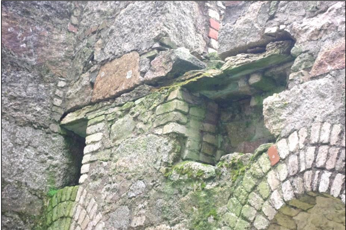
Fig 75 Interior north-east wall jost sockets and lintel before remedial works.
