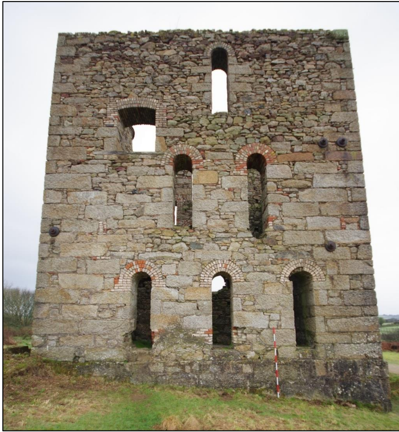
Fig 71 North-east elevation before remedial works.
