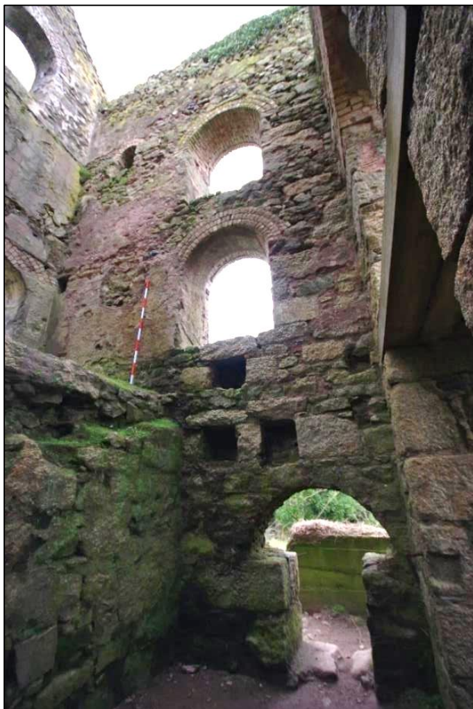
Fig 24 Interior north-west wall before remedial works.
