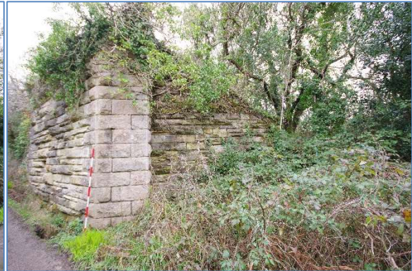
Fig 45 RRB06 Reen Rose Bridge east abutment, south side retaining wall, looking northeast.
