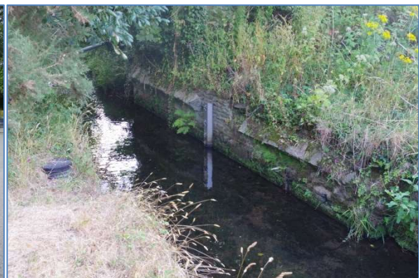
Fig 60 Remains of the 19th century Cocks Hill Bridge on the south side of the river, looking southeast.
