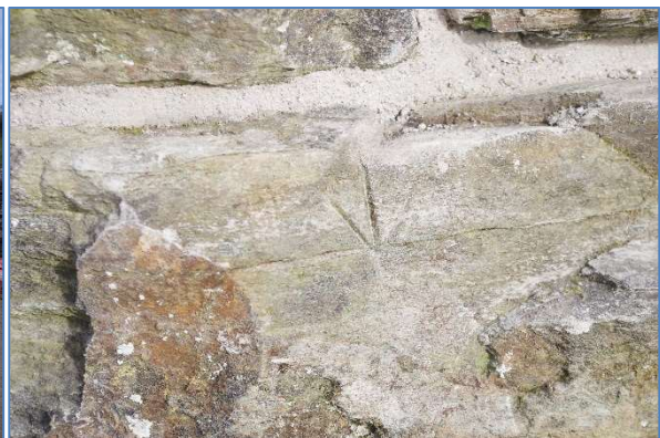
Fig 12 COV14 Benchmark on northern parapet wall of Cocks Viaduct, east end, looking north.
