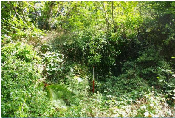
Fig 71 Retaining wall at northeast corner of site, with the sloped ramp beyond, looking northeast towards Bone Mill Road.
