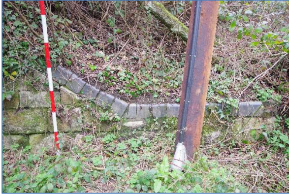
Fig 34 LHB11 Lighthouse Bridge southern abutment, brick coping on west side retaining wall, looking south.
