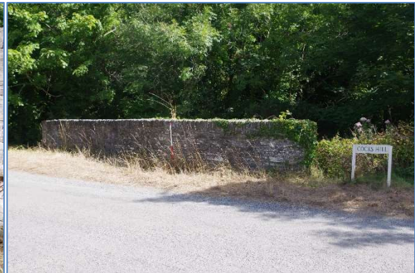
Fig 58 East parapet wall of the current bridge at Cocks Hill, looking east.
