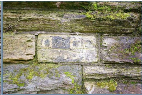
Fig 51 RRB12 Reen Rose Bridge west abutment, south retaining wall, railway sign, looking west.
