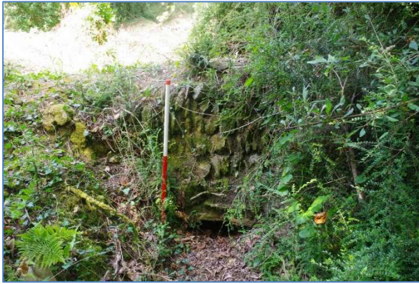
Fig 75 Southeast elevation of the Cornish hedge at the southeast end of the leat showing the stone capped culvert underneath.
