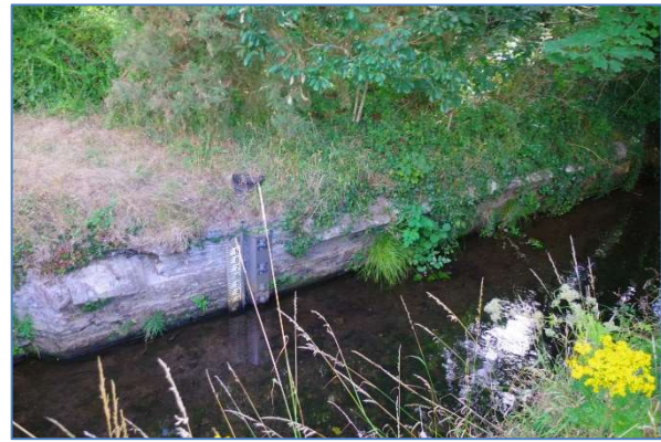
Fig 62 Remains of the 19th century Cocks Hill Bridge on the north side of the river, looking northeast.
