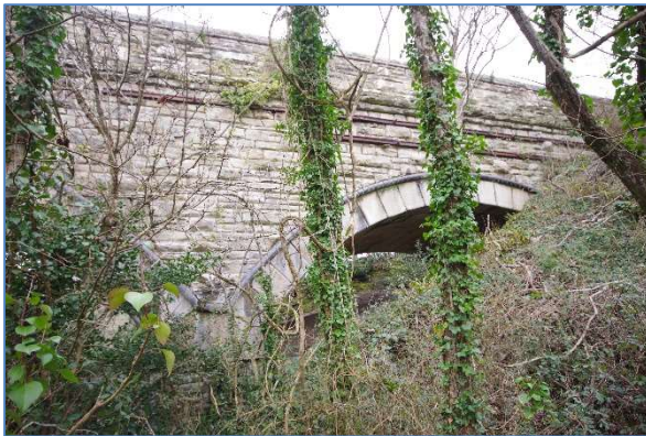
Fig 21 COV48 Cocks Viaduct, south elevation, western and west central arches, looking northwest.
