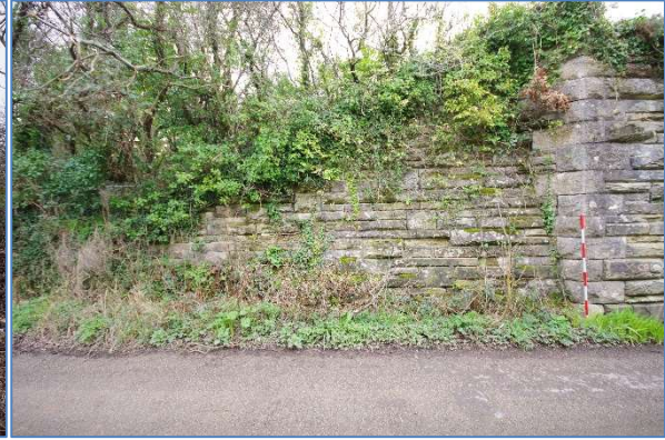
Fig 43 RRB04 Reen Rose Bridge east abutment, north side retaining wall, looking east.
