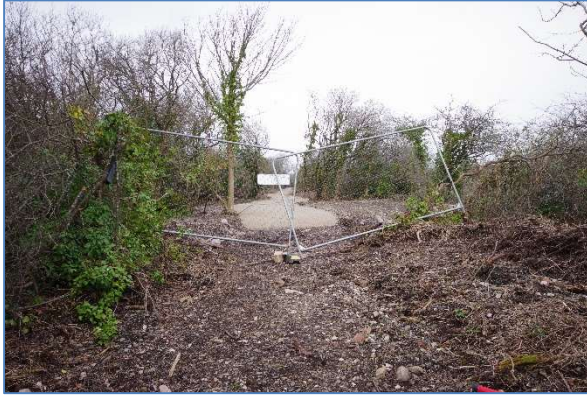
Fig 42 RRB03 Reen Rose Bridge from the top of the eastern abutment, looking east.
