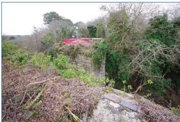
Fig 40 RRB01 Reen Rose Bridge from the top of the eastern abutment, looking west.
