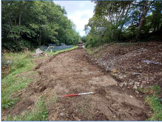
Fig 79 Stripped section along the bank of the flood relief channel at Bolingey Bone Mill, looking northwest.
