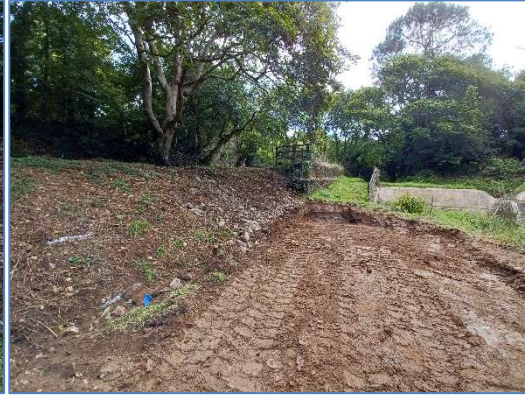
Fig 80 Stripped section in preparation for the trail where it enters the Bolingey Mill site, looking southeast.
