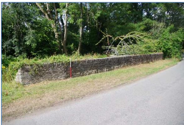
Fig 59 West parapet wall of the current bridge at Cocks Hill, looking northwest.
