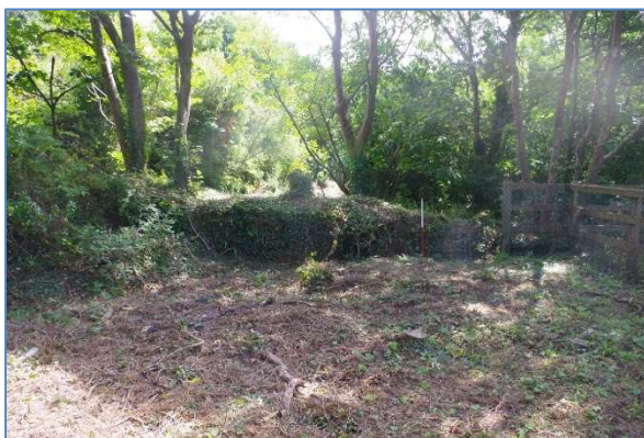
Fig 67 Northwest elevation of the boundary wall overlying the leat (right of shot), looking southeast.
