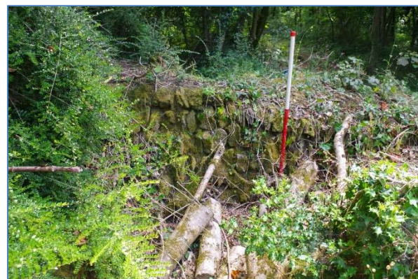
Fig 74 Northwest elevation of the Cornish hedge overlying the southeast end of the leat.
