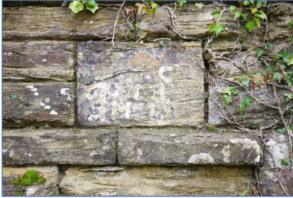
Fig 48 RRB09 Reen Rose Bridge east abutment, north retaining wall railway sign, looking east.
