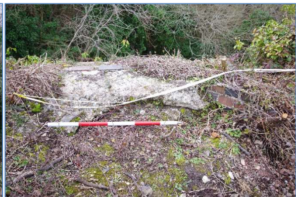
Fig 41 RRB02 Reen Rose Bridge modern consolidation of the top of the eastern abutment, looking northwest.
