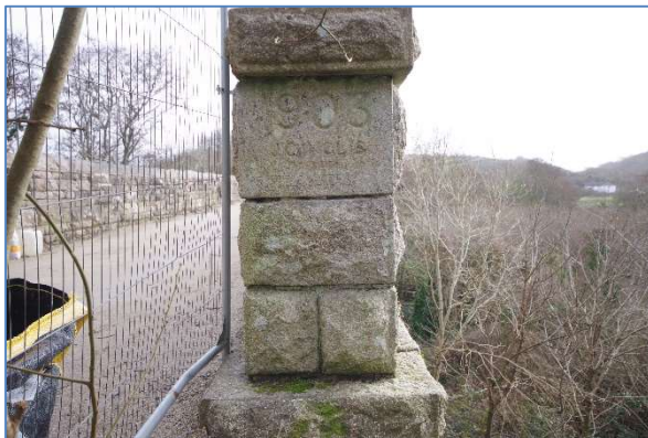
Fig 9 COV08 Inscription on pier at west end of Cocks Viaduct, looking east.
