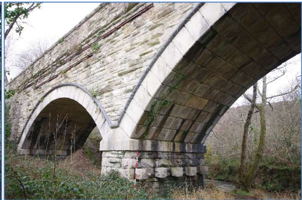
Fig 22 COV50 Cocks Viaduct, south elevation, east central and eastern arches, looking northeast.
