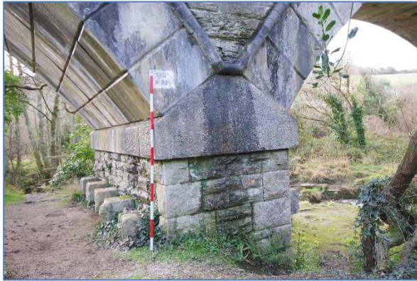
Fig 13 COV32 Pier between the two central arches of Cocks Viaduct, with Railway sign, looking south.
