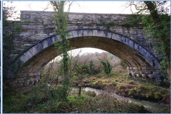
Fig 14 COV34 Western central arch of Cocks Viaduct over the Perran Stream, looking south.
