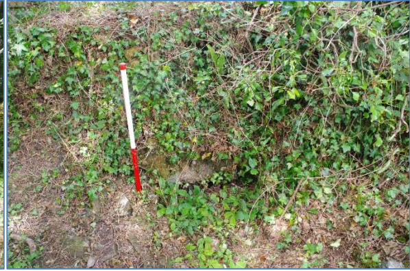
Fig 70 Culvert opening in the base of the overlying boundary wall, looking northwest.
