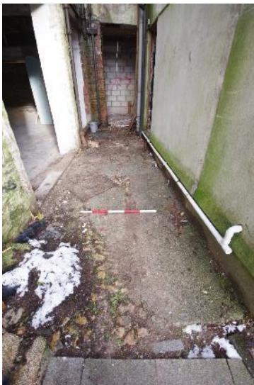
Fig 190 19th century stone sett surface between the Mining Exchange and Wheal Peevor purser's office looking north east.
