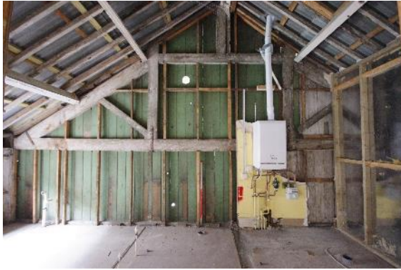
Fig 166 F11, F12 and F13 south west wall during the watching brief with truss exposed.
