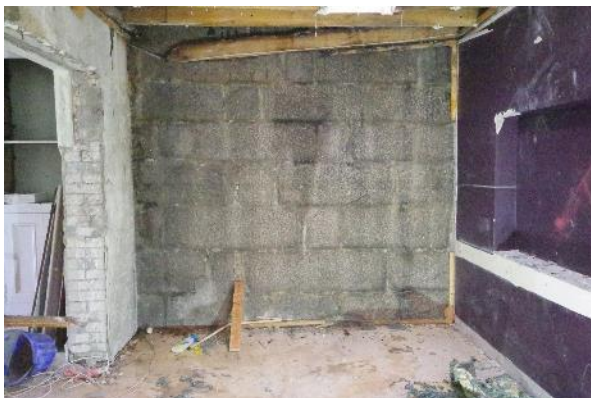
Fig 183 F19 during watching brief, south west wall with 20th century covering removed showing exterior ashlar granite wall of the market house.
