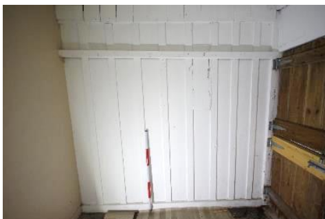
Fig 85 G15 north west wall.
