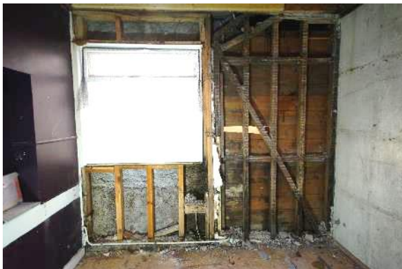
Fig 182 F19 during watching brief, north west wall showing the two phases, the early 20th century extension wall on the right and 1960s wall on the left.
