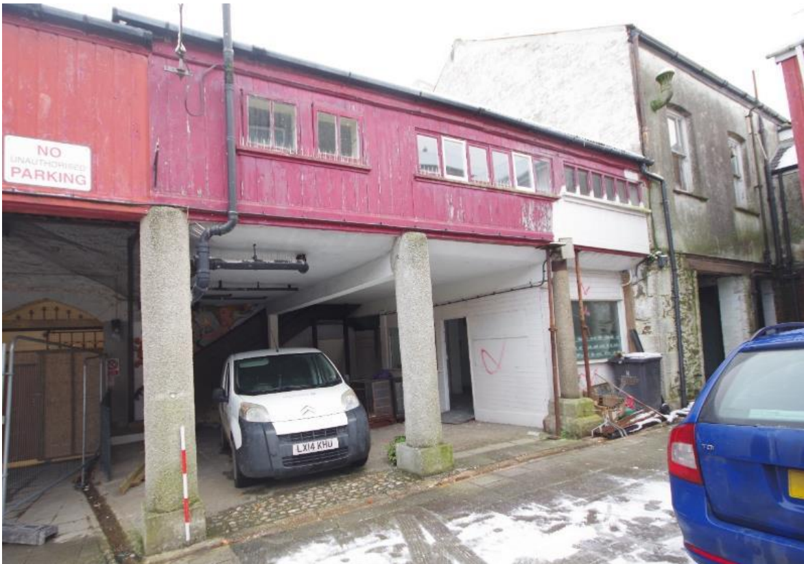
Fig 53 South east elevation of the Mining Exchange extension (left) and Mining Exchange (right).
