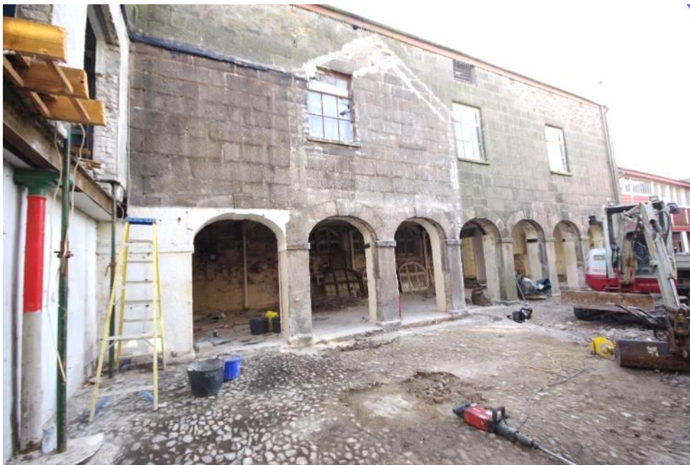
Fig 46 North west elevation of the market house fully exposed during the watching brief.
