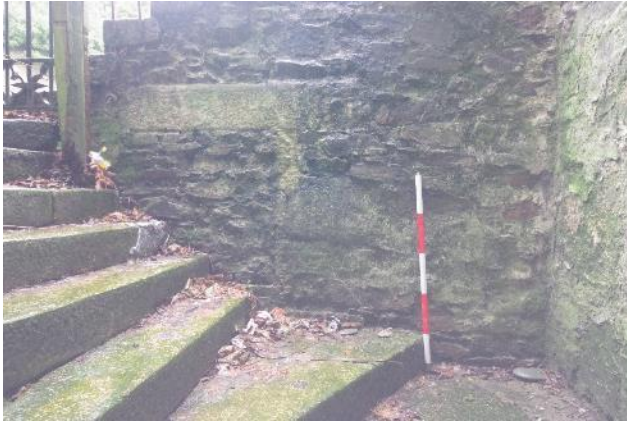
Fig 117 Steps next to purser's office looking south east showing blocked door opening into former room beneath market house steps.
