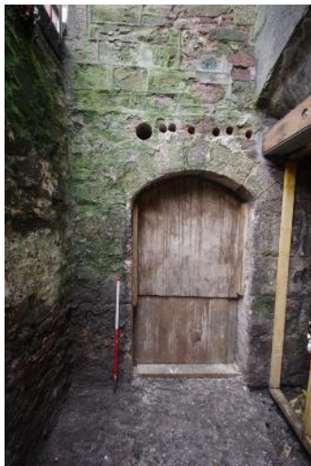
Fig 119 Arched door opening in north east wall of market house taken following removal of steps next to Wheal Peevor purser's office and unblocking.
