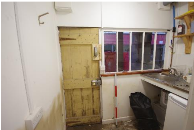
Fig 83 G13 north west wall.
