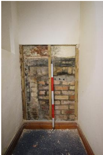
Fig 67 G2 south west wall showing blocked fireplace.
