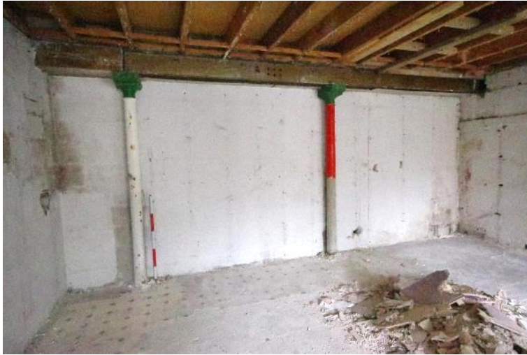
Fig 75 G8 and G9 north east walls during demolition with exposed original supporting columns for Wheal Peevor purser's office.
