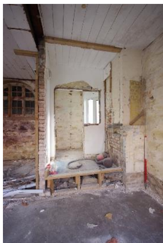
Fig 68 G2, G3 and G4 during watching brief, showing raised floor and chimney breast. Looking south east.
