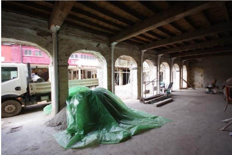
Fig 64 G1 north west wall during watching brief with c1900 windows removed from arcade.
