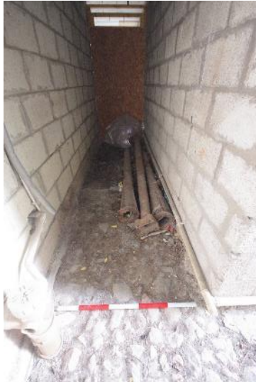
Fig 191 19th century stone sett surface in passage beneath purser's office looking south east.
