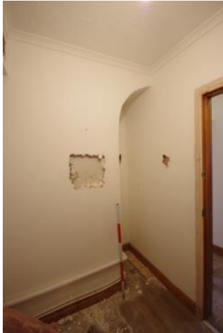
Fig 73 G8 south east wall showing arch.
