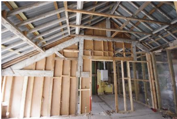
Fig 167 F10 and F14 south west wall during the watching brief with truss exposed.
