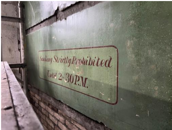
Fig 155 F8 south east wall smoking prohibited sign revealed.
