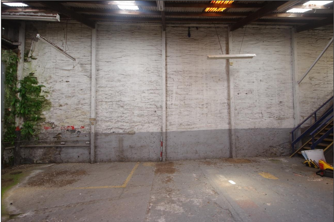
Fig 22 Interior southern part of the east wall of Room 1 (Garage) inside the late 20th century extension.
