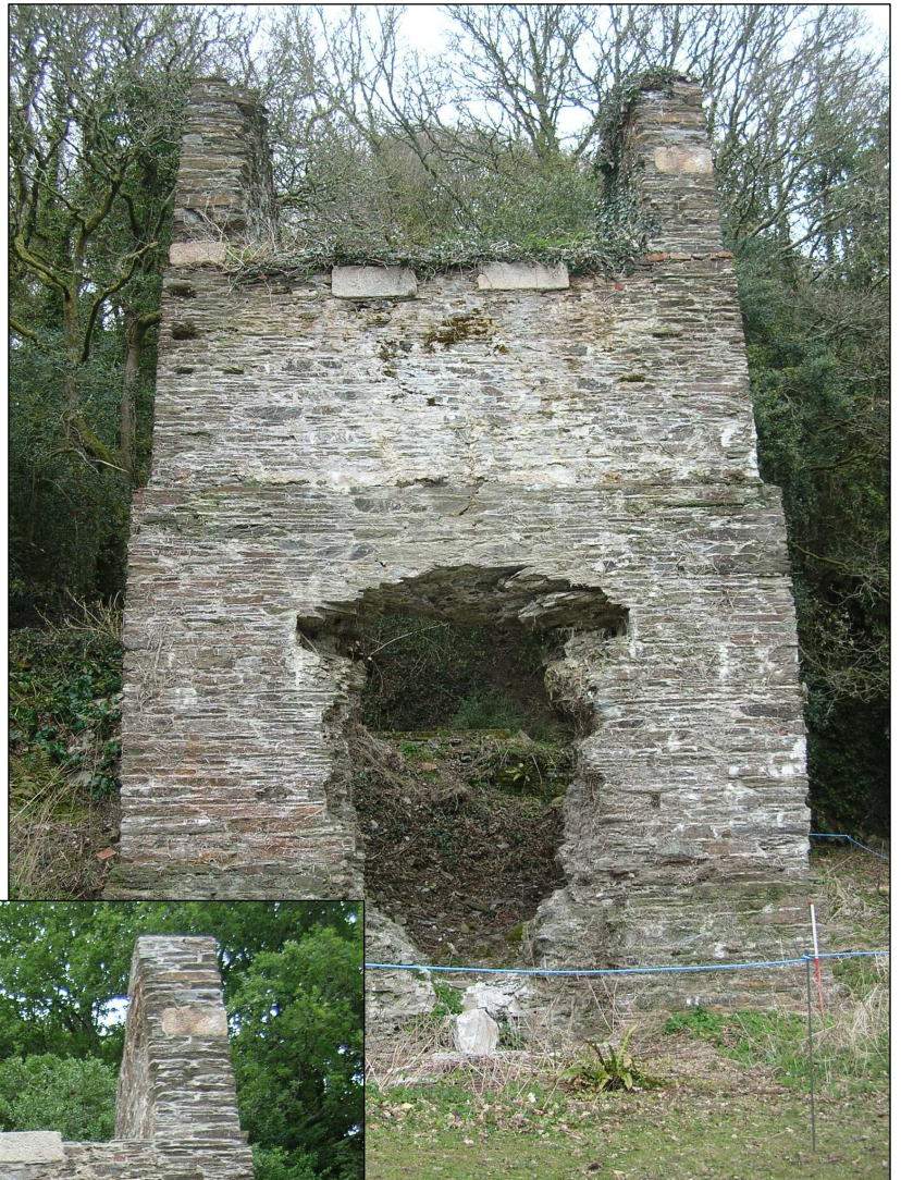
Fig 6 South side view of the Pumping Engine House before works: (Site 1) C. Buck 2010© CC HE
