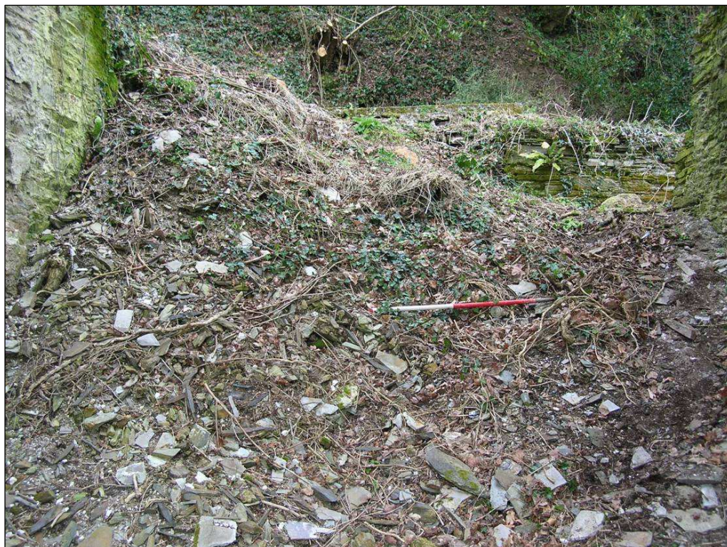
Fig 15 North (internal) view of the Pumping Engine House before works C Buck 2010© CC HE
