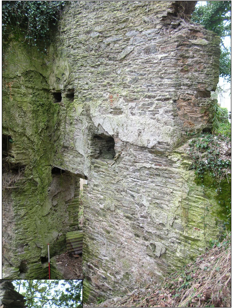
Fig 12 West (internal) view of the Pumping engine house before works (Site 1) C. Buck 2010© CCHE
