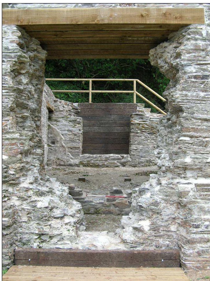
Fig 16 North (internal) view of the Pumping Engine House after works C Buck 2010© CC HE
