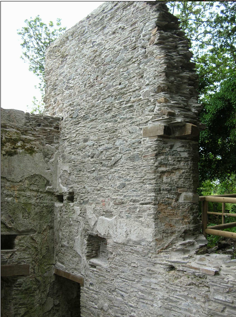
Fig 13 West (internal) view of the Pumping engine house after works (Site 1) C. Buck 2010© CCHE
