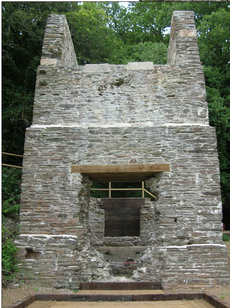
Fig 7 South side view of the pumping Engine House after works: (Site 1) C. Buck 2010© CC HE
