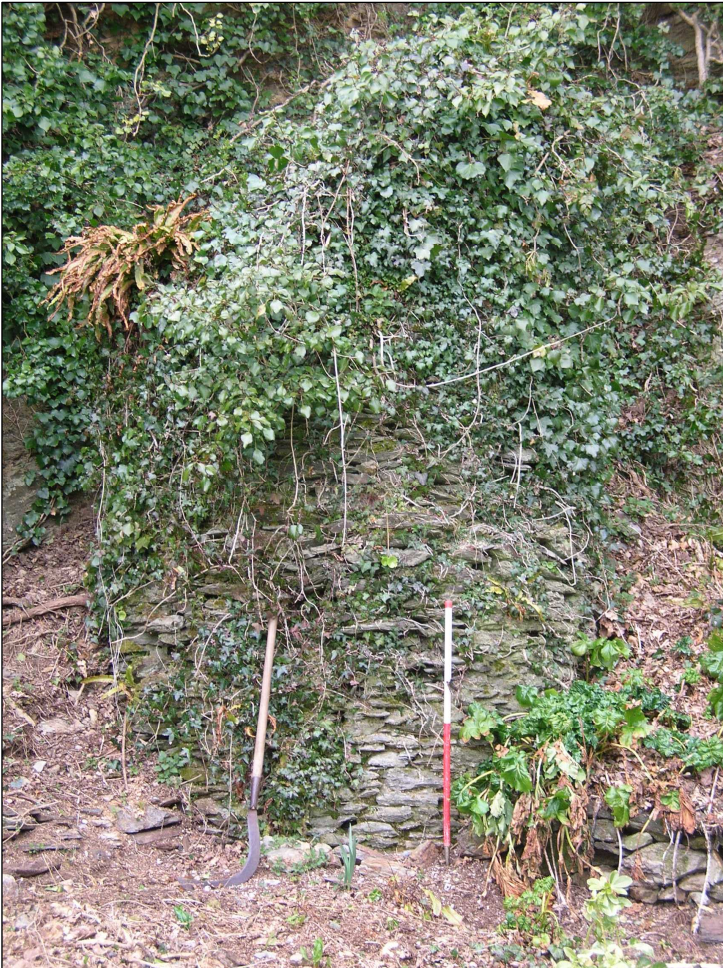
Fig 23 View of the winding engine boiler house chimney before works C Buck 2010© CC HE
