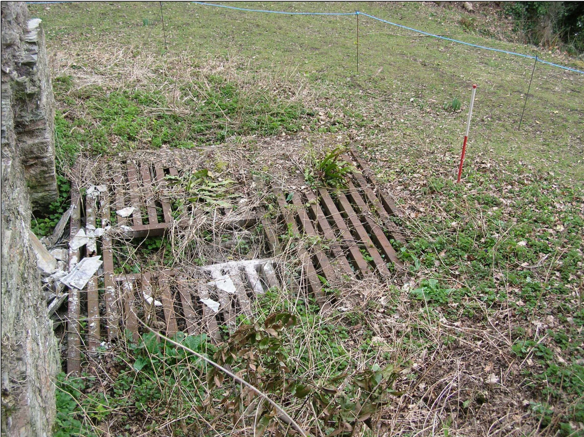
Fig 20 View of the Pumping Engine Shaft before works C Buck 2010© CC HE
