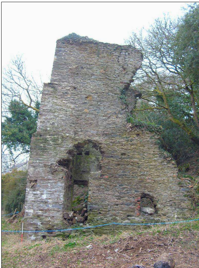
Fig 9 East side view of the Pumping Engine House before works C Buck 2010© CC HE
