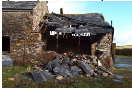
Fig 51 Building 2: front wall, far right
