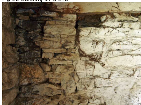
Fig 23 Building 1: S end blocked vent detail
