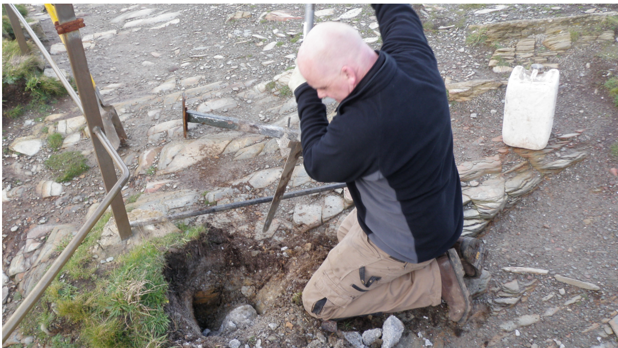
Fig 2: Posthole 2 - breaking out concrete from the existing posthole adjacent to The Tunnel.
