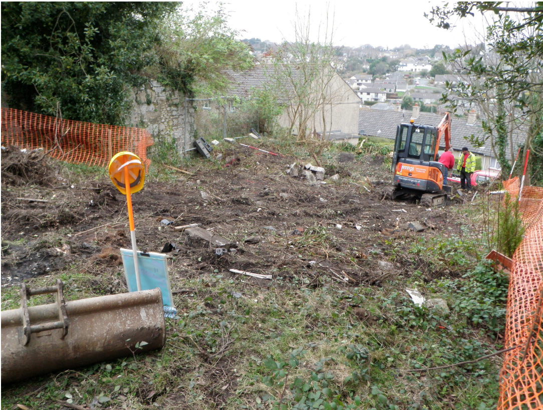
Figure 8 Looking north across the site (2 nd March 2011), showing the site after vegetation clearance, but prior to excavation.
