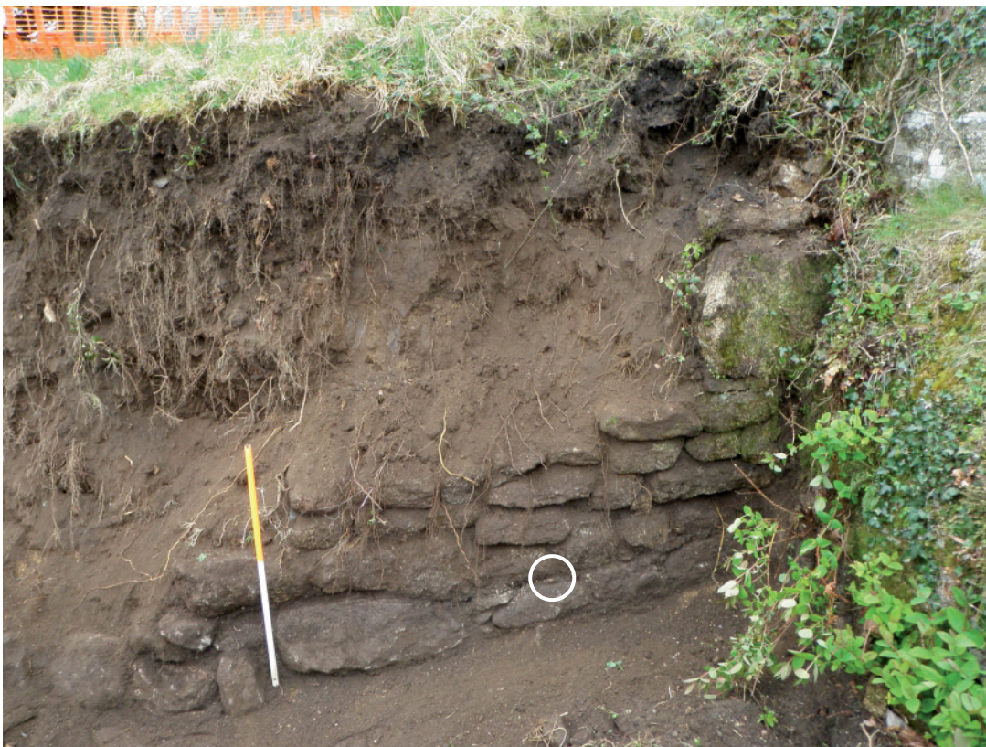
Figure 8 Looking north at the extreme eastern end of the wall - where it joins the Listed church steps. The white circle marks the find spot (between the stone coursing) for two sherds of c19 th century pottery (which dates this part of the wall).
