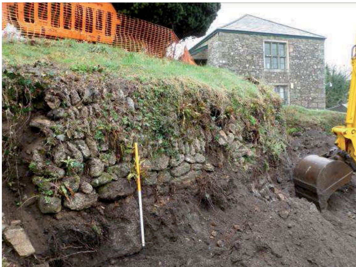
Figure 6 Looking north-east along the churchyard wall prior to dismantling, showing newly revealed basal wall foundations.
