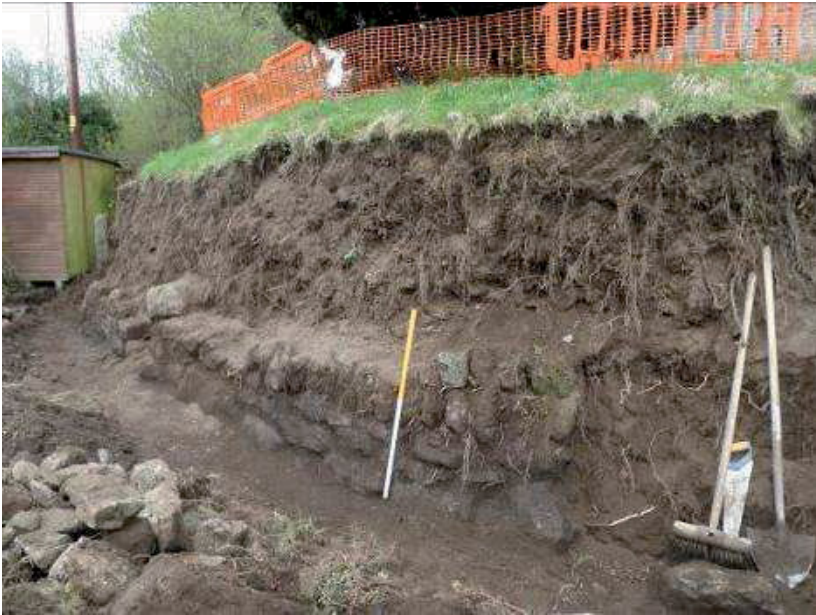
Figure 9 Looking south-west along the exposed basal walling, showing the gap caused by recent collapse and subsequent repair work.
