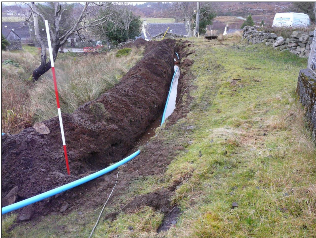
Plate 1 - Photo 27, a section of the trench in Drumbuie below an un-made track, facing E
