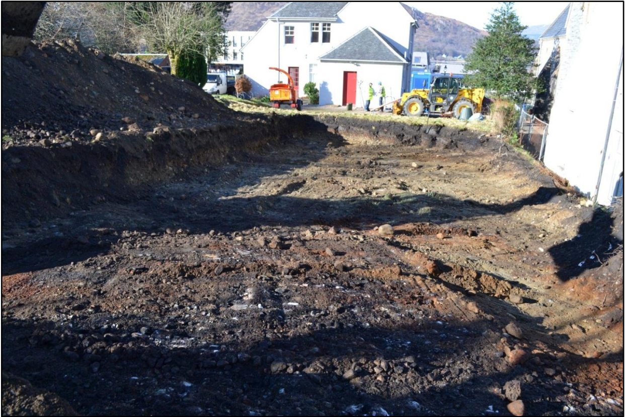
Plate 2: The site post-stripping, facing WNW. It shows the ground sloping towards the Manse
